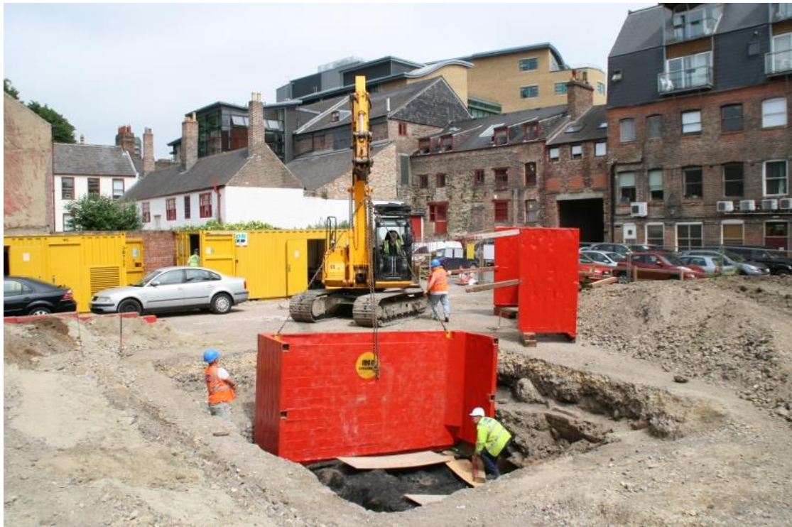
Plate 9. Trench 1, during shoring installation, working shot; rear of Broad Chare, including Live Theatre, in rearground; looking north
