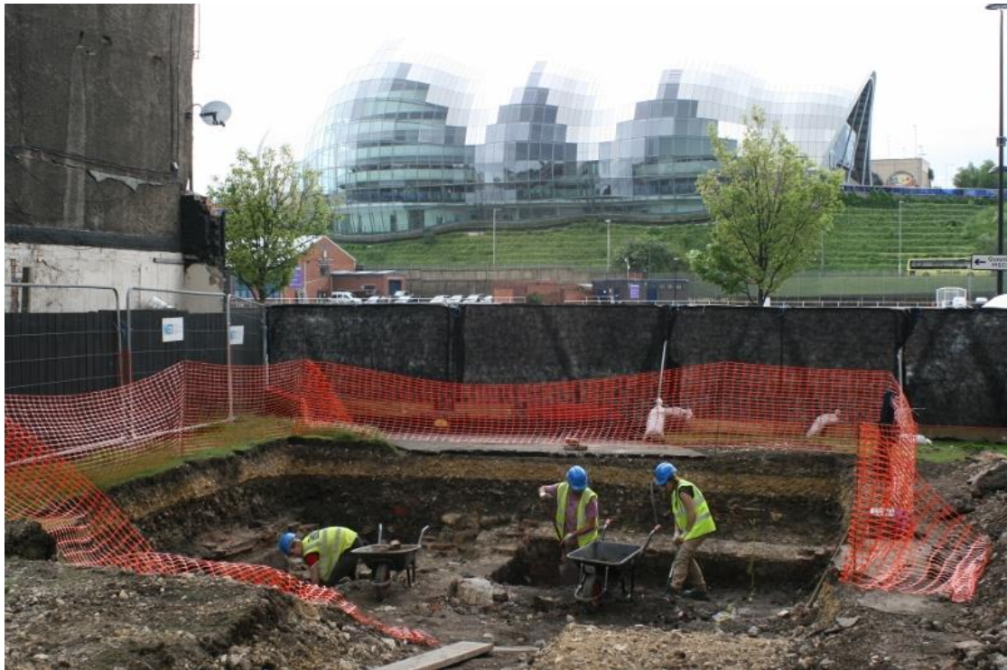
Plate 7. Trench 2, prior to shoring installation, working shot; Sage Gateshead in rearground; looking south-east
