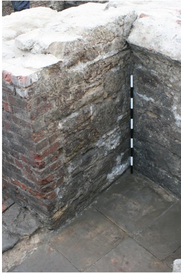
Plate 29. Trench 2, Phase 3 structures: walls [32] and [33] (with brick facing [38]) at junction with wall [34] (right); looking south-east (1m scale)
