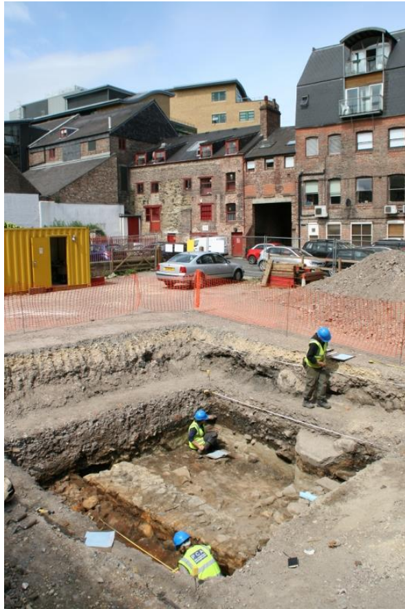
Plate 5. Trench 1, prior to shoring installation; rear of Broad Chare frontage, including Live Theatre, in rearground; looking north
