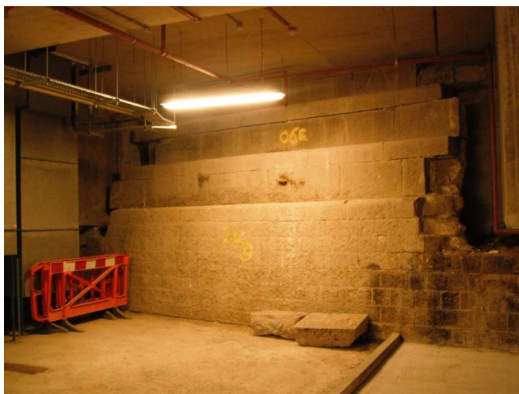
Plate 13: View of retained structure to 1876-1878 graving dock, beneath Reuters Data Centre, south of the site
