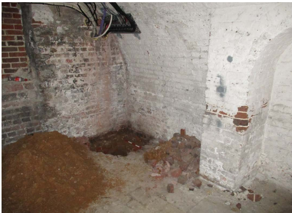
Plate 2: View southwest of Test Pit 7. The work confirmed that the basement had truncated the site beyond the original level of the natural river terrace gravels.
