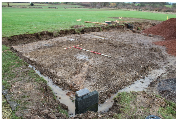
Plate 3. General shot of level reduction inside footprint of foundation trenches for garage, looking east. Scales 1 x 2m; 1 x 1m.
