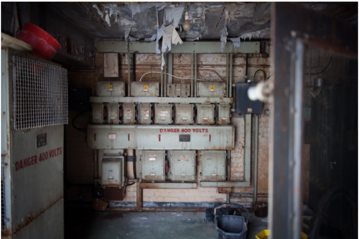
Plate 34 Electricity switch room 2.04 (former valve rectifiers and resistors room), looking north
