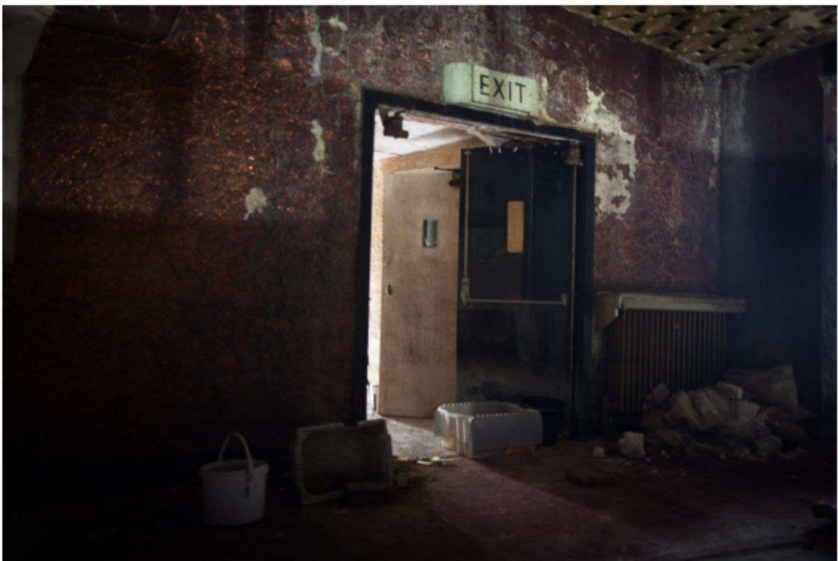
Plate 31 Exit from upper tier of circle 2.01 to stairwell 2.08 and electricity switch room 2.04, looking south-west
