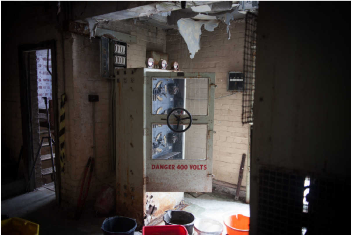
Plate 35 Electricity switch room 2.04 (former valve rectifiers and resistors room), looking south-east
