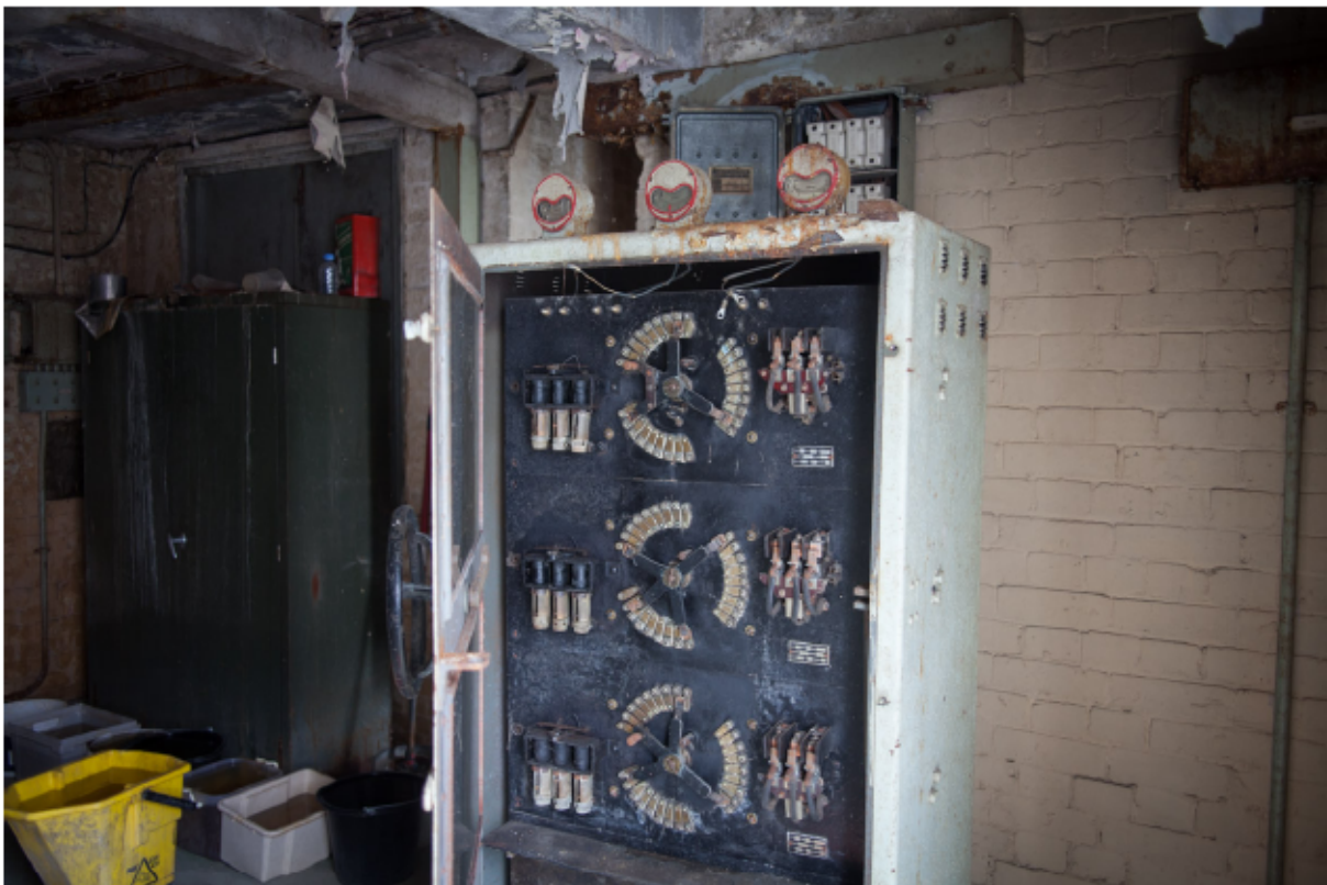
Plate 36 Electricity switch room 2.04 (former valve rectifiers and resistors room), looking north-east
