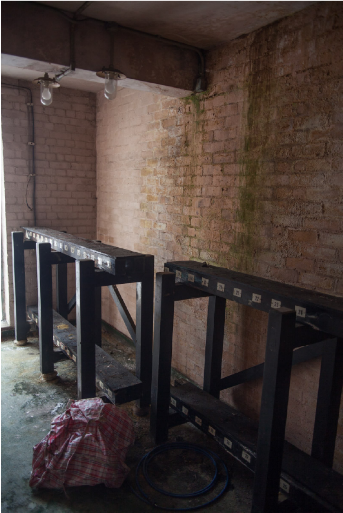
Plate 37 Secondary battery room 2.05, looking south-west
