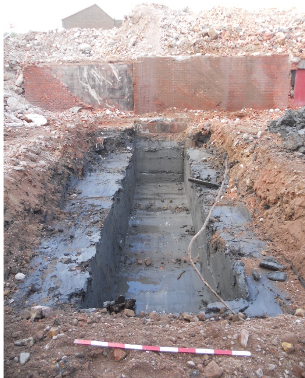
Plate 4: General view of Trench 1 looking north. South wall of Kingfisher Court in background.
