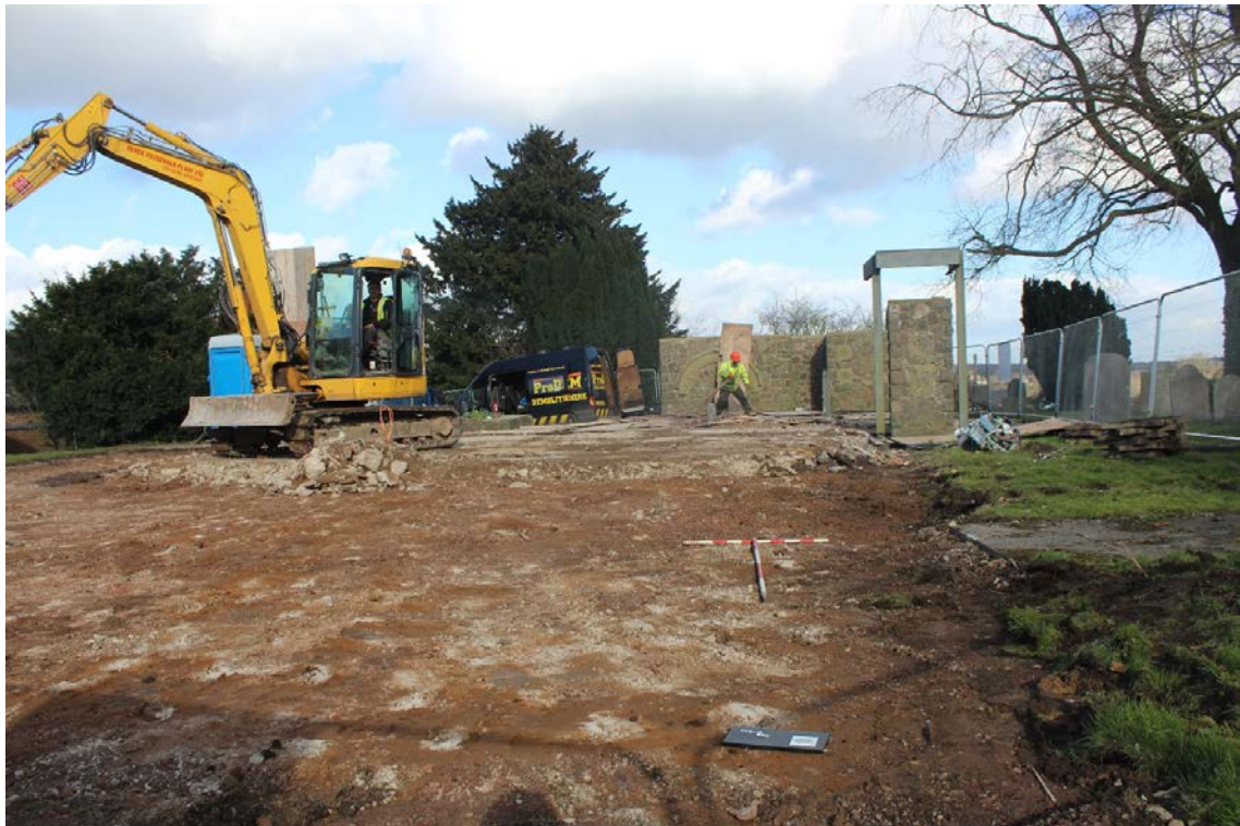
Plate 6: Additional working shot of demolition with the elements of the church left in situ visible. From E; contexts 101 , 103 and 105 are visible.
