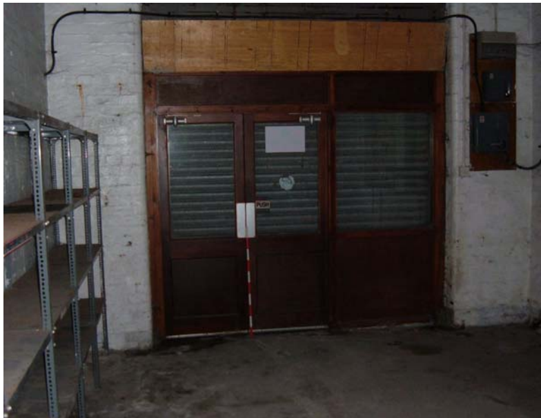
Plate 9. Former Rocket House, interior, south wall/main doorway, from the north (1m scale).
