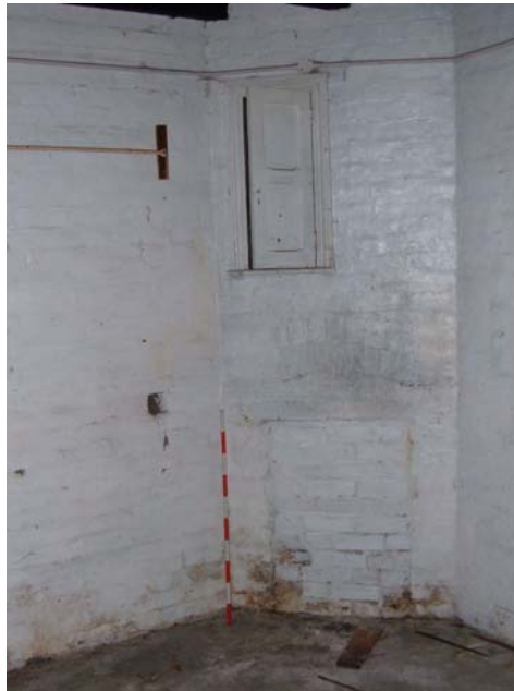
Plate 12. Former Rocket House, interior, angle of north and west walls, from the south-east (1m scale).
