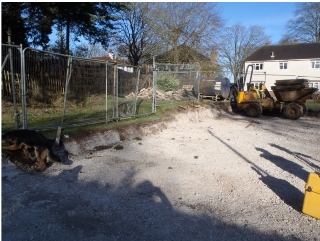
Plate 3: D8, view to East, rear of site stripped to natural chalk. 1m scale.
