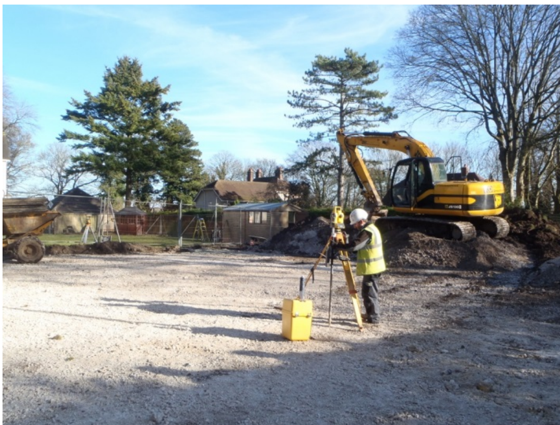
Plate 5: D10, view to East, extent of stripping, rear of site. 1m scale.
