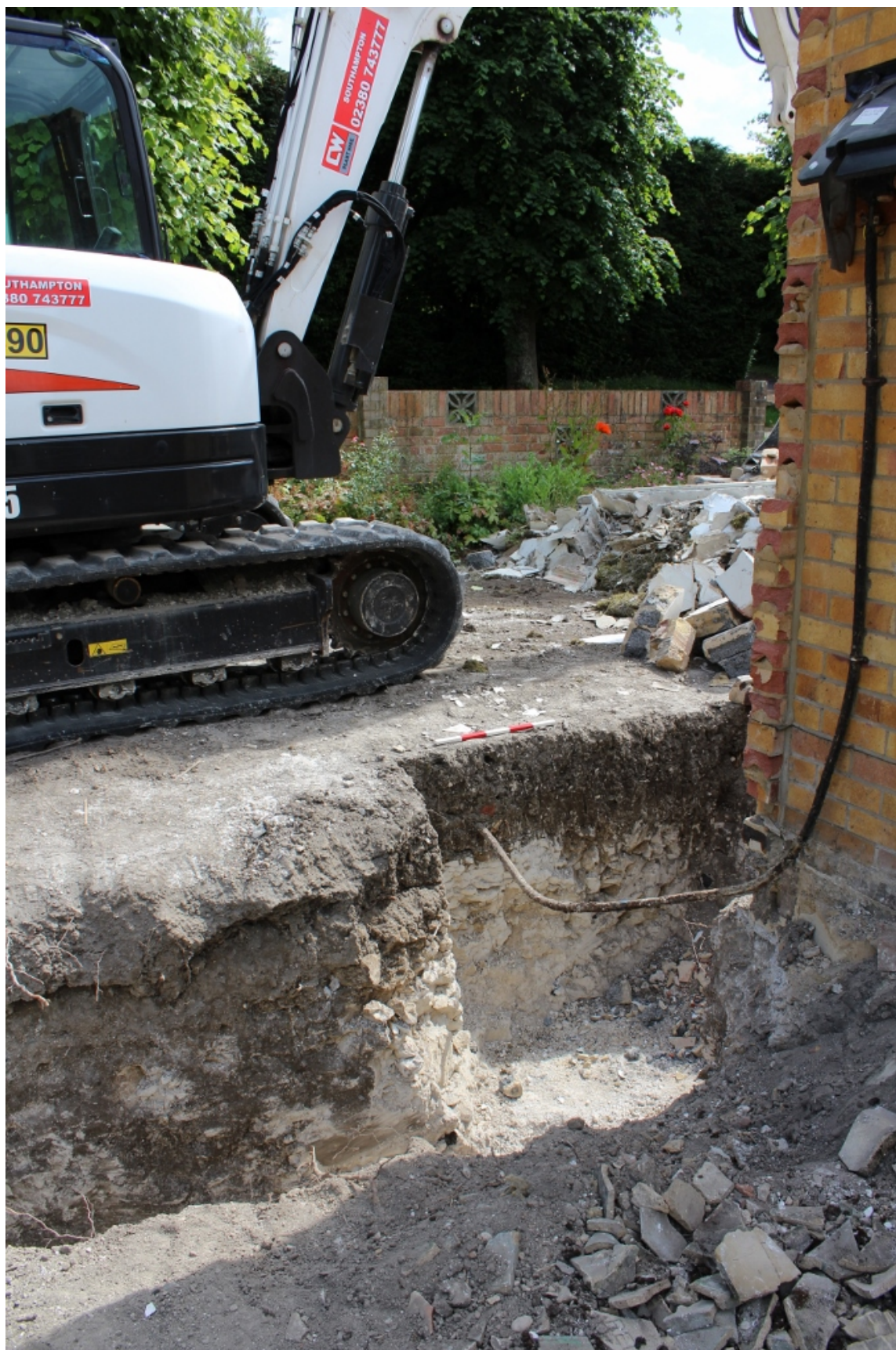
Plate 4: D3 View to south-west of new foundation trench abutting south wall of existing house. Scale 0.5m.
