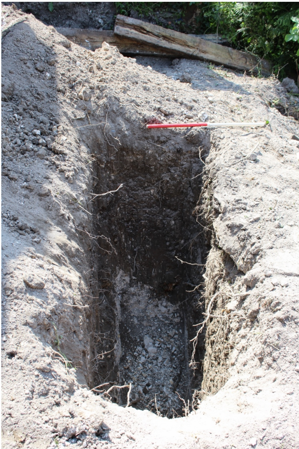
Plate 5: D1 View west of new foundation trench showing natural chalk at c. 1.5m depth below garden soil. Scale 1m.
