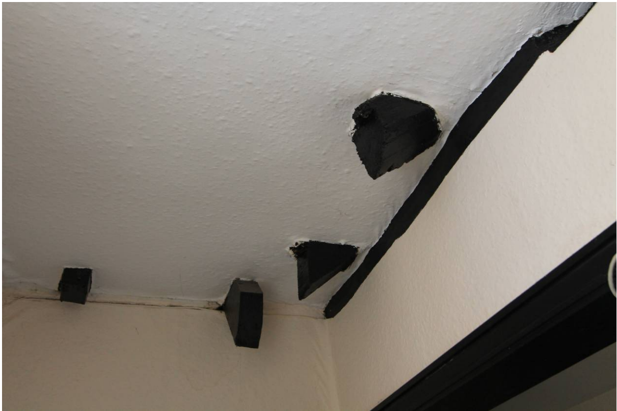
Plate 29 Cut off rafters in (FF6)
