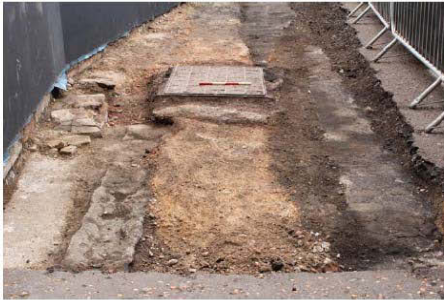
Plate 7: Concrete bedding for road [12], kerb [13], York Stone paving slabs [10] and bedding concrete [11], looking west, 0.4m scale
