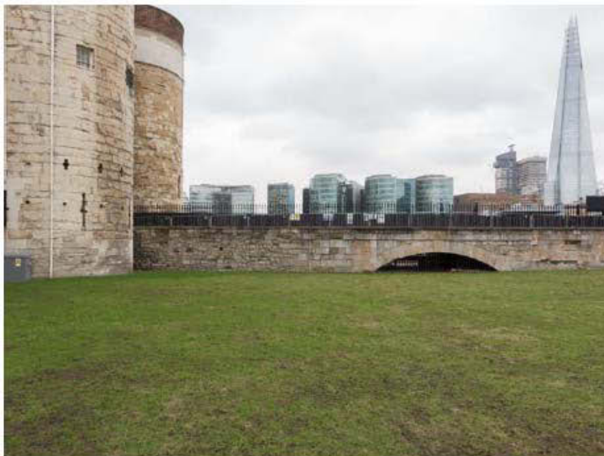
Plate 6: Central Arch of the Causeway with the Byward Tower looking south from within the moat, 2m scale.
