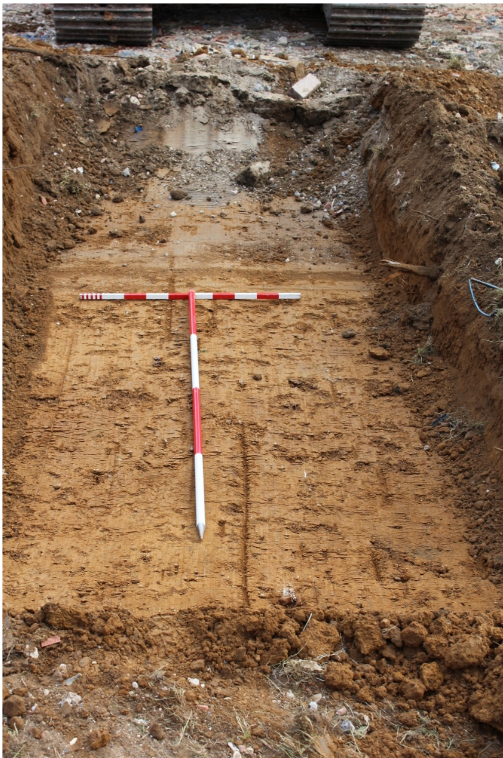
Plate 1: Clean Brickearth exposed in footprint of proposed new house. View to south-east.
