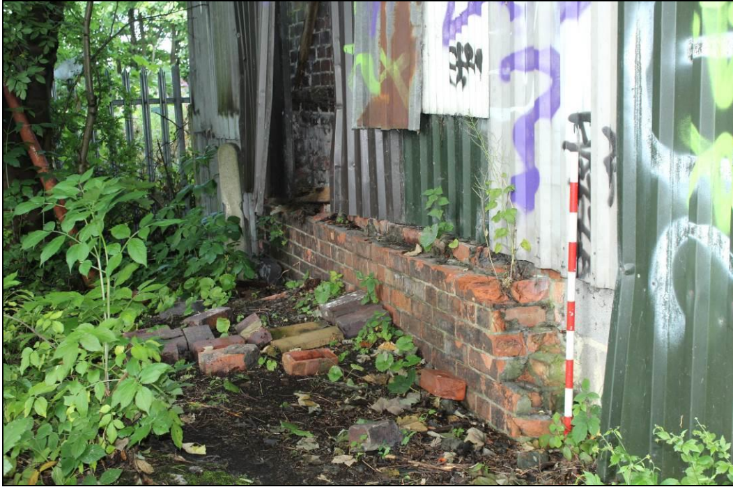
Plate 7. Detailed oblique view of original wall of Albert Hill signal box wall, external elevation, looking south-west (1m scale)
