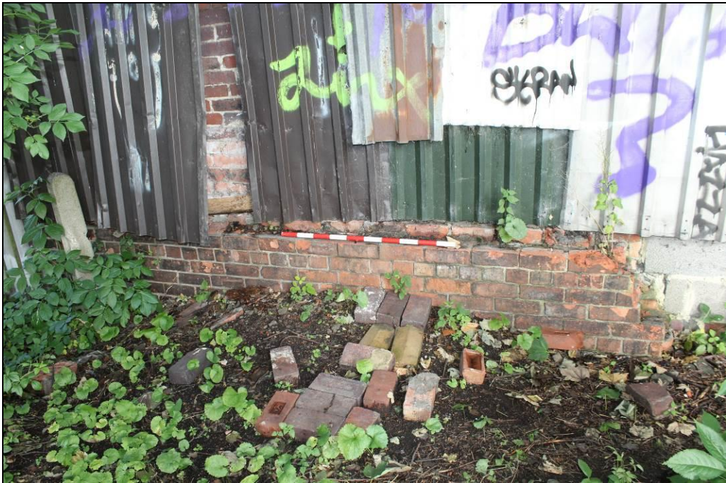
Plate 10. Detailed view of original wall of Albert Hill signal box wall, external elevation, looking west (1m scale)
