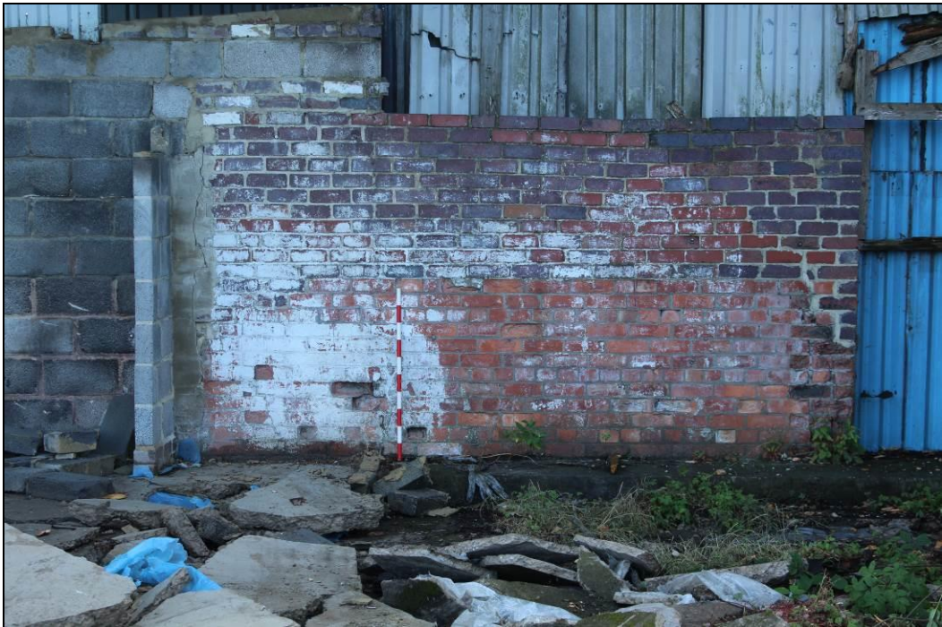
Plate 6. Detailed view of original wall (lower courses) of Albert Hill signal box, internal view (1m scale)
