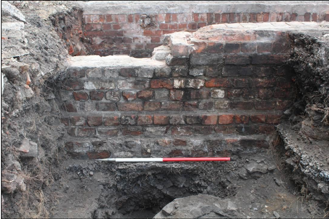
Plate 13. View of north-east facing elevation of wall [212] with concrete foundations [211], looking south-west (1m scale)
