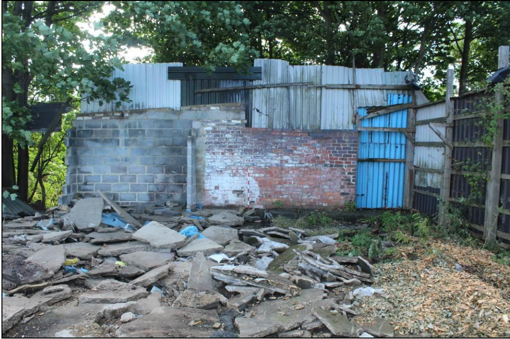
Plate 5. General view of later additions to signal box wall, looking south-east (1m scale)
