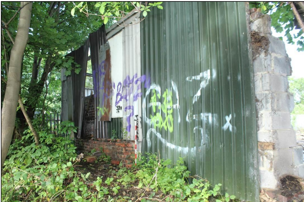
Plate 8. Oblique view of original wall of Albert Hill signal box wall, external elevation, looking south-west (1m scale)
