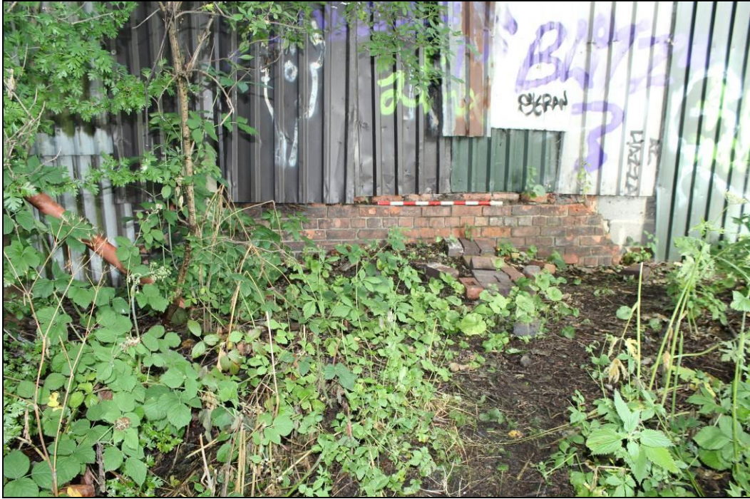
Plate 9. General view of original wall of Albert Hill signal box wall, external elevation, looking north-west (1m scale)
