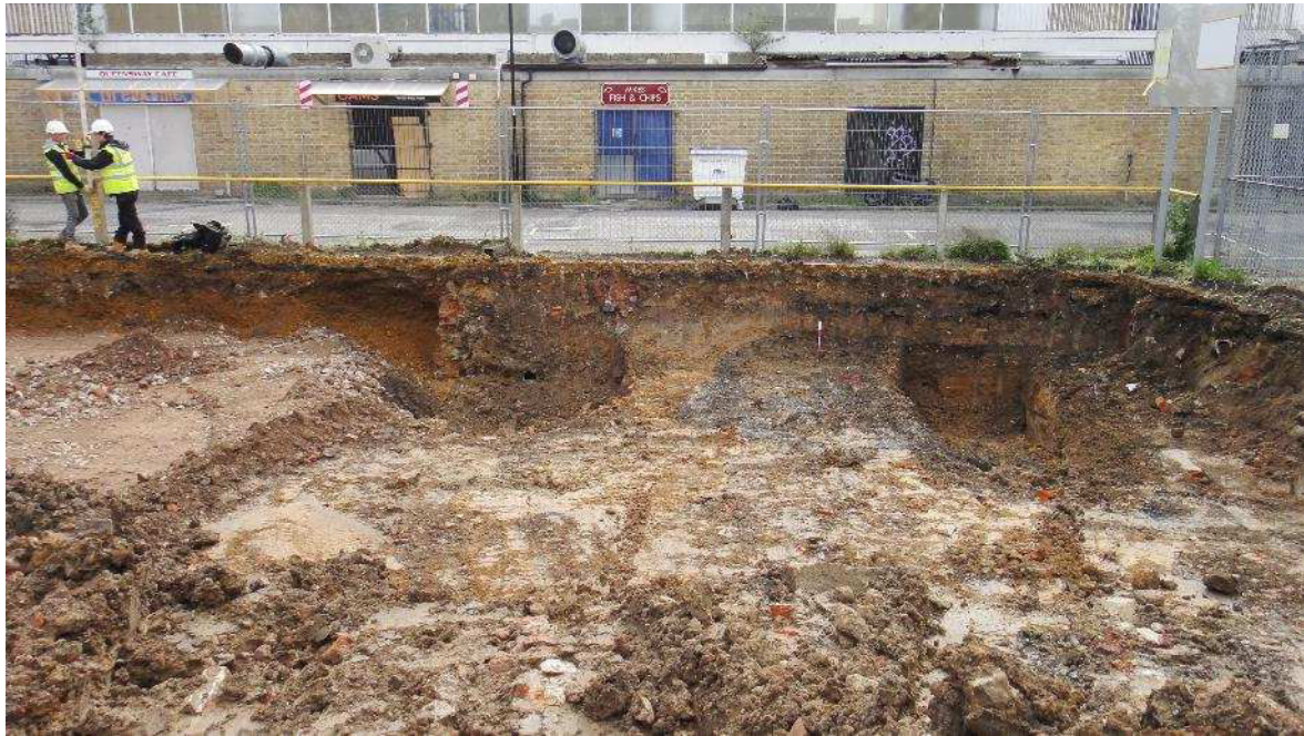
Plate 17. General shot of the area of the Site to west of Trench 7 and north of the Electricity Sub-Station showing strong brown gravel infilling in the section and extensive cuts in redeposited brickearth infilling of the canal in the base of the trench. Scales 2 x 0.4m.
