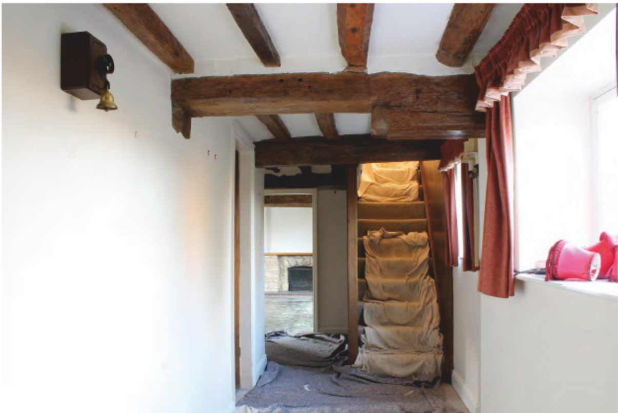
Plate 19 Farmhouse, ground floor looking west, showing cut away beam for head clearance.
