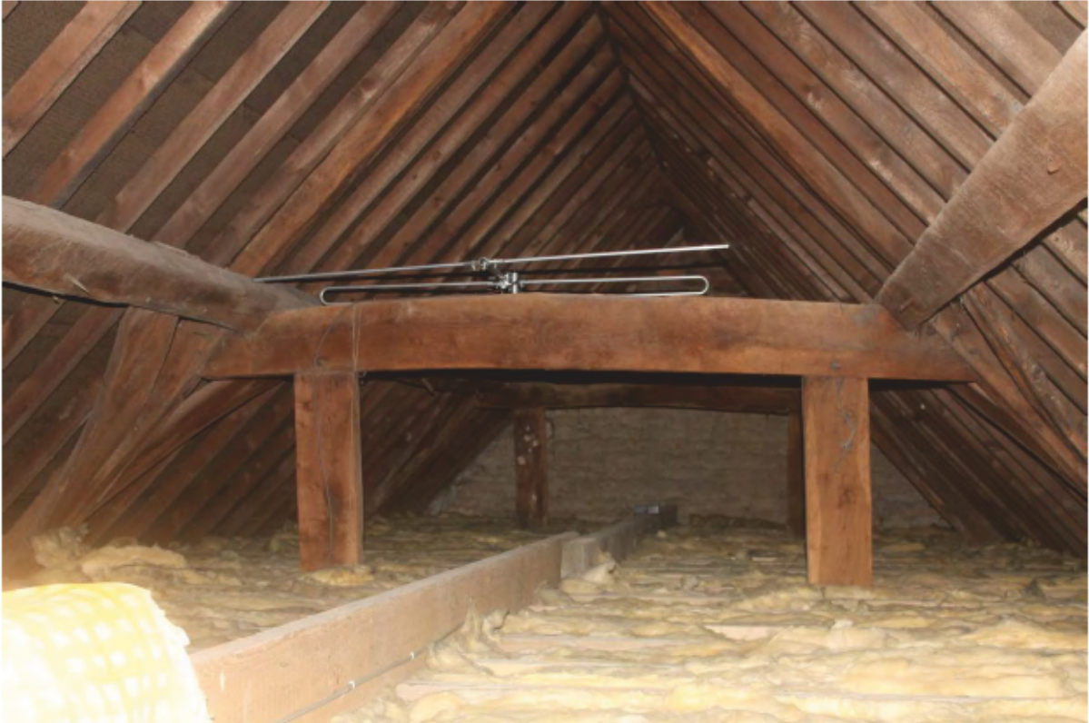
Plate 26 Western roof (bays 1-3) showing curved wind bracing and queen post roof, looking west
