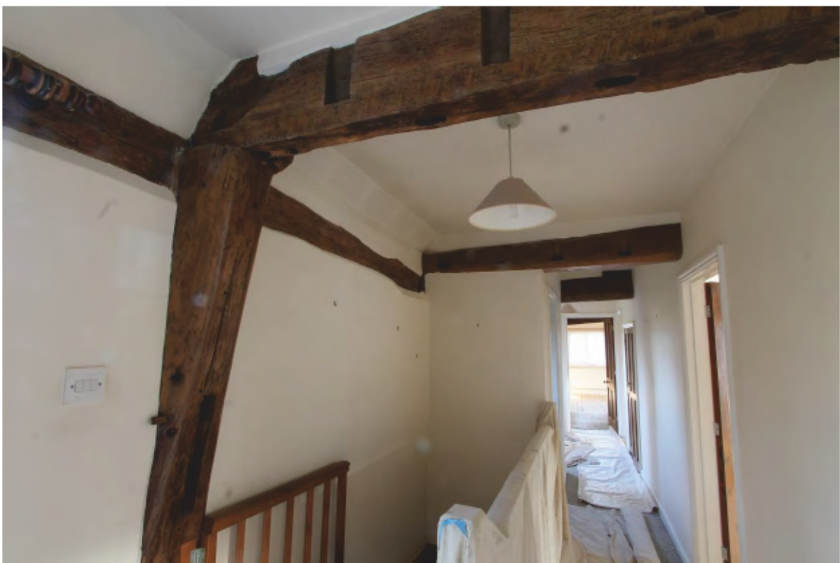
Plate 23 Jowl to storey post and tie-beam, looking east from bay 2
