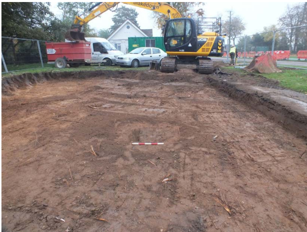
Plate 3: Location of Pit [5] in relation to overall Access Road Trench, looking east (BRBS15 D1 (22))
