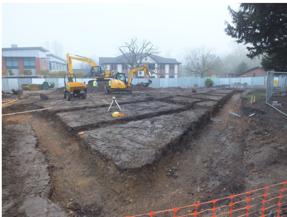
Plate 16: General shot showing excavation of D& T Footings Trench at south-west end, looking north-east (BRBS15 D1 (75))
