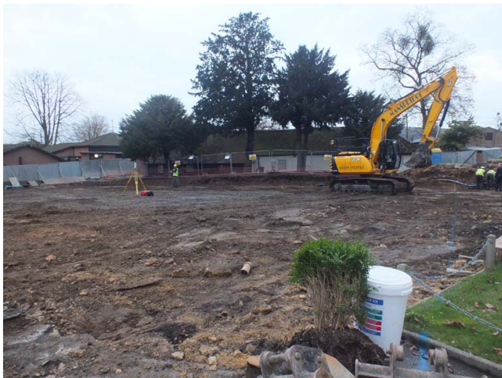
Plate 15: General site shot prior to excavation of D& T Footings Trench at north end, looking south (BRBS15 D1 (34))
