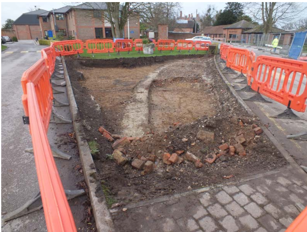
Plate 9: General shot of Access Road Trench at south-western extent, looking north-west (BRBS15 D2 (32))
