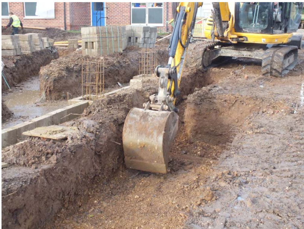
Plate 17: General shot showing excavation of D& T Footings Trench at NE end, looking north north-east (BRBS15 D2 (29))
