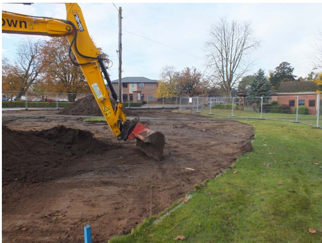
Plate 2: General shot showing machine stripping of turning point in new access road trench towards north-west extent, looking north-west (BRBS15 D1 (11))
