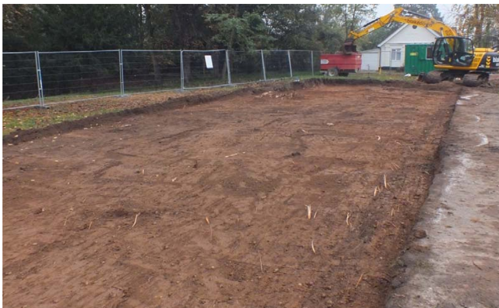
Plate 1: General shot showing machine stripping of Access Road Trench at eastern extent, looking north-east (BRBS15 D1 (24))
