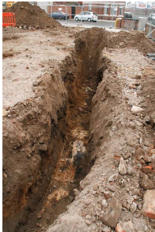
Plate 8. Area 4, detail of westernmost foundation trench with limestone bedrock exposed in base, looking south
