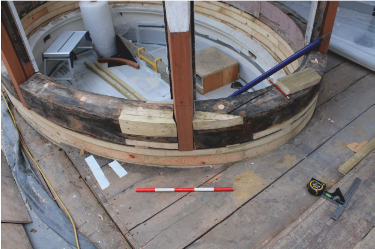
Plate 106 Lantern B: Repaired sill sections and new Sapele hardwood mullion inserts looking south-east
