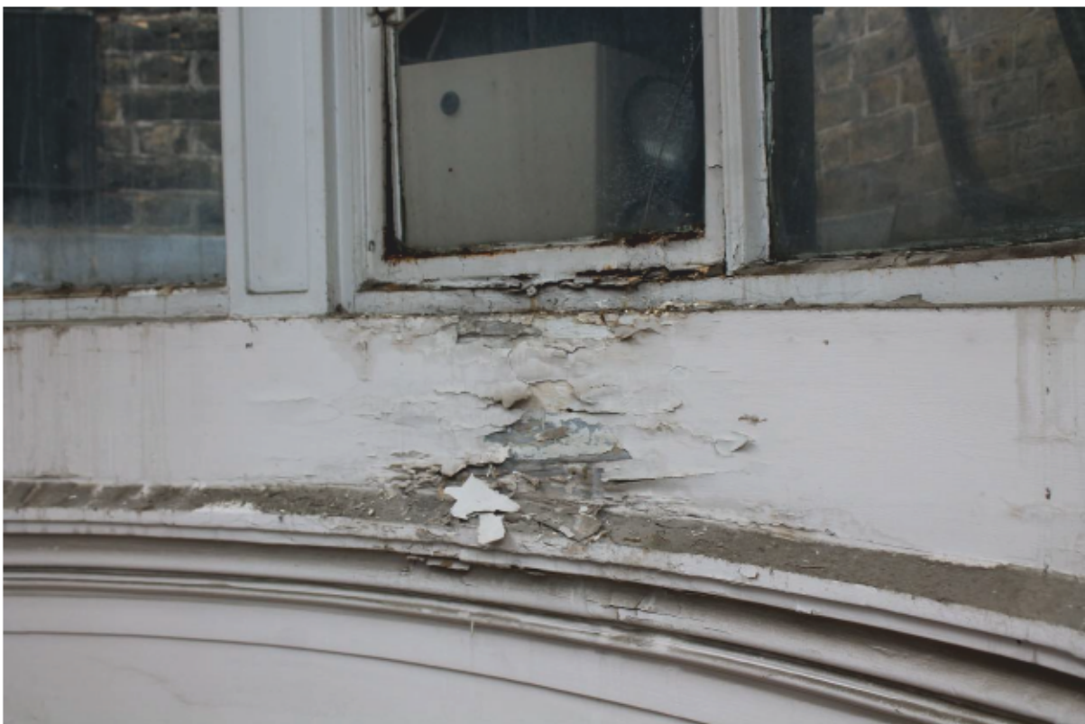
Plate 72 Lantern C: Decay below casement 30
