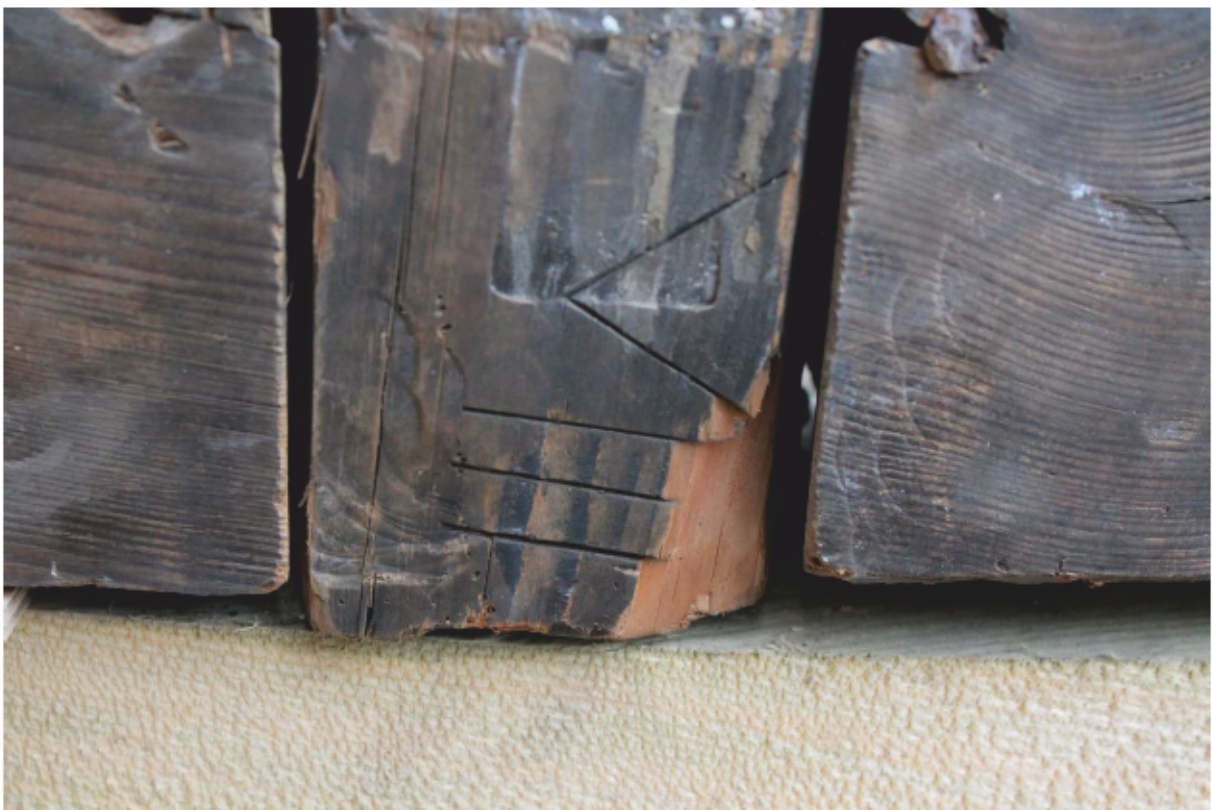
Plate 104 Lantern B: Roman marking to mullion foot
