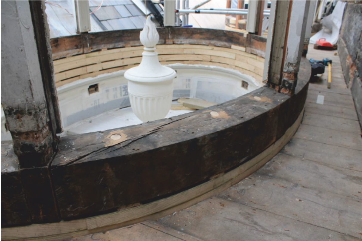
Plate 105 Lantern A: Sectional sill repaired and fixed to new composite sill, looking north-east
