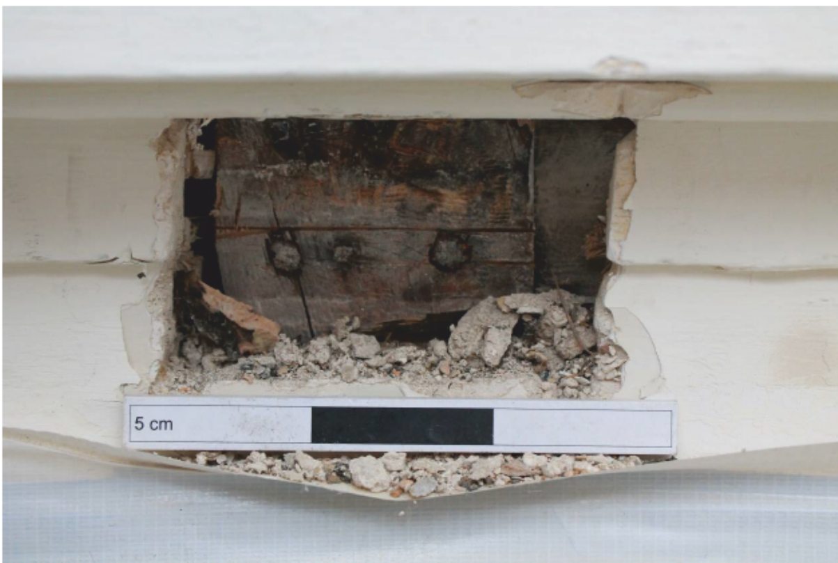
Plate 98 Lantern B: Mullion foot halved over and nailed into sub-structure (viewed through internal plaster moulding)
