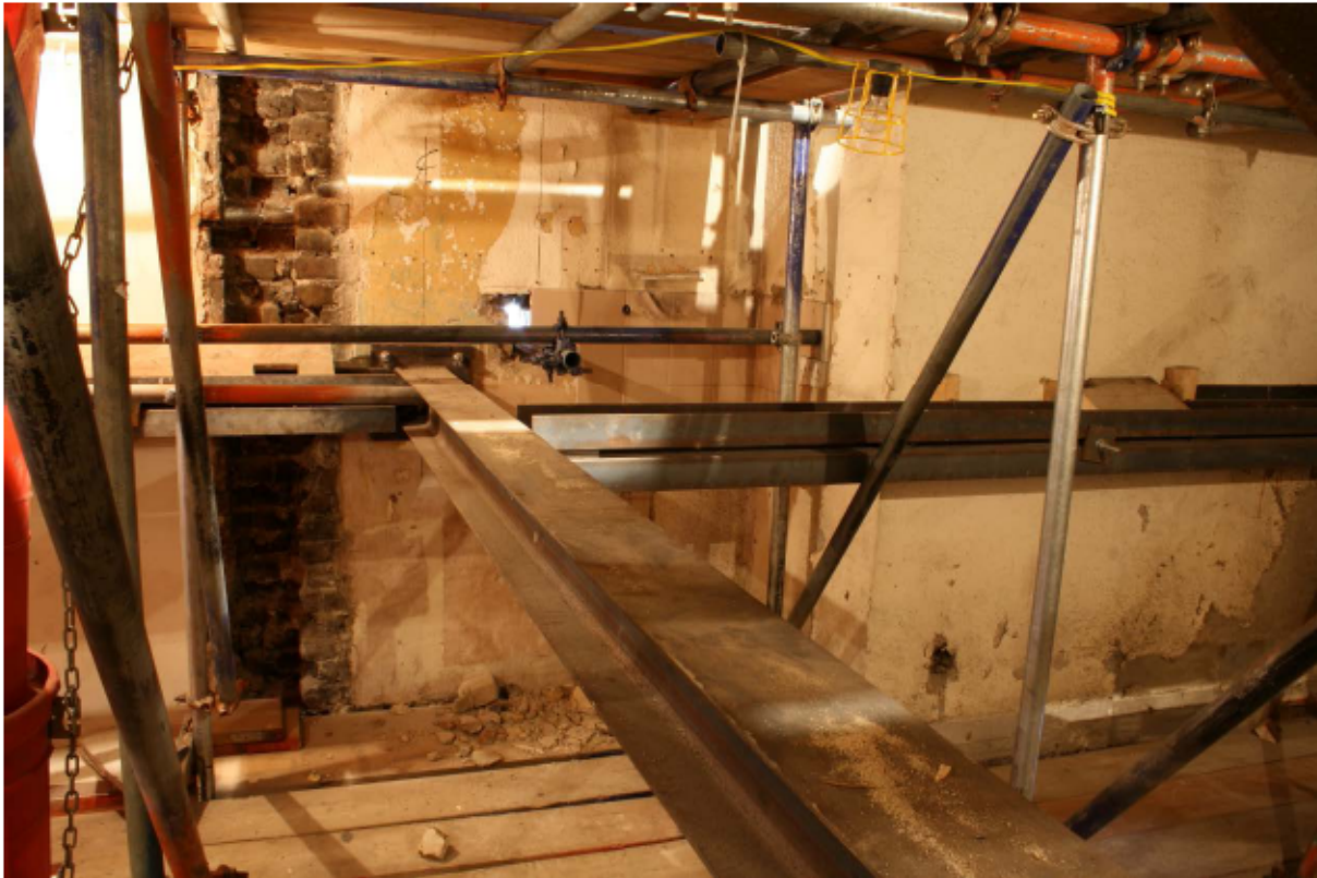
Plate 68 Towards the east end of the Internal north wall of no. 141 Borough High Street at first floor level, looking north
