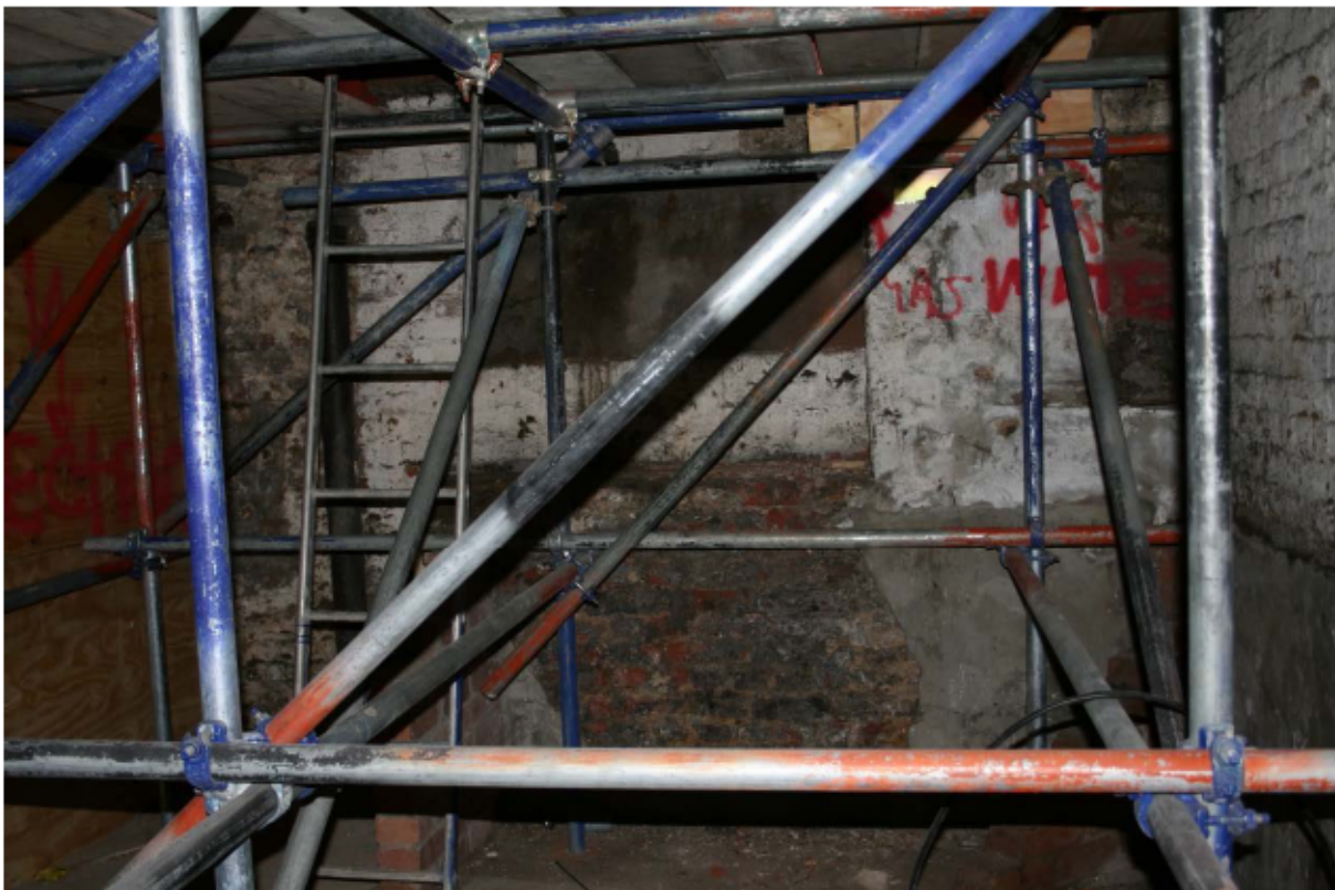
Plate 15 Internal west (front) wall of no. 141 Borough High Street at basement level, looking west
