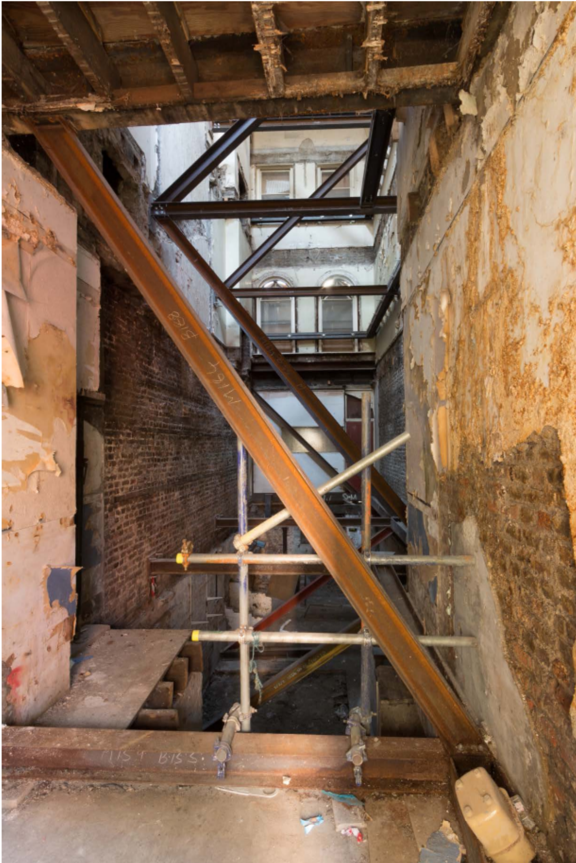
Plate 13 Internal west (front) wall of no. 141 Borough High Street at ground floor level, looking west
