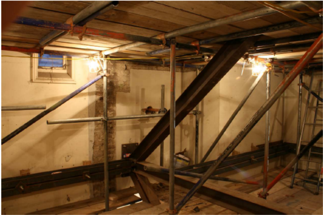
Plate 78 North wall of no. 141 Borough High Street at second floor level, looking north-east
