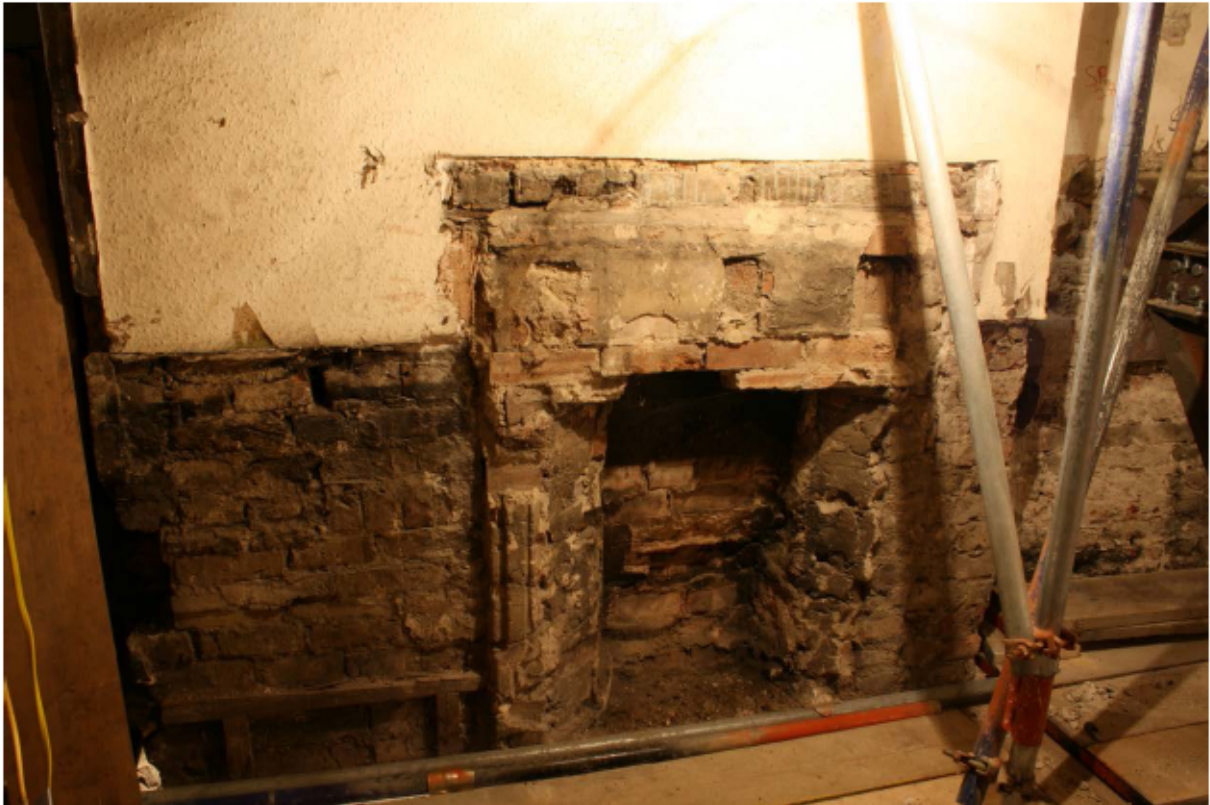
Plate 31 Fireplace at the east end of the south wall of no. 141 Borough High Street at first floor level, looking south
