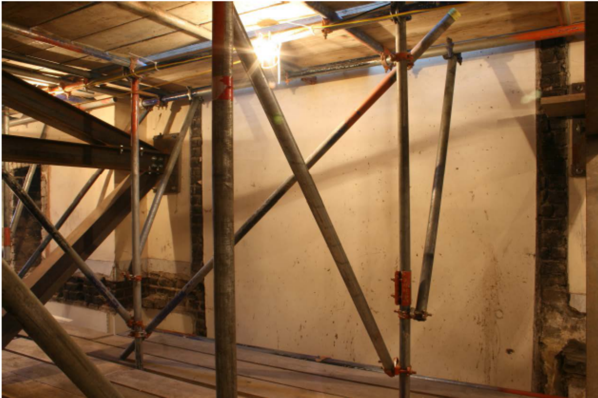
Plate 47 Internal south wall of no. 141 Borough High Street at third floor level, looking south-east
