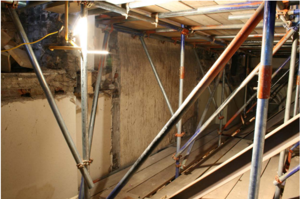
Plate 37 Internal south wall of no. 141 Borough High Street at first/second floor level, looking south-west
