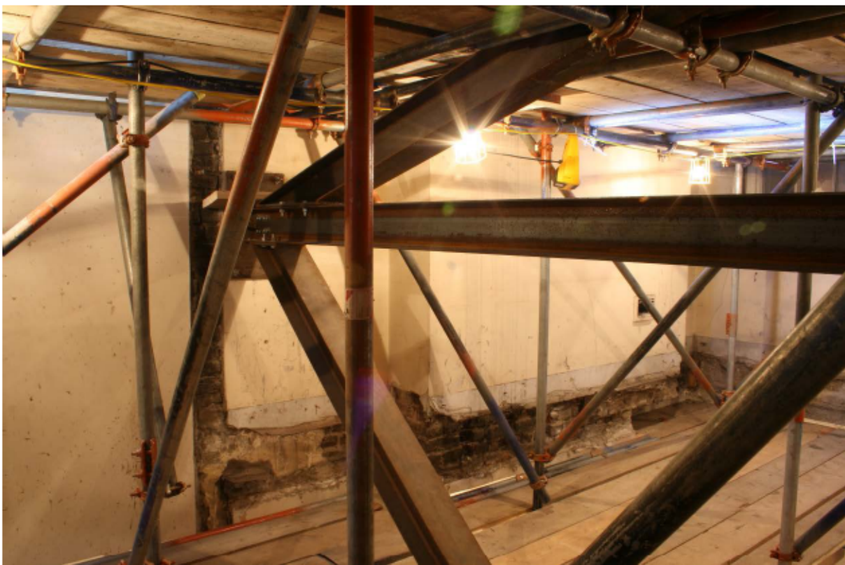
Plate 48 Chimney breast at the west end of the south wall of no. 141 Borough High Street at third floor level, looking south-west
