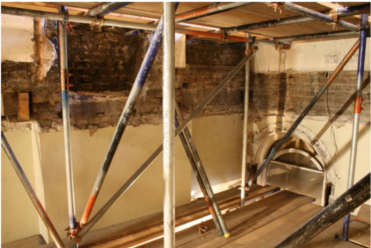
Plate 40 Chimney breast at the west end of the south wall and west wall of no. 141 Borough High Street at first/second floor level, looking south-west
