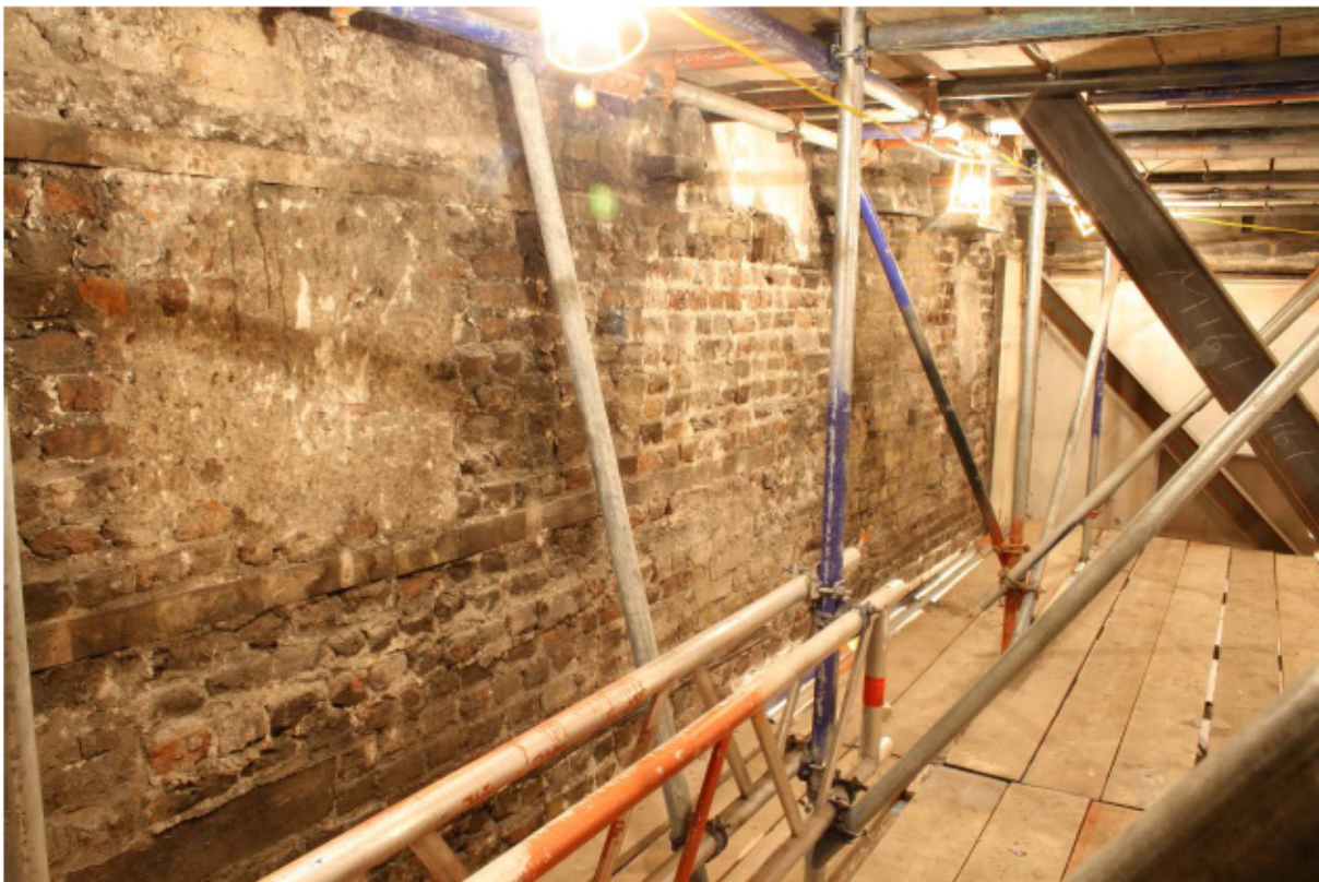
Plate 30 Internal south wall of no. 141 Borough High Street at ground (upper part) floor level, looking south-west
