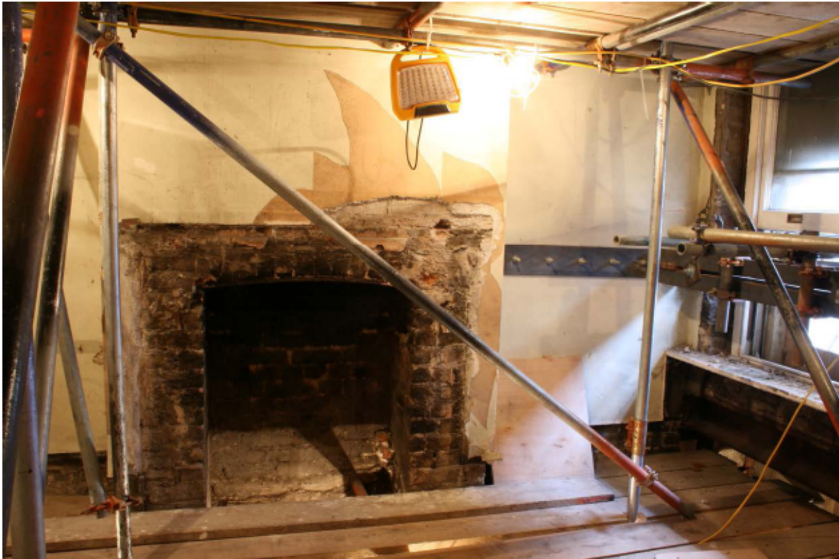
Plate 35 Fireplace at the west end of the south wall of no. 141 Borough High Street at first floor level, looking south-west
