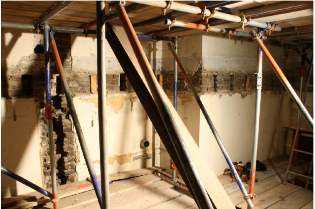
Plate 73 Scar of the second floor along the east end of the north wall of no. 141 Borough High Street, looking north
