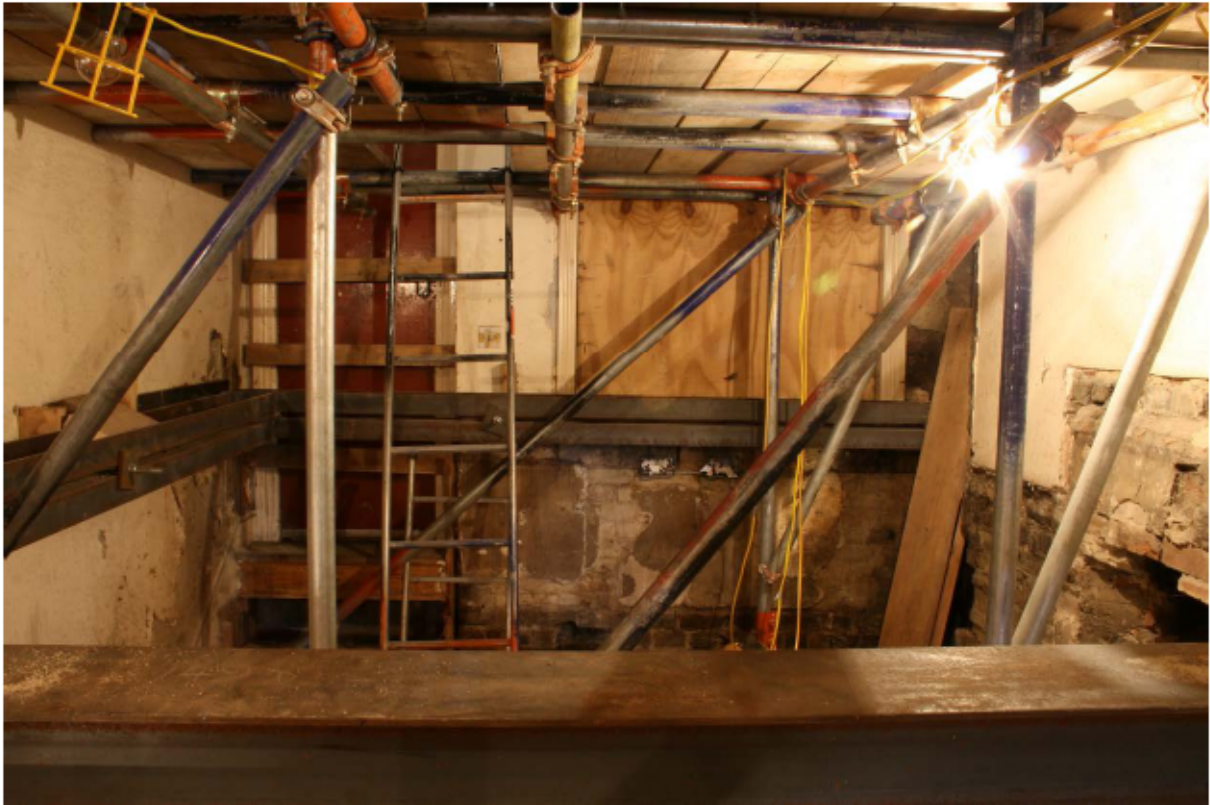
Plate 51 Internal east wall of no. 141 Borough High Street at first floor level, looking east
