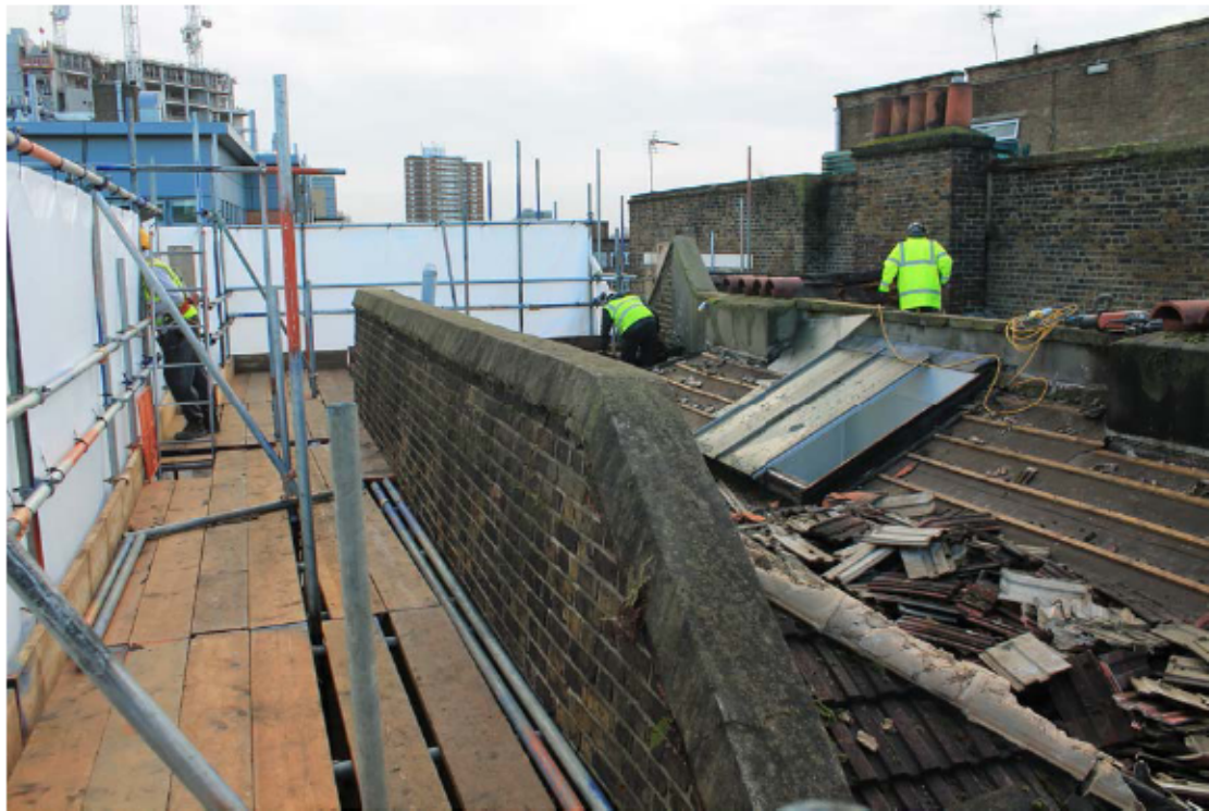
Plate 83: North parapet and roof over no. 141 Borough High Street during removal of the tiles, looking south-east
