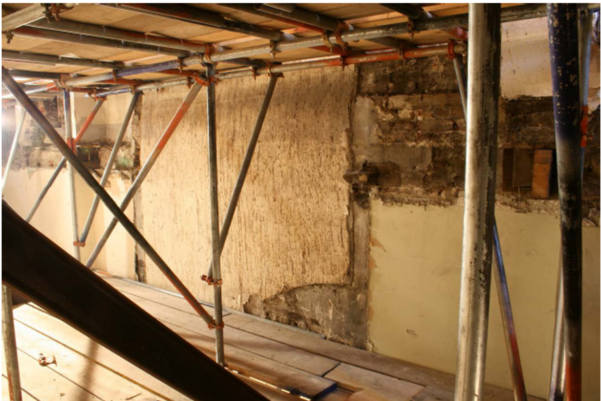
Plate 38 Internal south wall of no. 141 Borough High Street at first/second floor level, looking south-east
