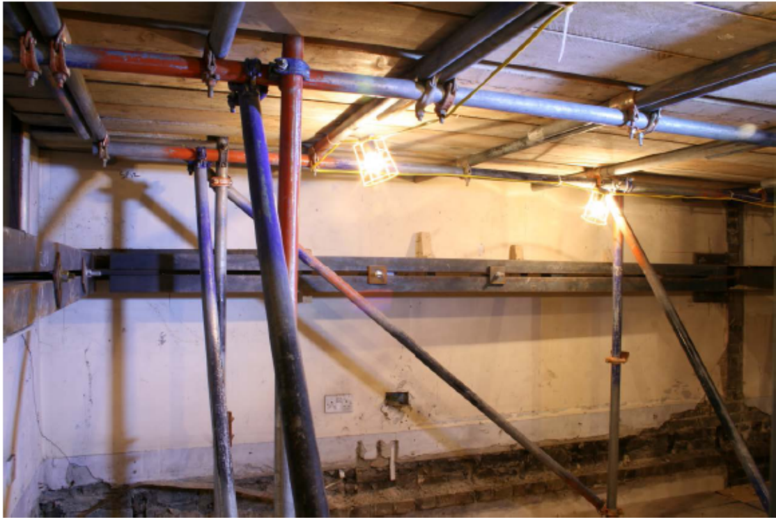
Plate 80 West end of the north wall of no. 141 Borough High Street at third floor level, looking north
