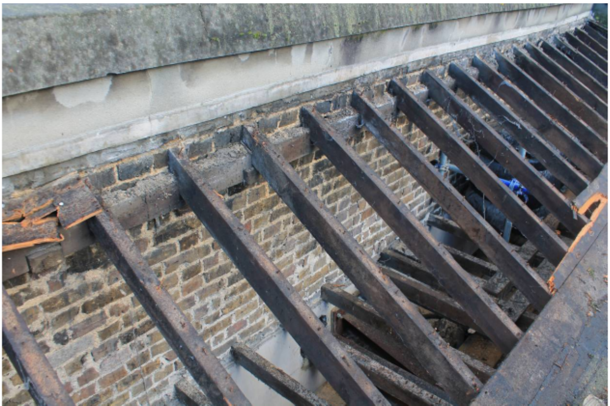
Plate 85: Rafters against the north parapet wall of no. 141 Borough High Street during stripping, looking north-east
