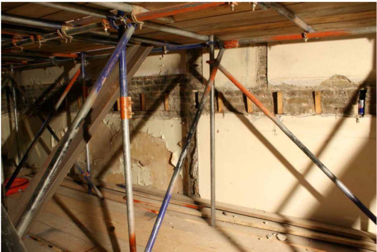
Plate 71 Scar of the second floor along the north wall of no. 141 Borough High Street, looking north
