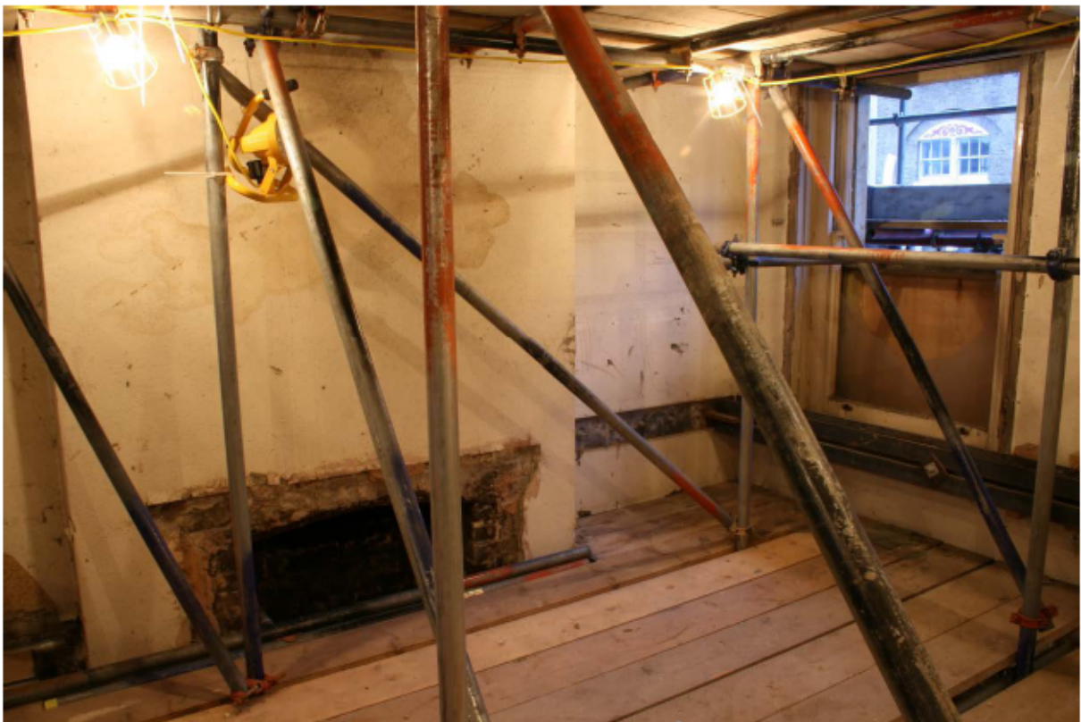
Plate 44 Chimney breast at the west end of the south wall of no. 141 Borough High Street at second floor level, looking south-west
