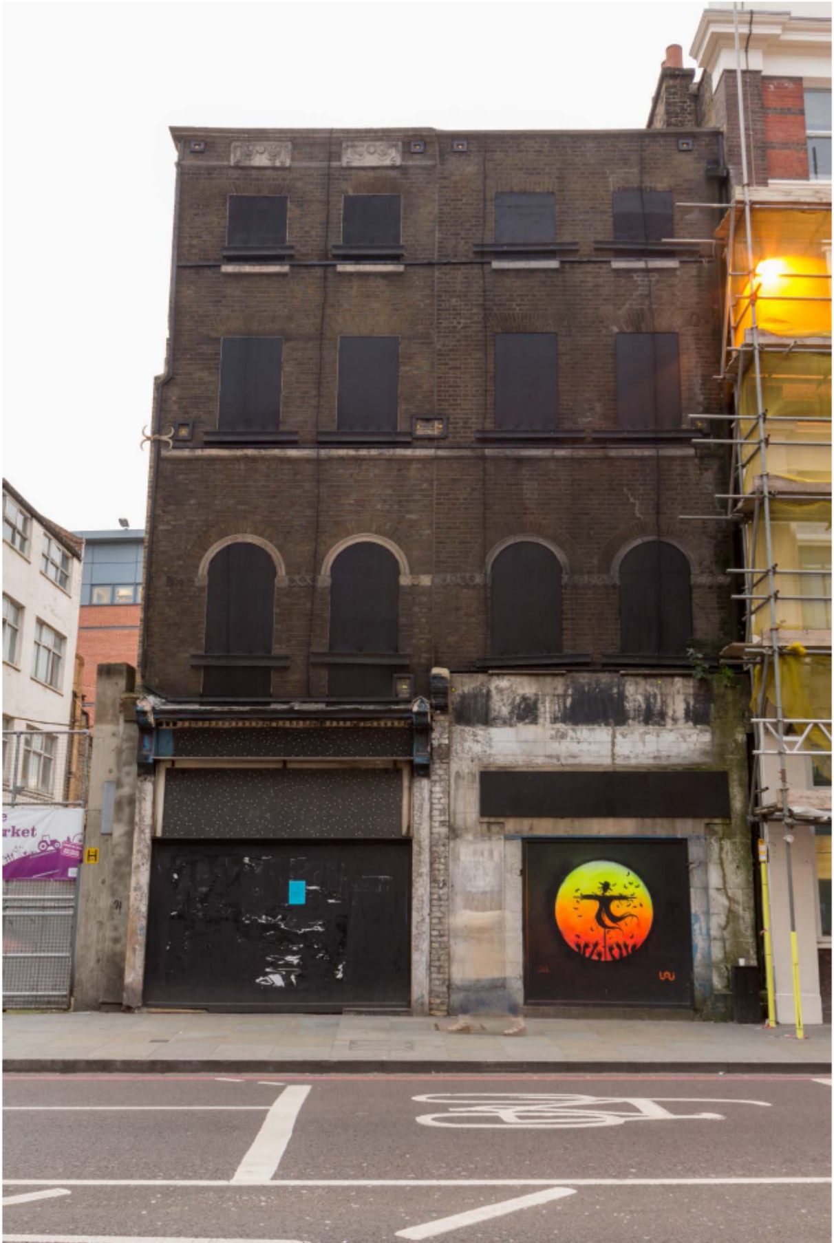
Plate 3 Nos 141 (left) and 143 (right) Borough High Street covered with netting, looking east
