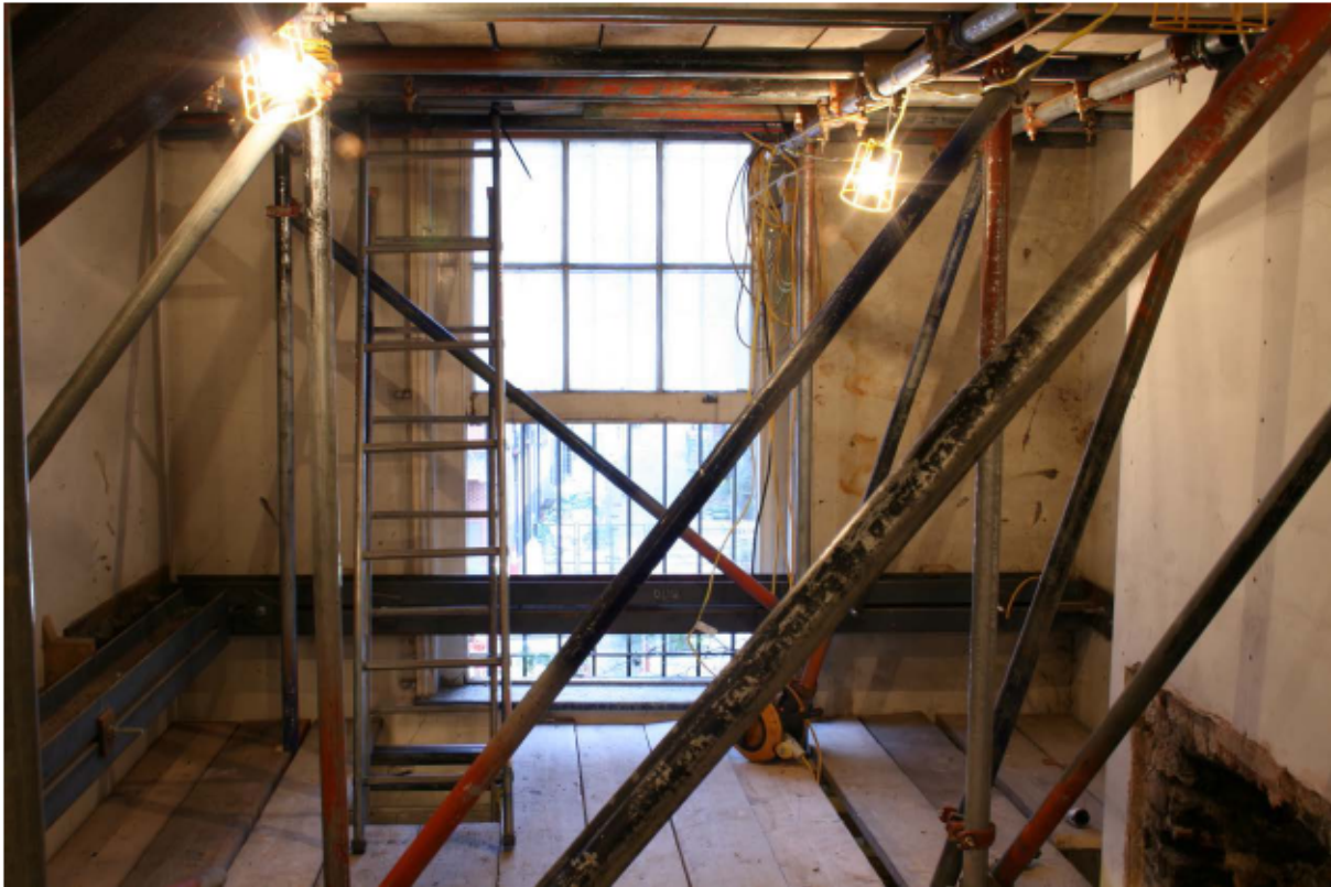
Plate 53 Internal east wall of no. 141 Borough High Street at second floor level, looking east
