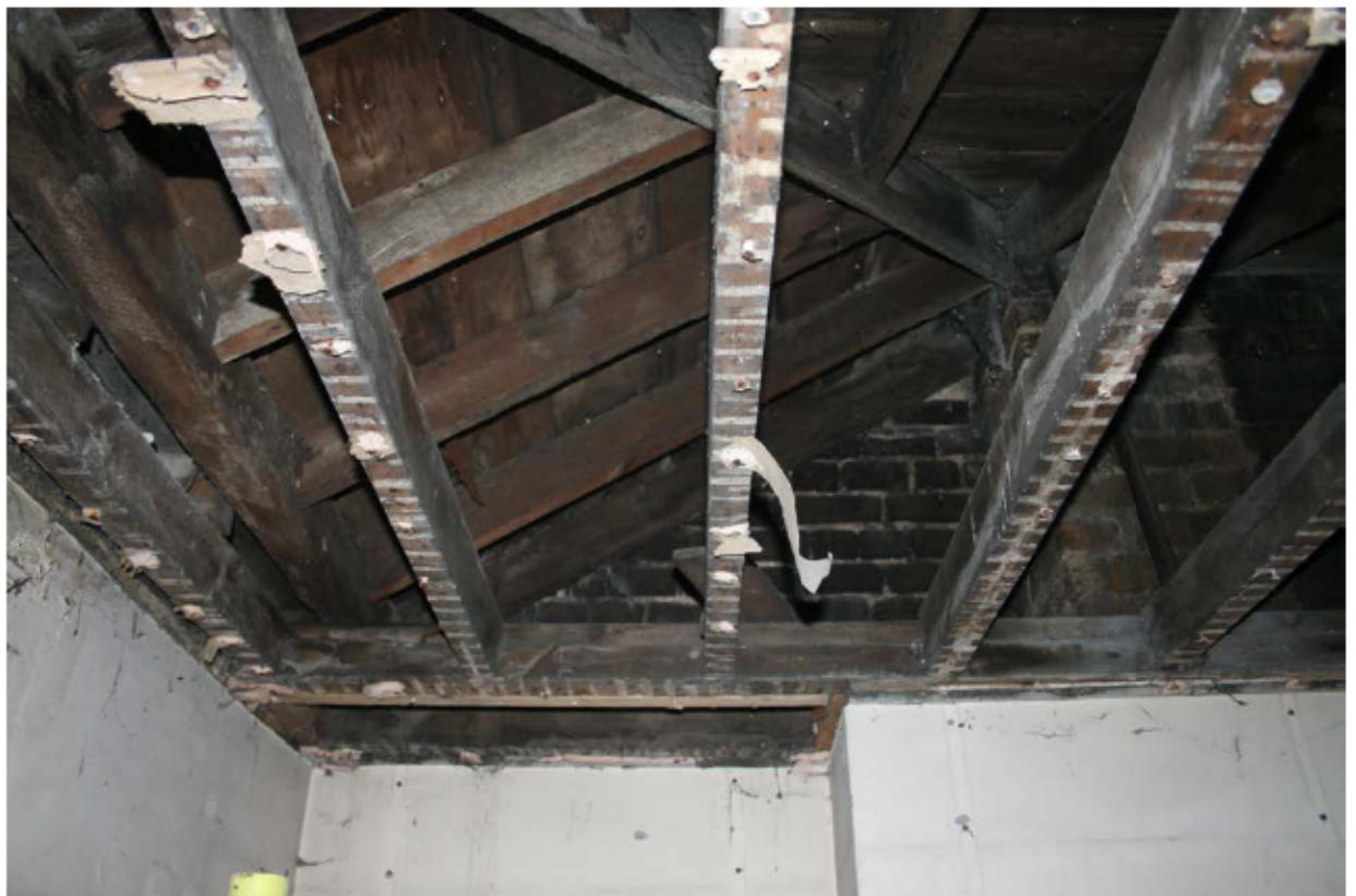
Plate 87: Hipped roof structure over the south-east corner of no. 141 Borough High Street, looking south
