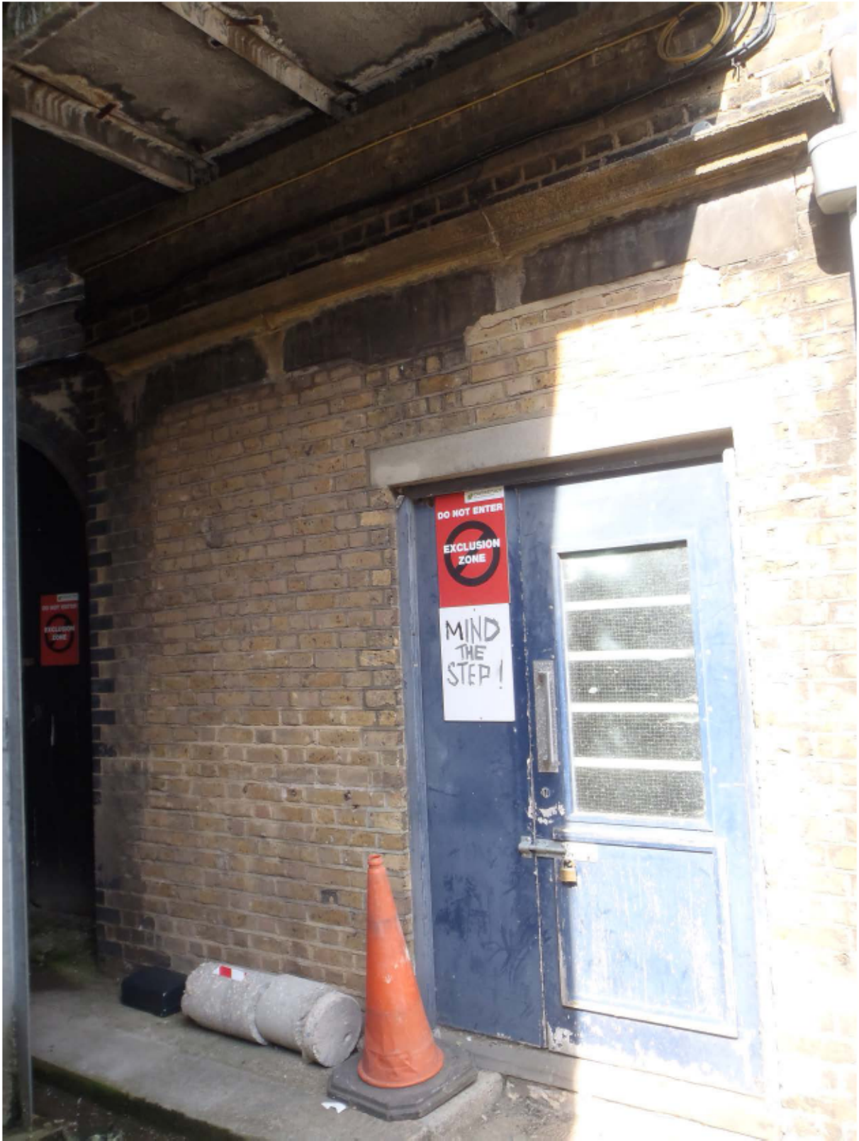
Plate 10 Back door in east (rear) elevation of no. 141 Borough High Street, looking south-west
