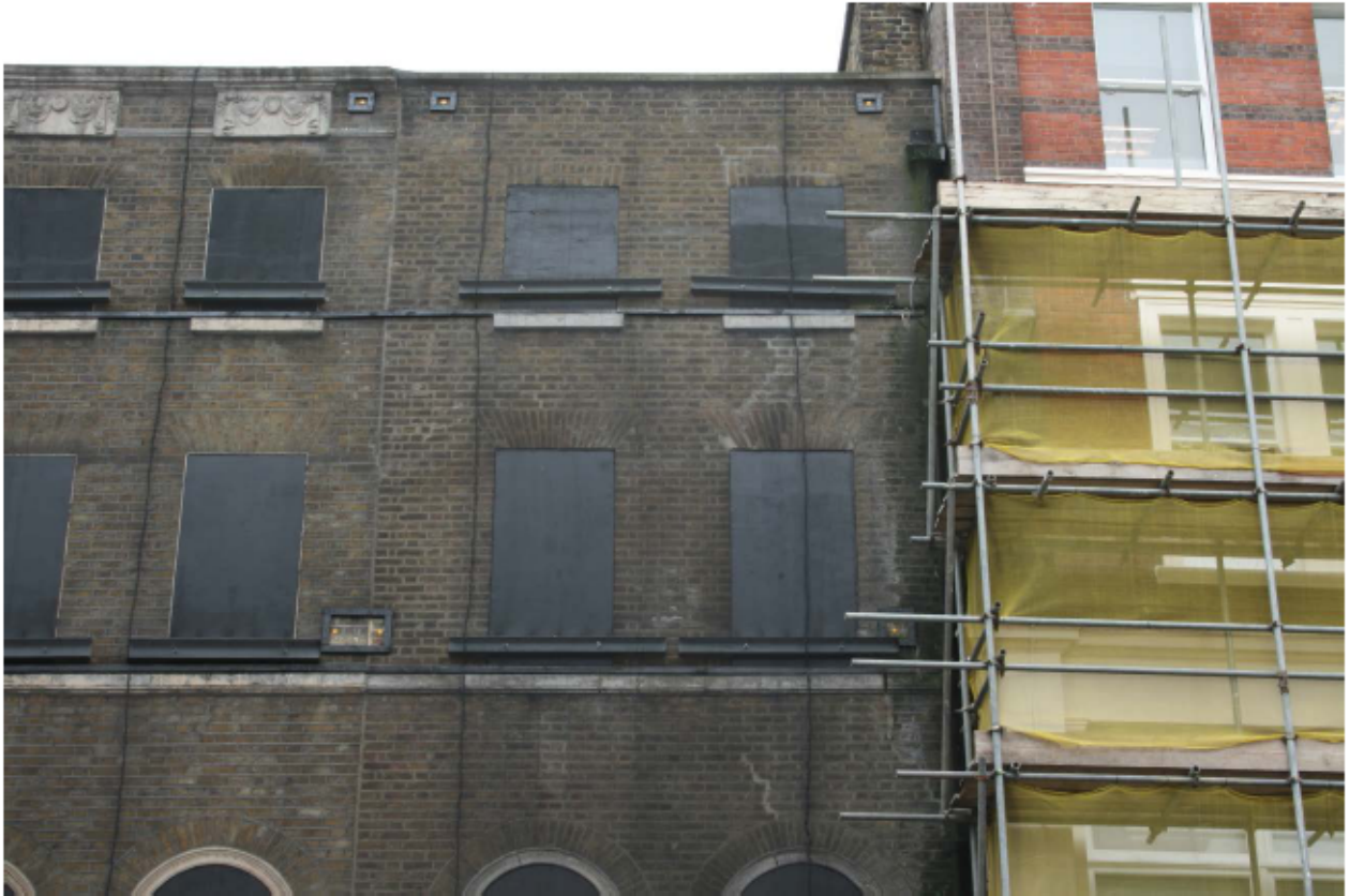
Plate 6 Nos 141 (left) and 143 (centre) Borough High Street at second and third floor levels, looking east
