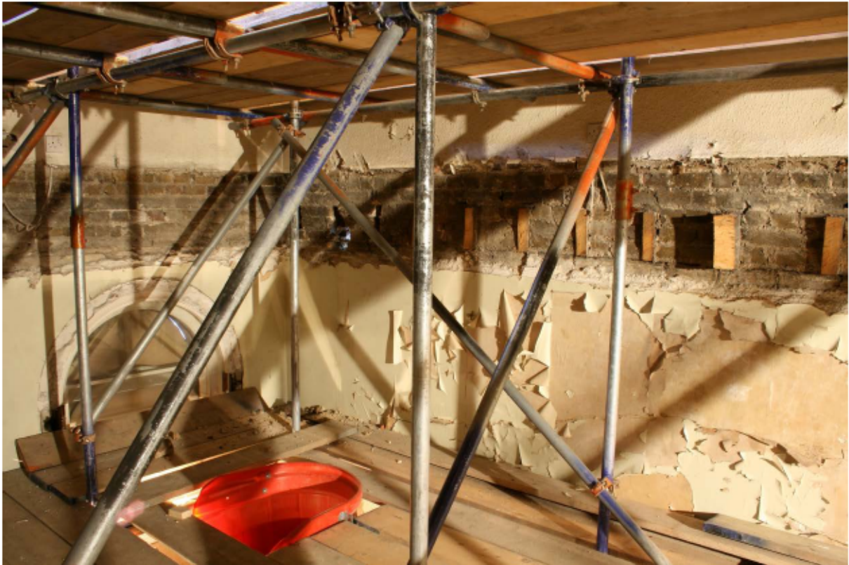
Plate 70 Scar of the second floor along the west (left) and north (right) walls of no. 141 Borough High Street, looking north-west
