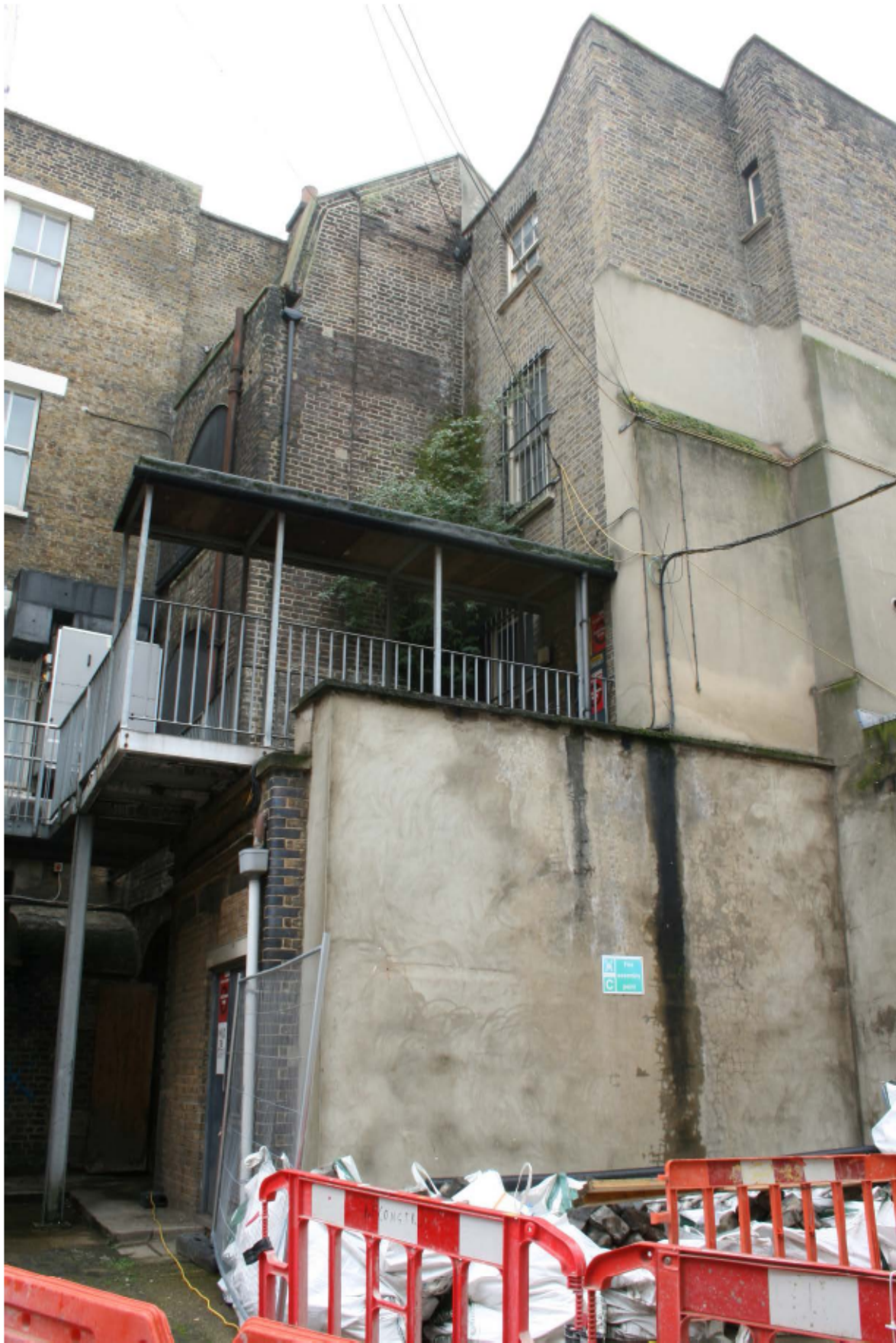
Plate 8 East (rear) and north (side) elevation of no. 141 Borough High Street, looking south-west
