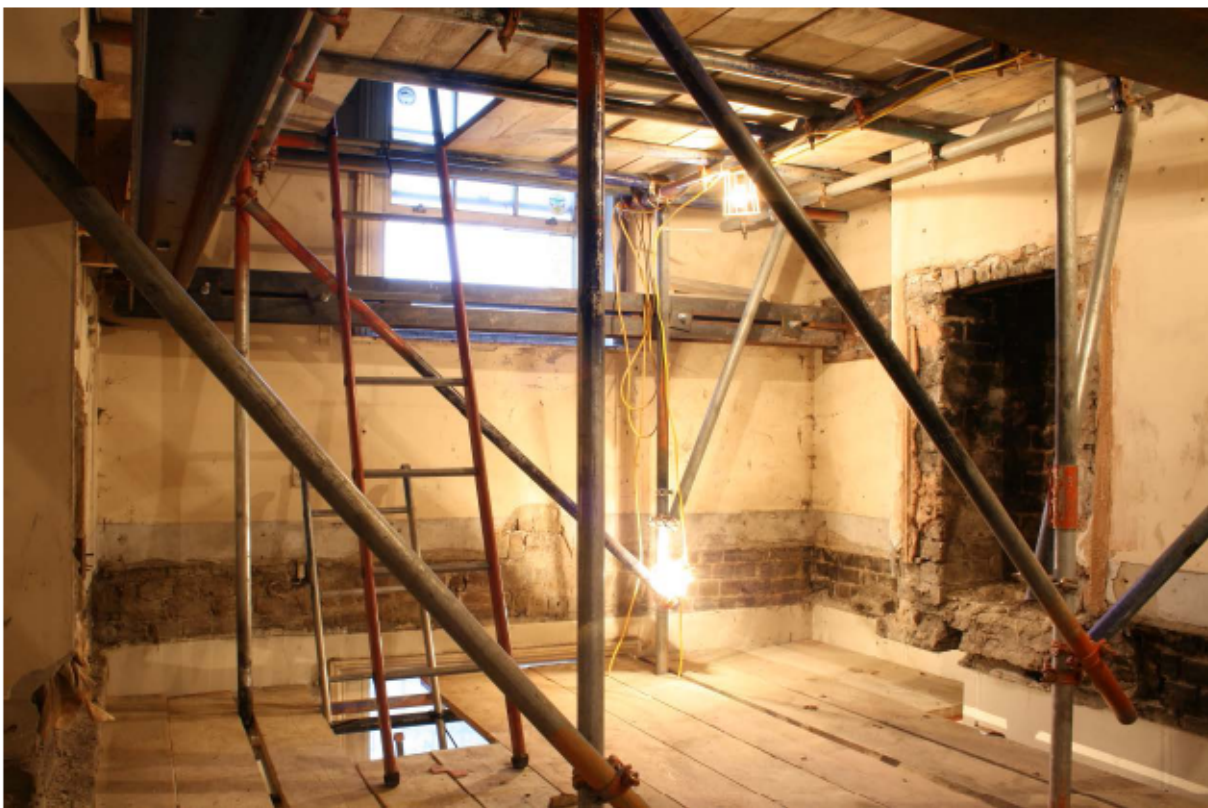
Plate 54 Internal east (centre) and south (right) walls of no. 141 Borough High Street at third floor level, looking east
