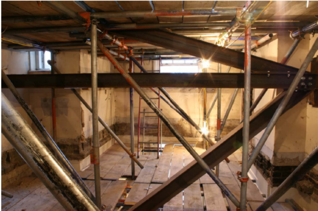
Plate 82 North (left) and east (centre) walls of no. 141 Borough High Street at third floor level, looking east
