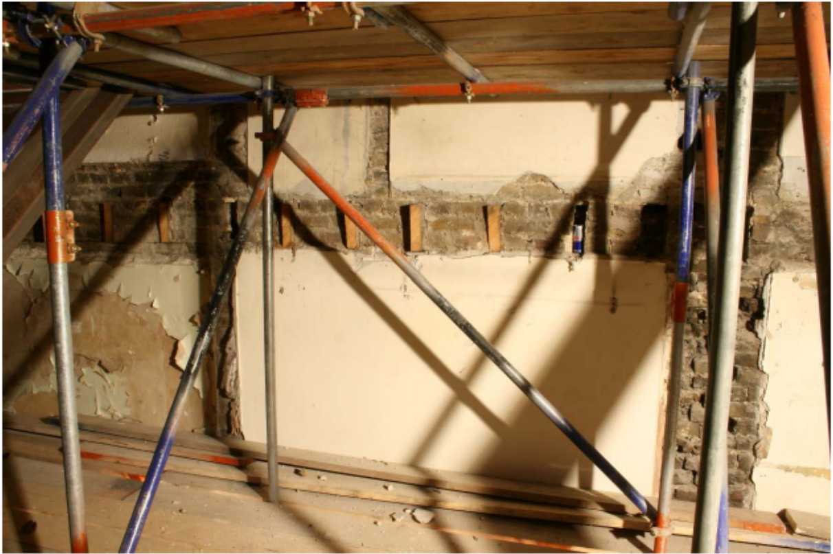
Plate 72 Scar of the second floor along the north wall of no. 141 Borough High Street, looking north
