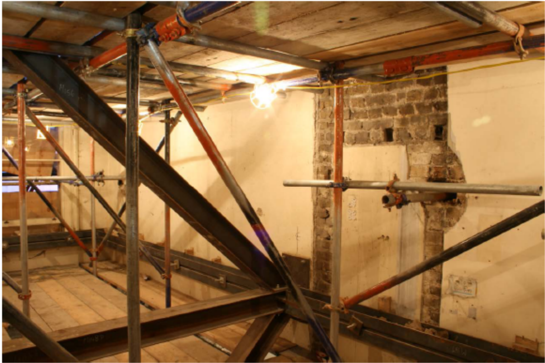
Plate 76 North wall of no. 141 Borough High Street at second floor level, looking north-west
