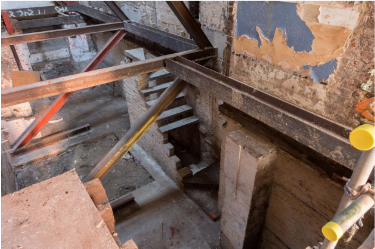
Plate 56 Internal north wall of no. 141 Borough High Street at basement level, looking north-west
