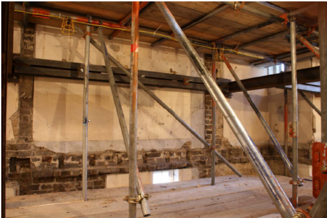
Plate 81 North wall of no. 141 Borough High Street at third floor level, looking north
