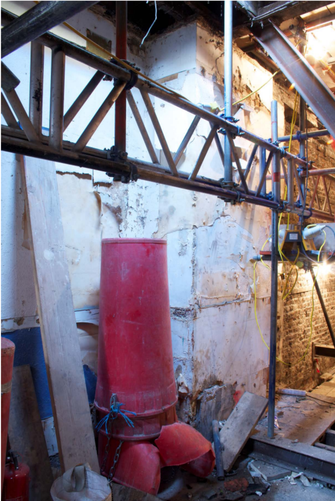
Plate 24 Internal south wall of no. 141 Borough High Street at ground floor level, looking south-west
