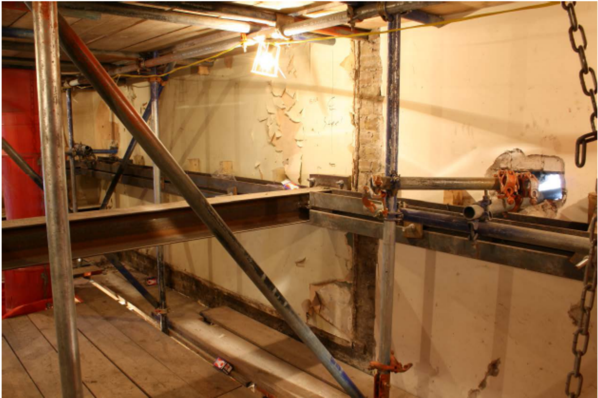
Plate 66 Internal north wall of no. 141 Borough High Street at first floor level, looking north-west
