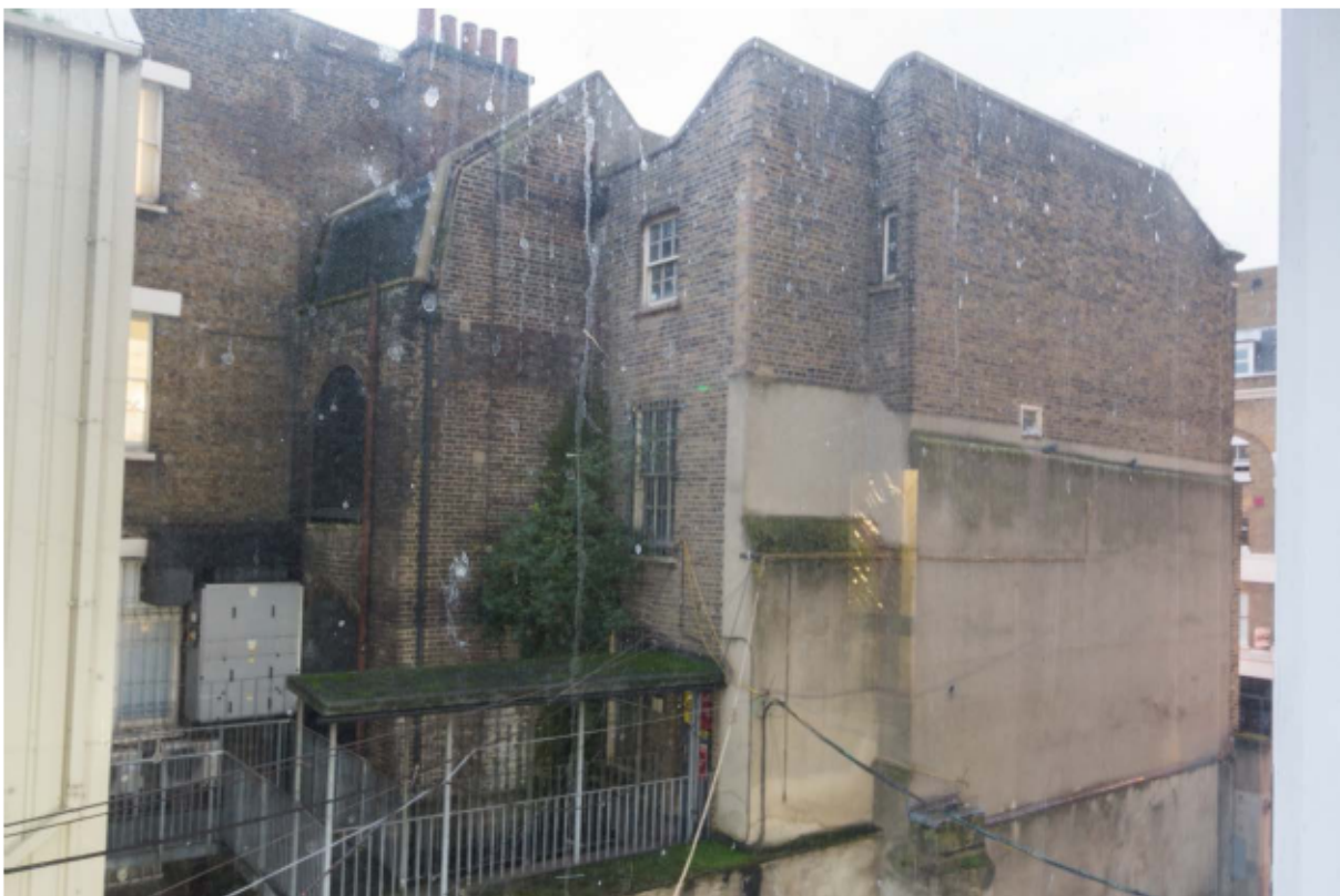
Plate 12 East (rear) and north (side) elevation of no. 141 Borough High Street at first floor level and above, looking south-west
