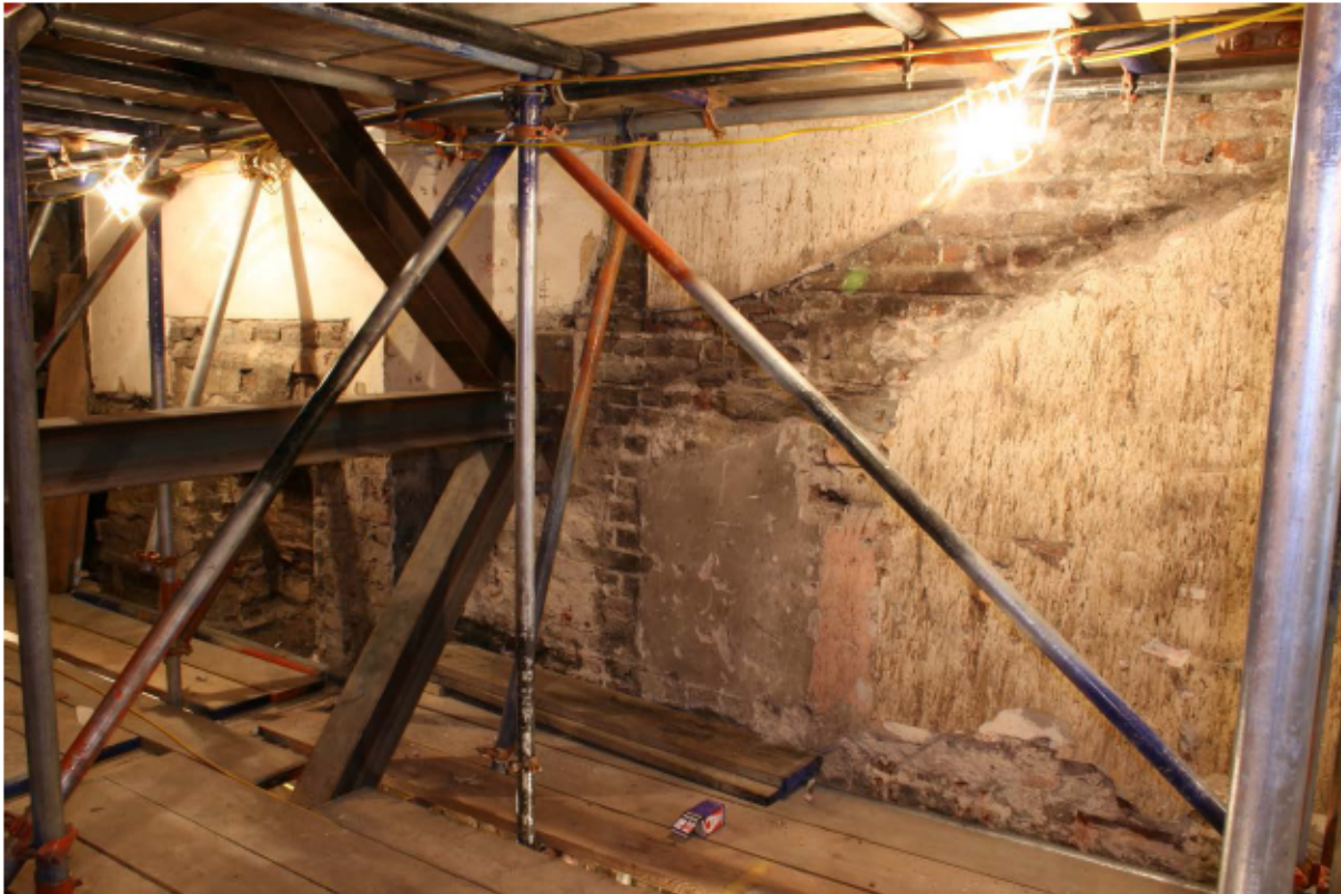
Plate 33 Internal south wall of no. 141 Borough High Street at first floor level, looking south-east
