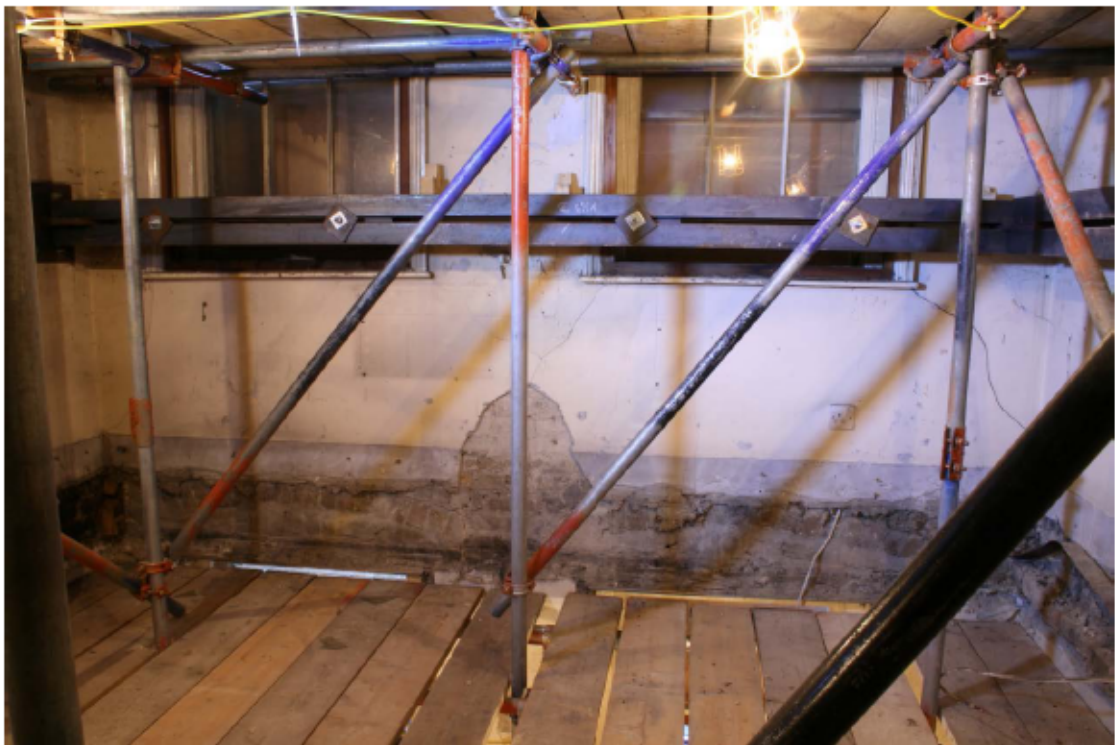
Plate 79 West wall of no. 141 Borough High Street at third floor level, looking west
