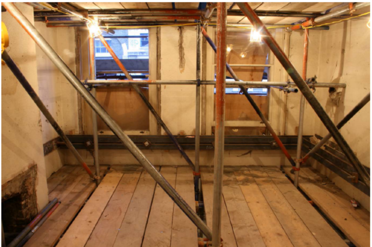
Plate 74 Second floor windows in the west wall of no. 141 Borough High Street, looking west
