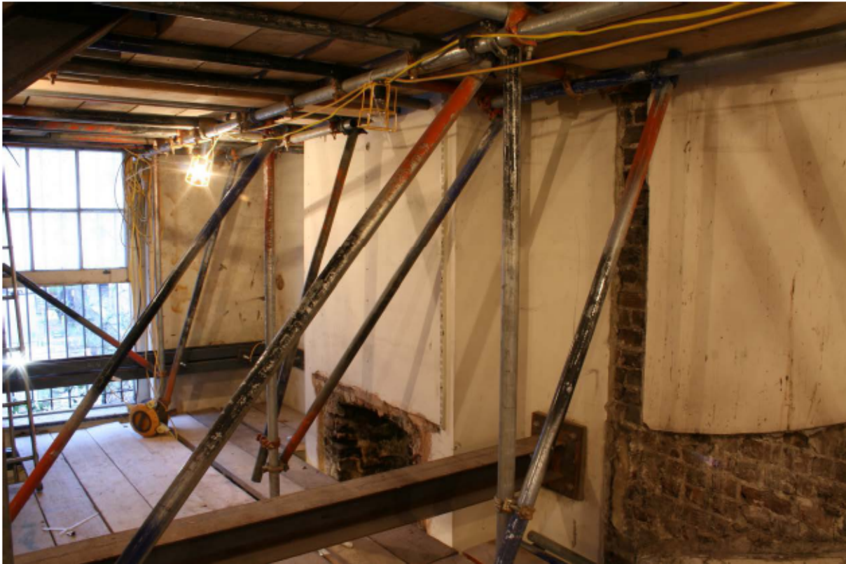
Plate 41 Chimney breast at the east end of the south wall of no. 141 Borough High Street at second floor level, looking south-east
