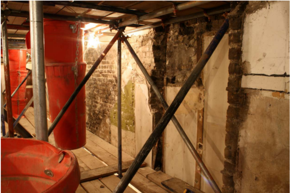
Plate 64 Internal north wall of no. 141 Borough High Street at ground floor level, looking north-west
