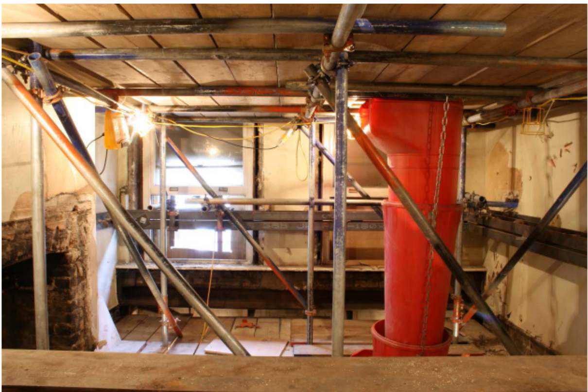
Plate 65 Internal west wall of no. 141 Borough High Street at first floor level, looking west
