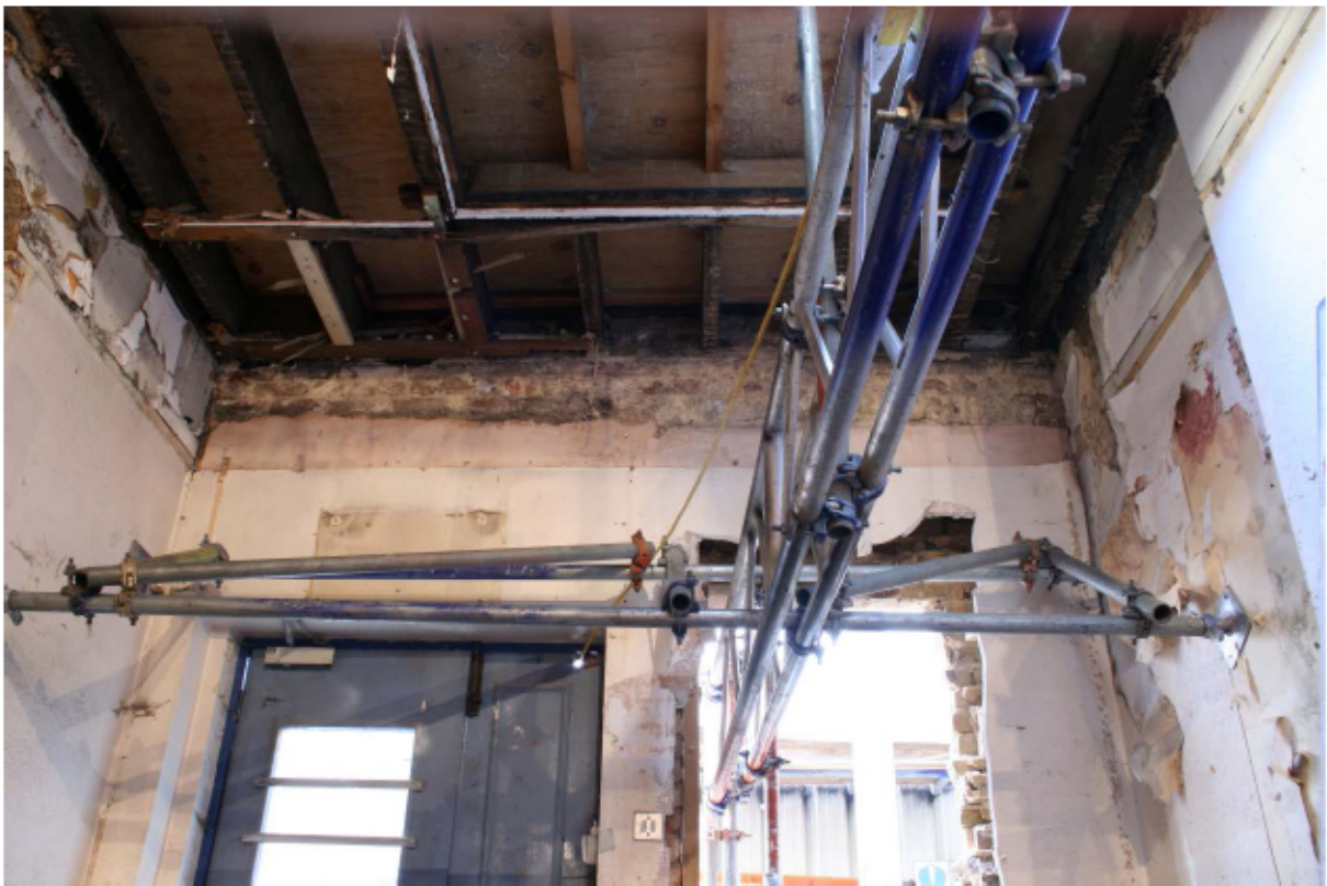
Plate 50 Internal east wall of no. 141 Borough High Street at ground floor level, looking east
