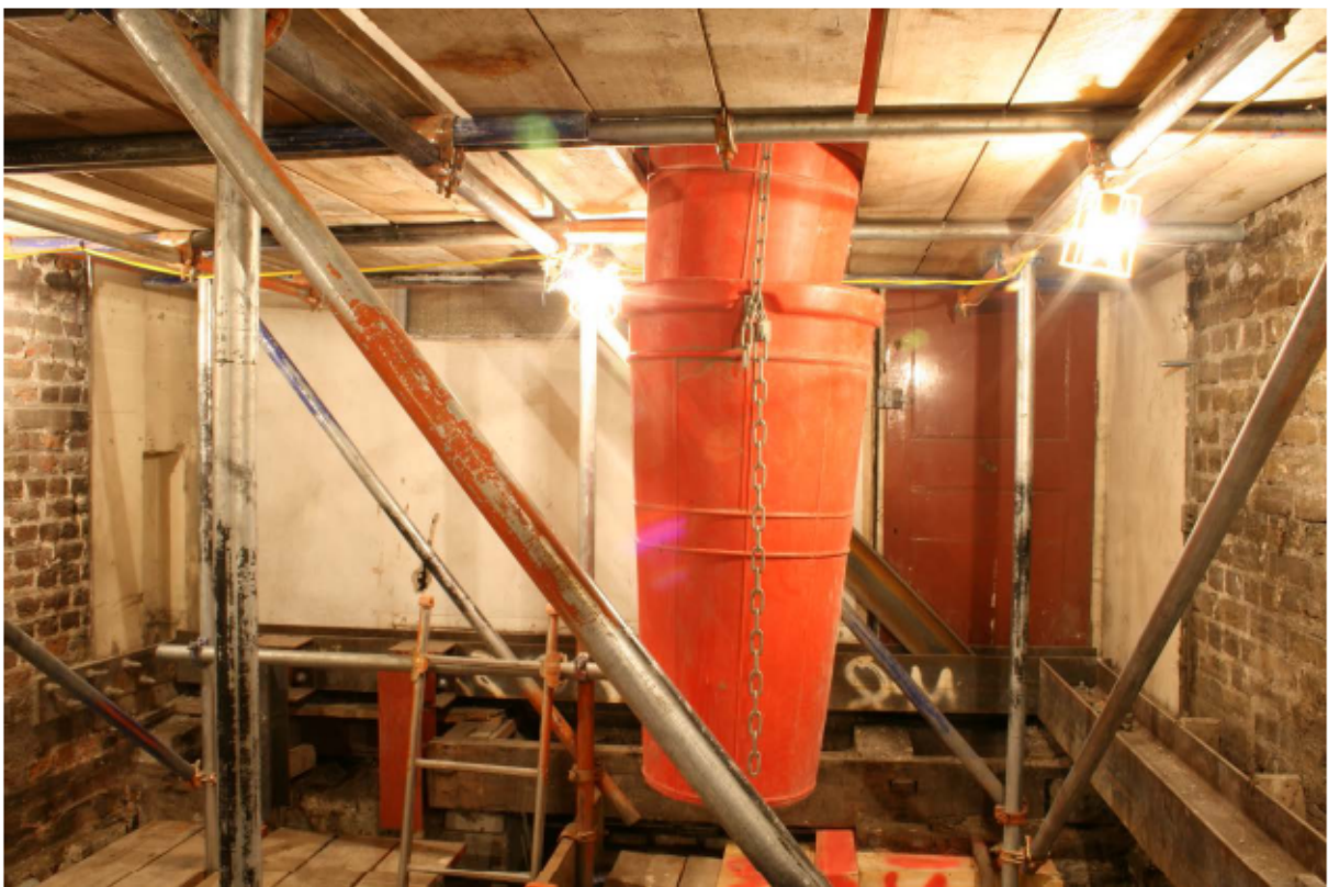
Plate 28 Internal west wall of no. 141 Borough High Street at ground floor level, looking west
