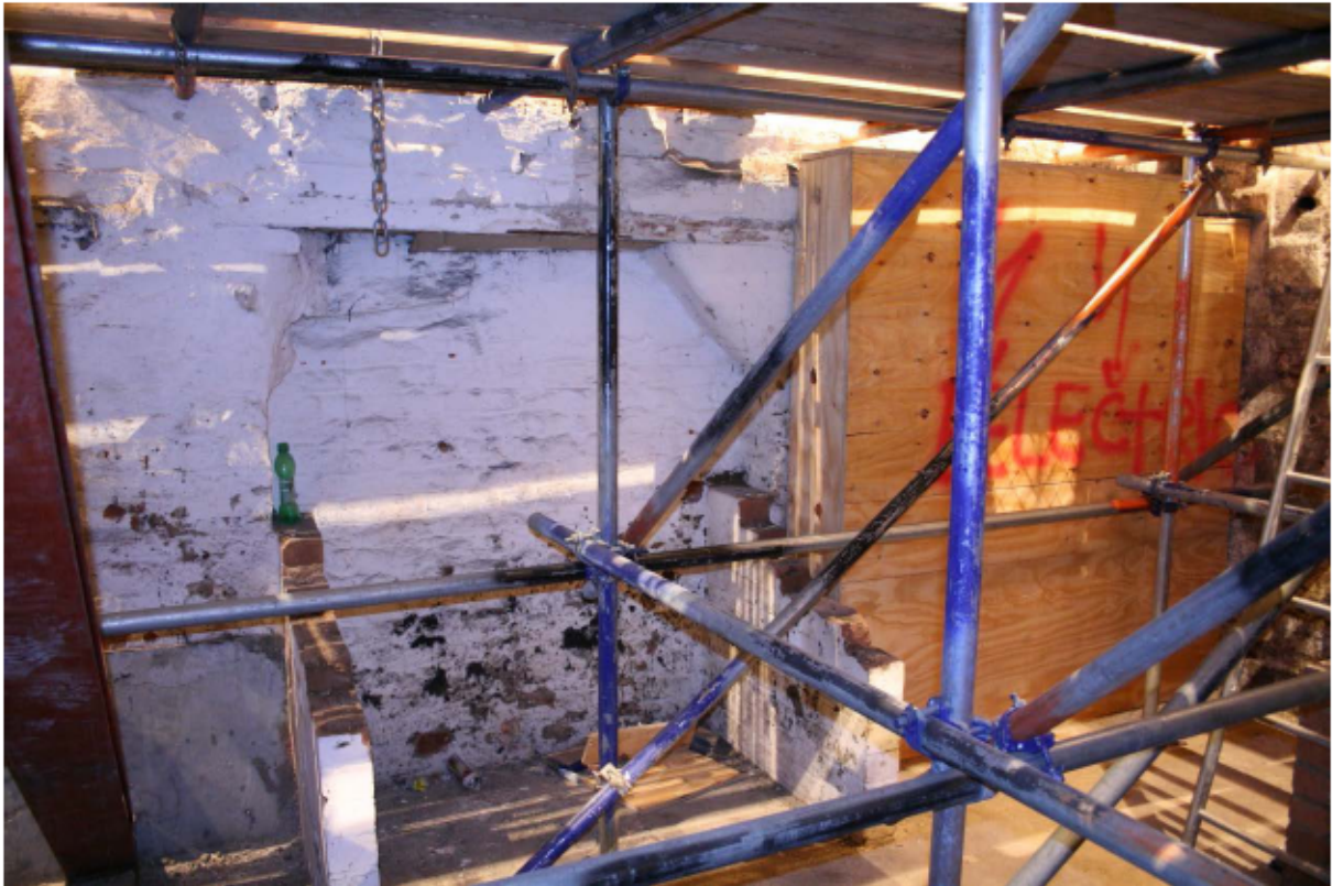
Plate 20 West end of internal south wall of no. 141 Borough High Street at basement level, looking south-west
