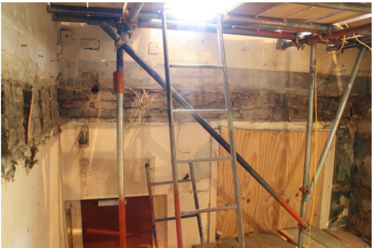
Plate 52 Internal east wall of no. 141 Borough High Street at first (upper part) floor level, looking east
