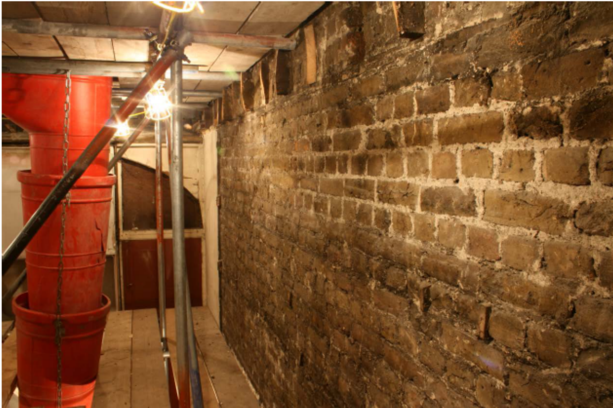
Plate 62 Internal west (left) and north (right) walls of no. 141 Borough High Street at ground floor level, looking north-west
