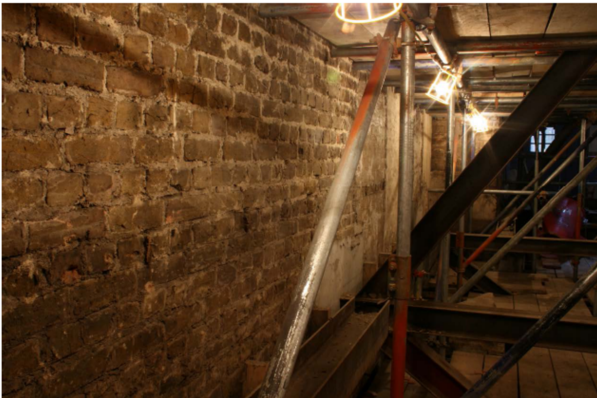
Plate 61 Internal north (right) walls of no. 141 Borough High Street at ground floor level, looking north-east
