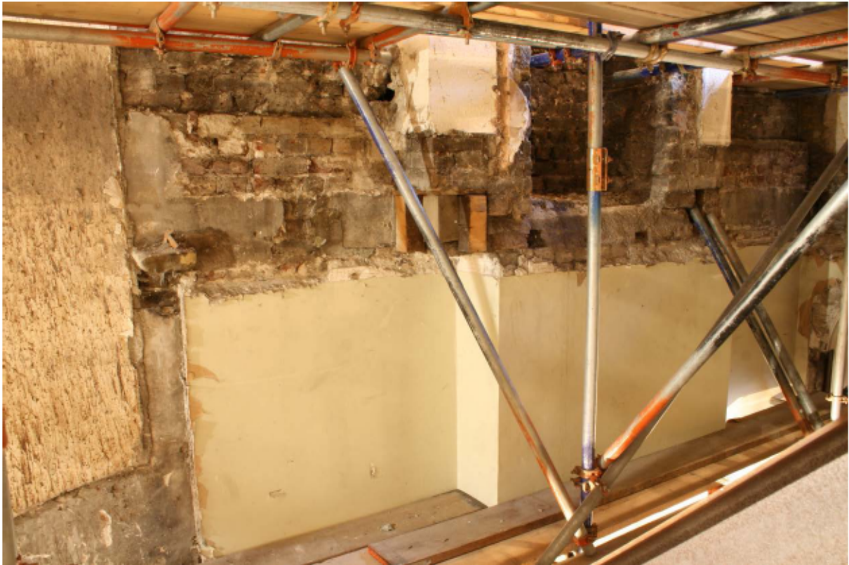
Plate 39 Chimney breast at the west end of the south wall of no. 141 Borough High Street at first/second floor level, looking south-west
