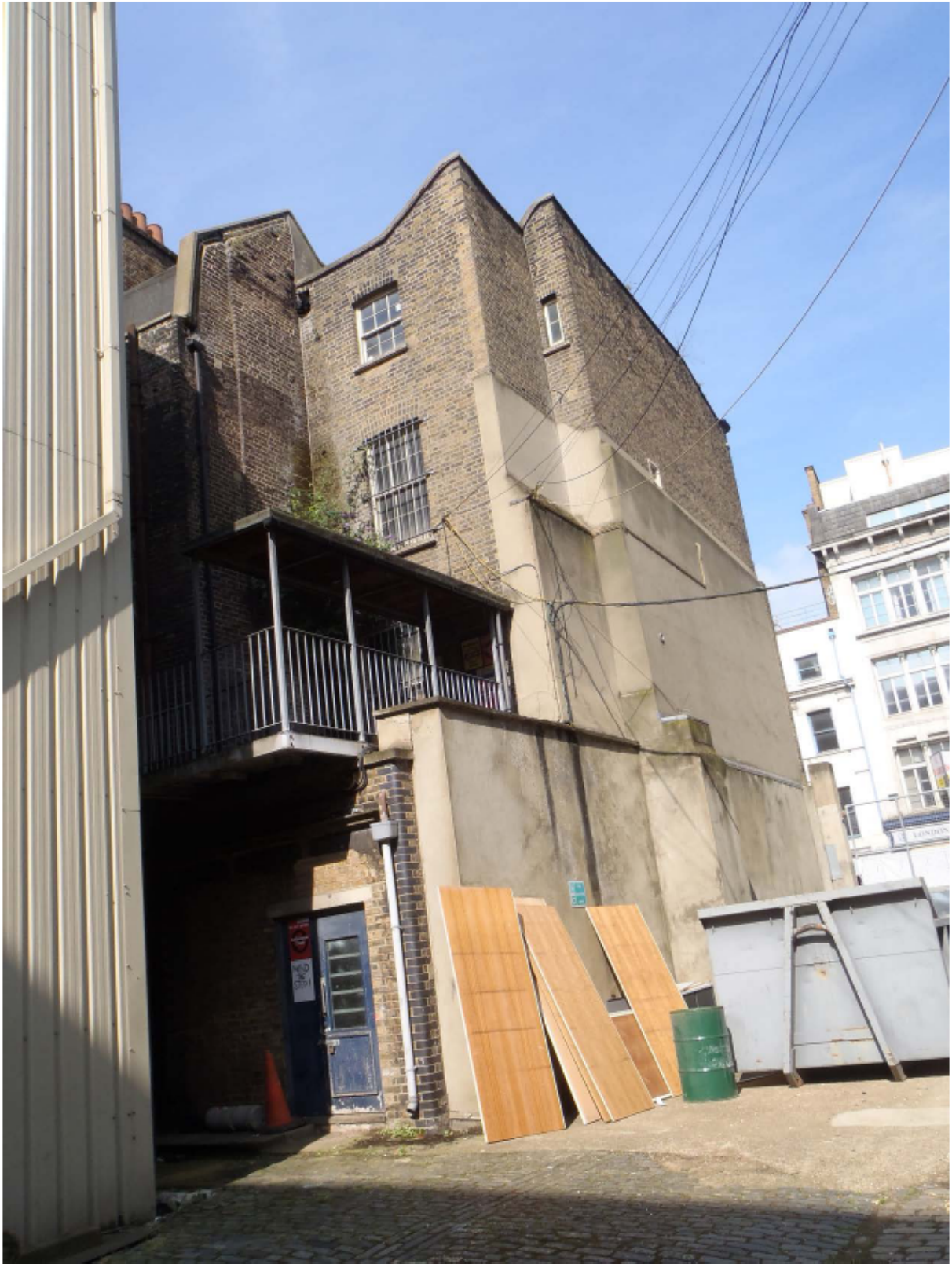
Plate 9 East (rear) and north (side) elevation of no. 141 Borough High Street, looking south-west
