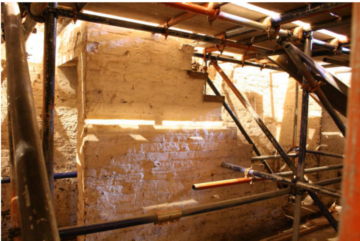
Plate 57 Flight of steps against the north wall of no. 141 Borough High Street at basement level, looking north-east
