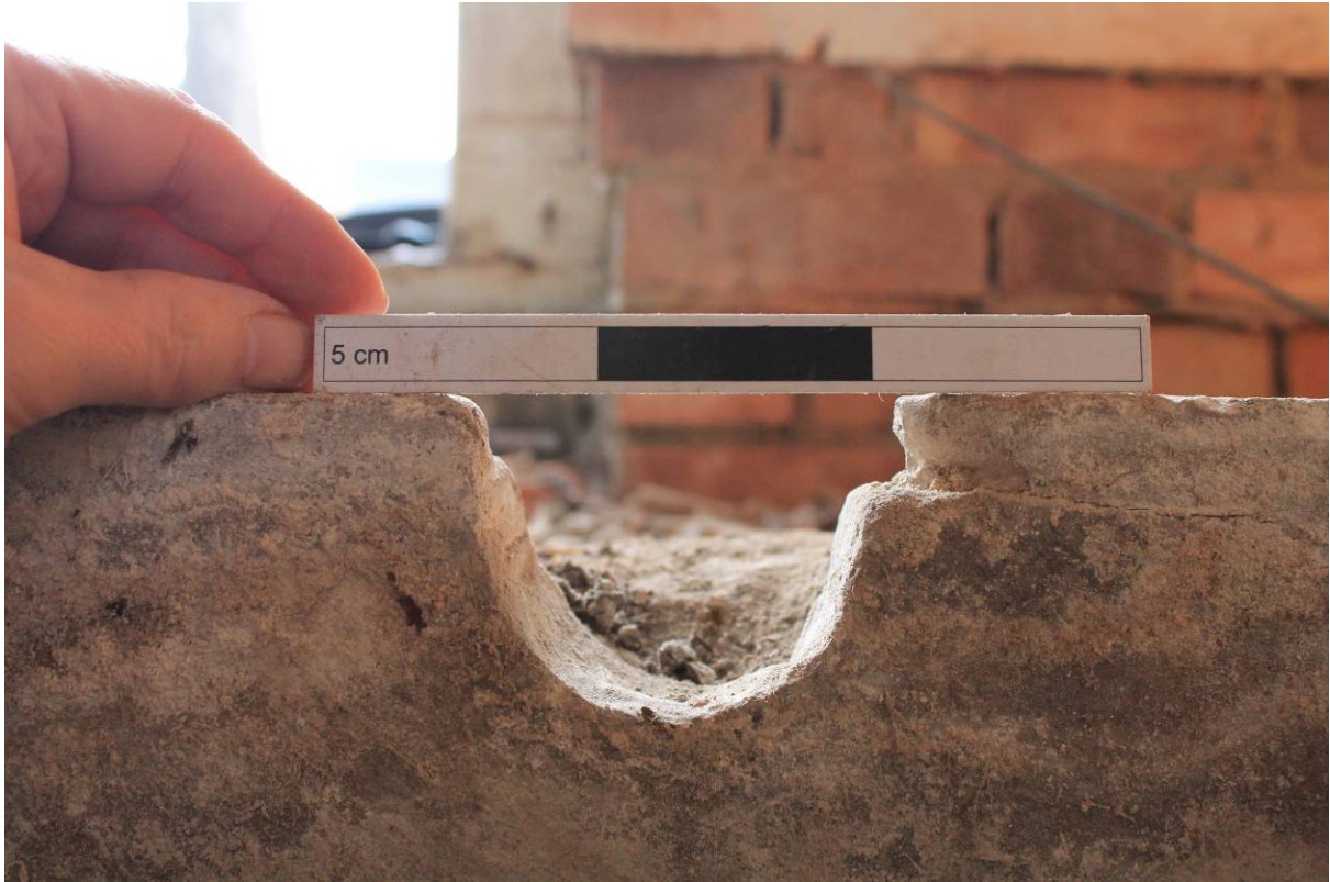
Plate 19 Notch for water spout at the south end of the east wall, looking east
