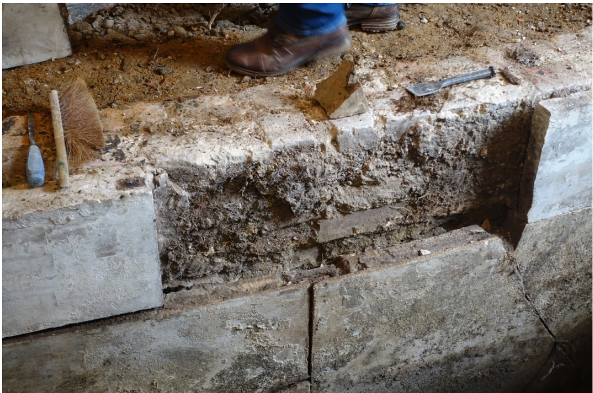
Plate 31 Recess or groove along the top of the Portland Stone slabs lining the bath and iron bridging tie that joined the slabs together, looking north
