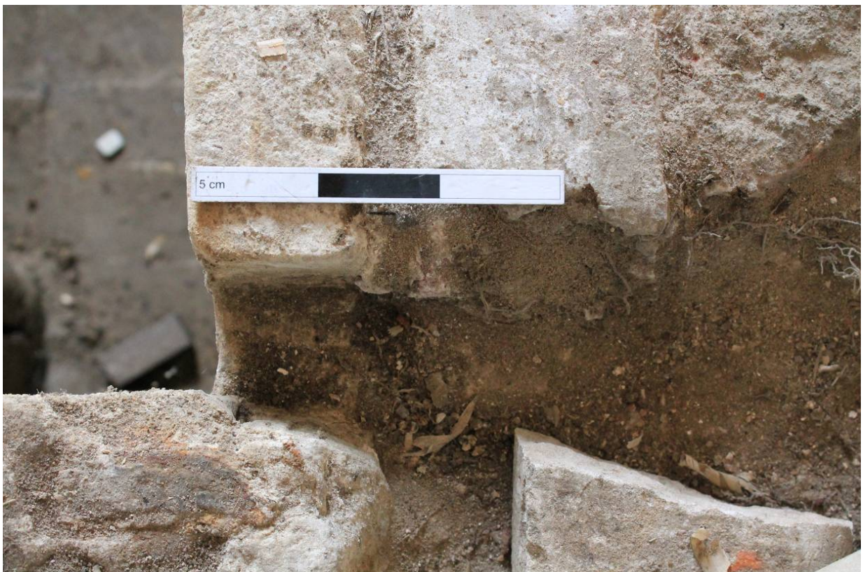
Plate 20 Notch for water spout at the west end of the south wall, looking down and east
