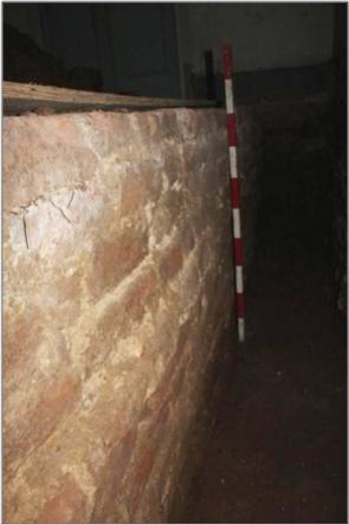
Plate 29 North side of the north wall of the bath structure, looking west
