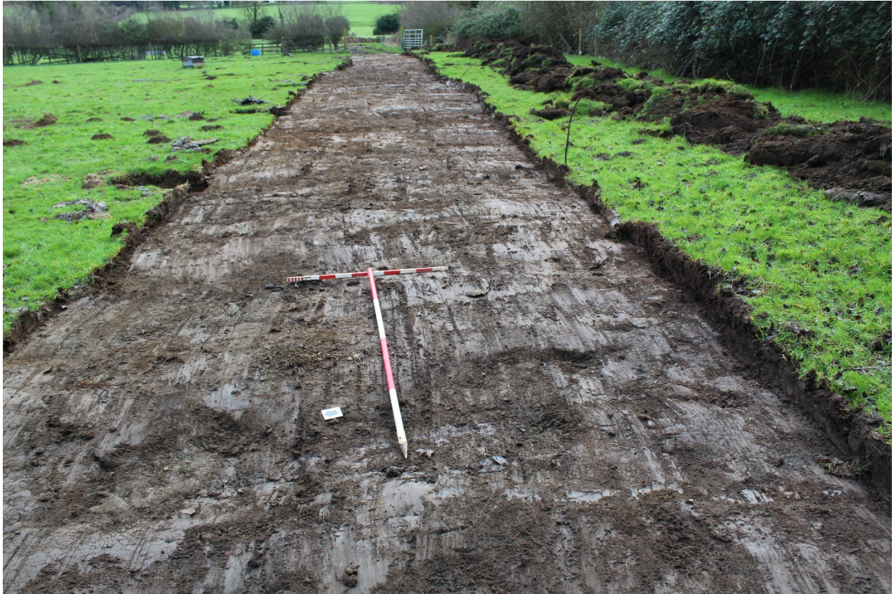
Plate 9: East-southeast facing shot of stripped road area adjacent to barn footings. Only the topsoil (context 01) has been revealed.
