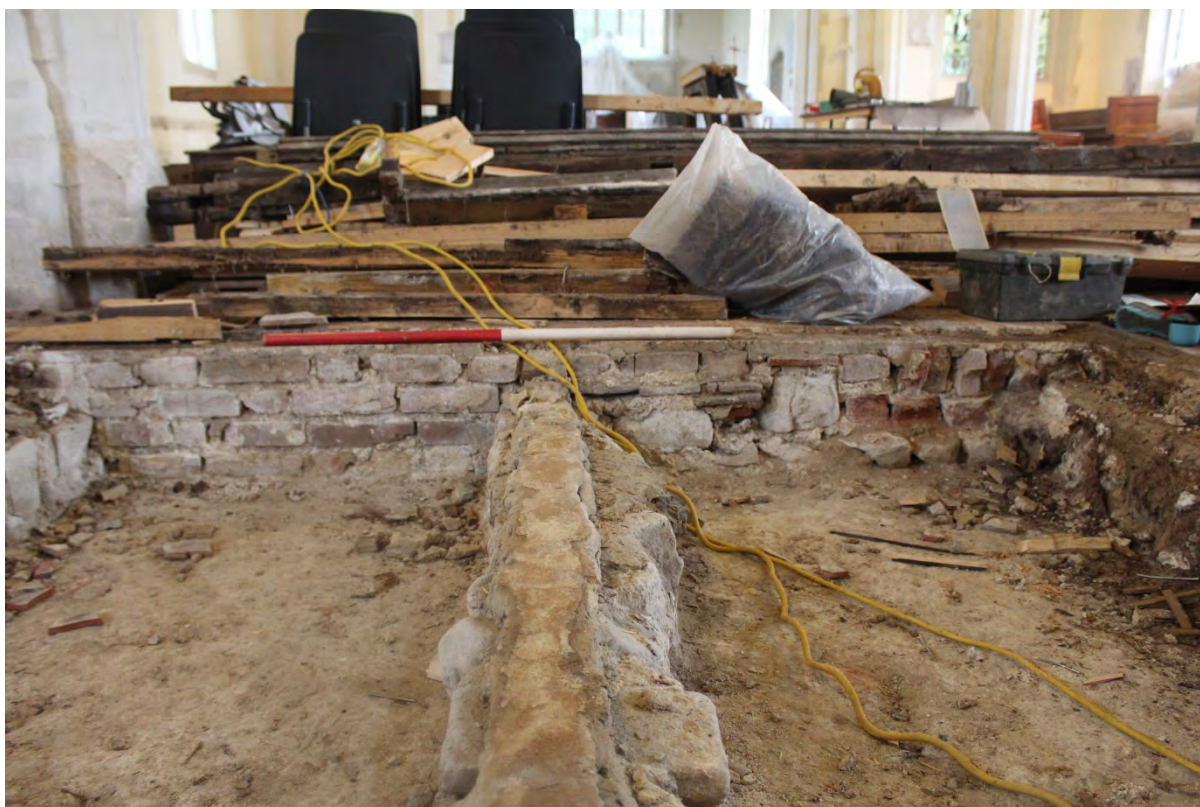
Plate 6: Area recorded following pew removal in the western end of the nave (north side of tower entrance)
