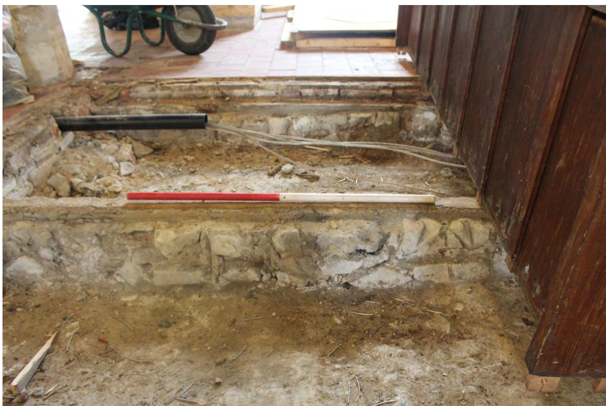
Plate 7: Area recorded following pew removal in the western end of the nave (south side of tower entrance)
