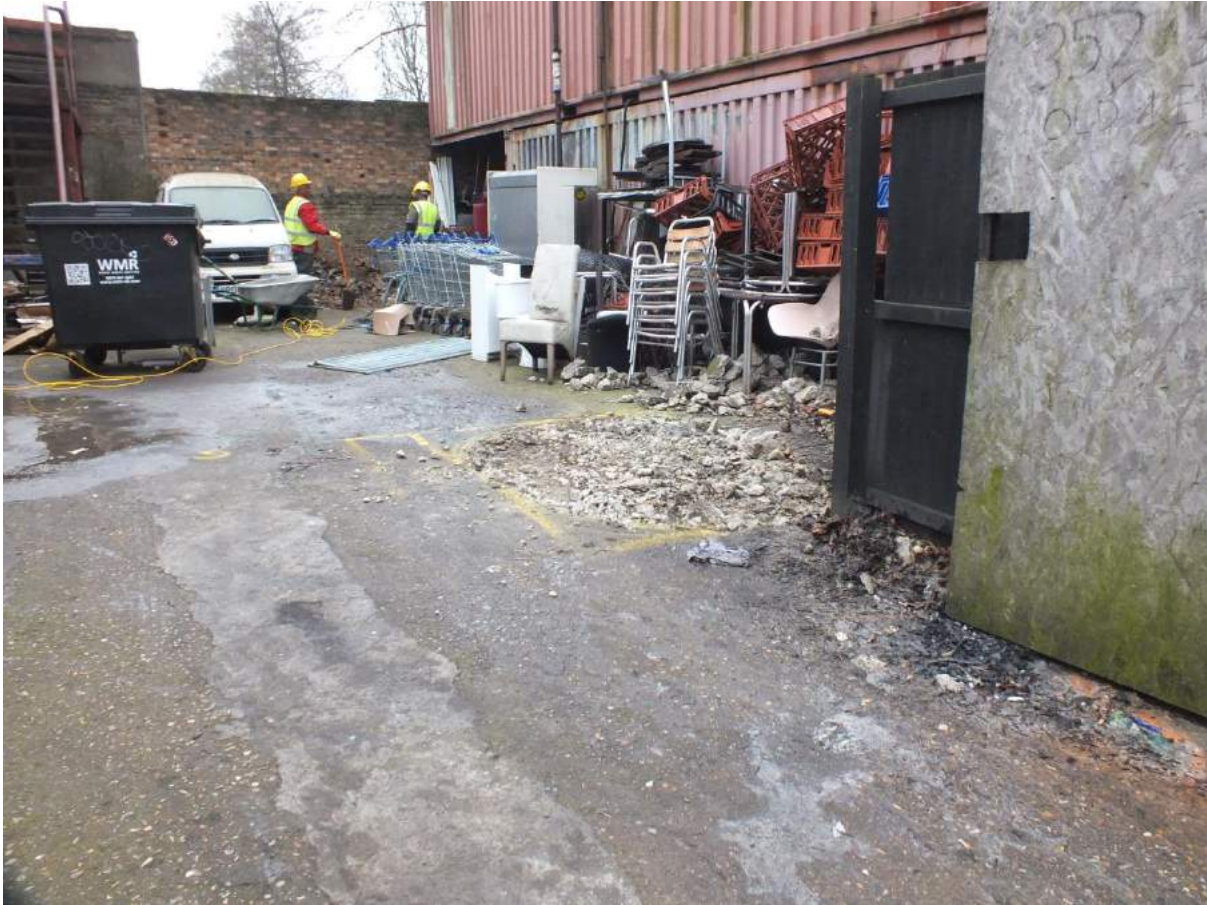
Plate 1: View of rear yard area prior to main excavation, showing hard standing level in which excavations occurred, looking south east
