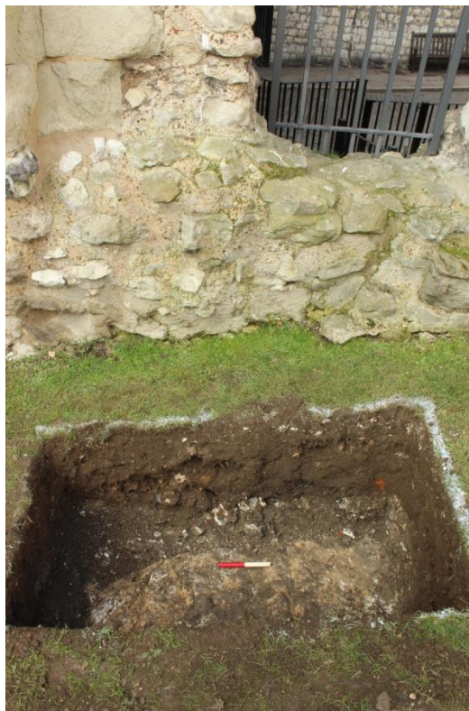
Plate 8: Tr 10B showing the trenches proximity to the Main Guard Wall, looking west
