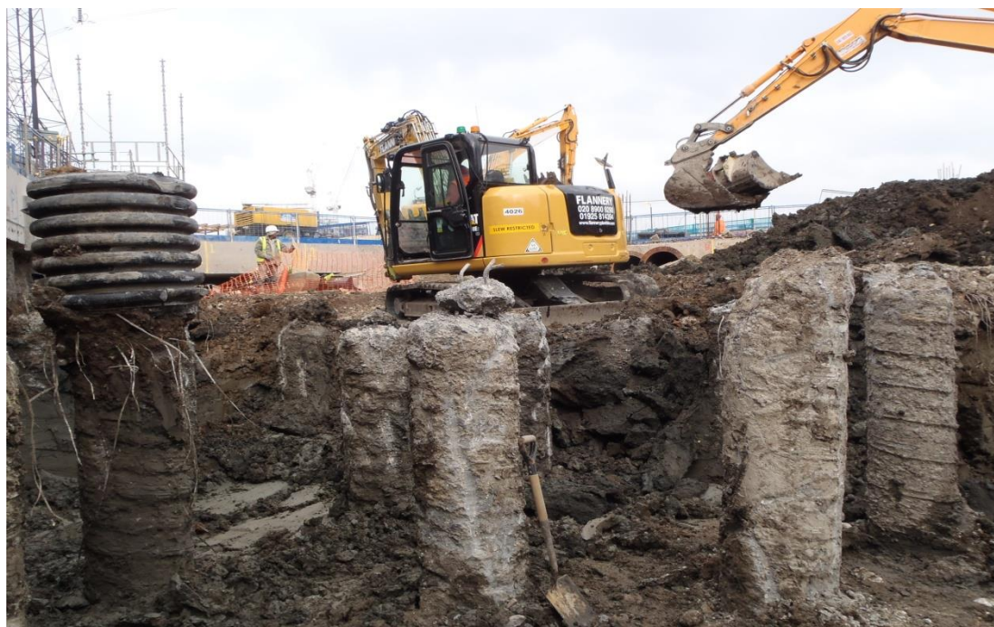
Plate 4: Site conditions: Density of piles in south-east sector (view to north west)
