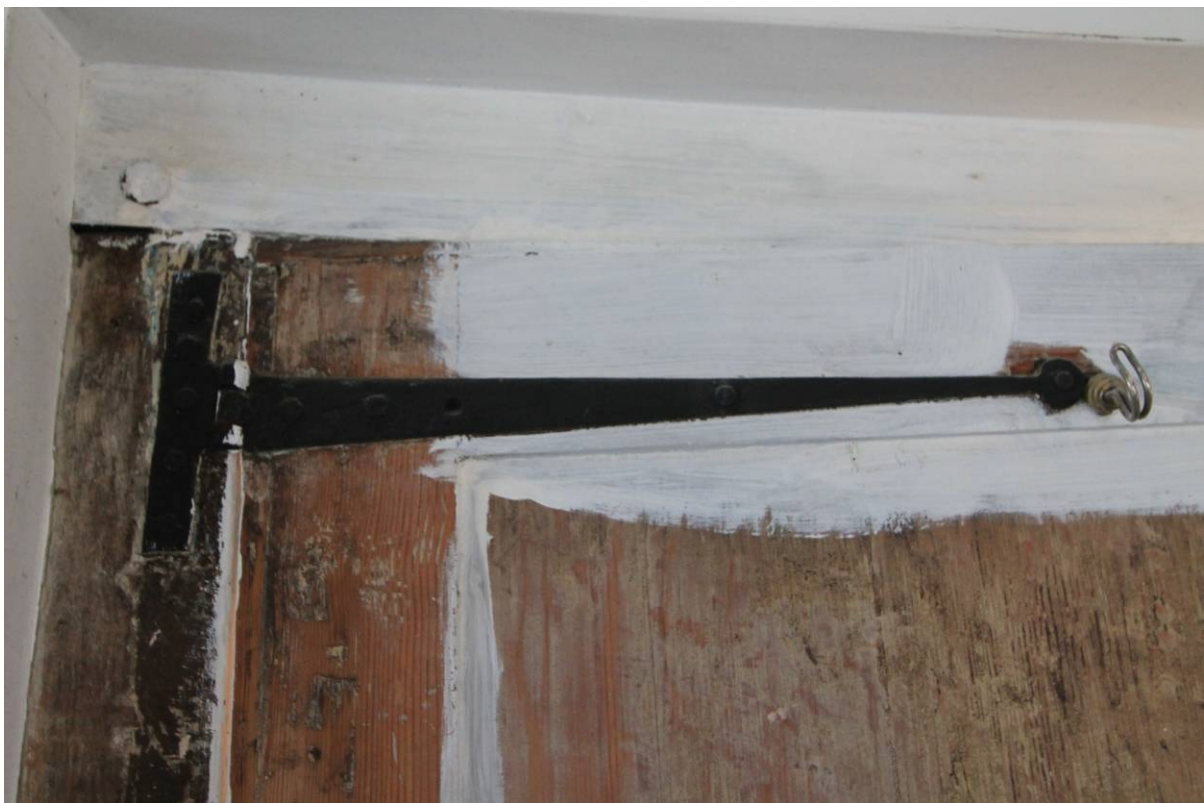
Plate 23 Eighteenth century strap hinge to door from GF1 to GF4, looking south-west
