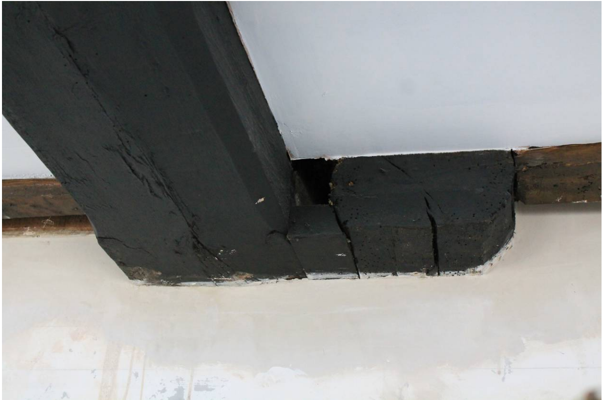
Plate 22 Simpler stops to binding joists and side by side layout of beams over axial wall in GF3, looking south-west
