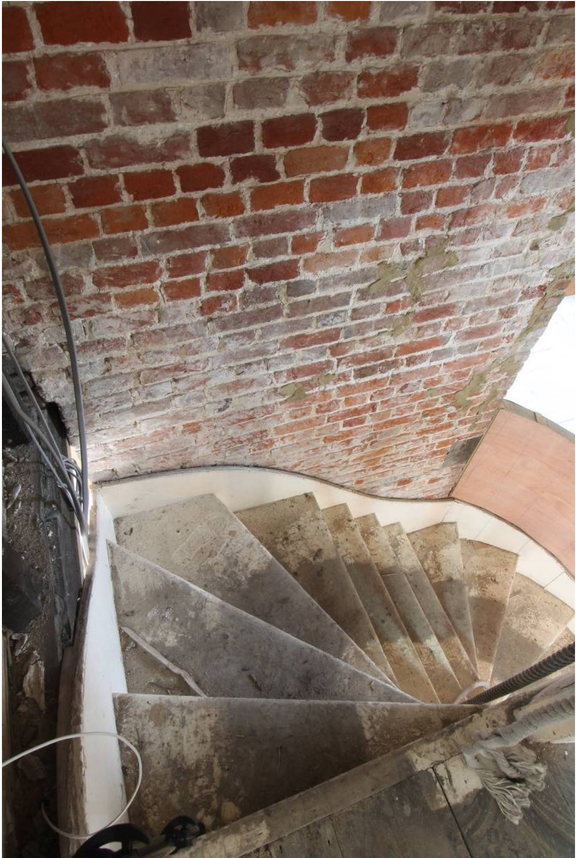
Plate 19 Winder stair, looking west down from the first floor to the ground floor
