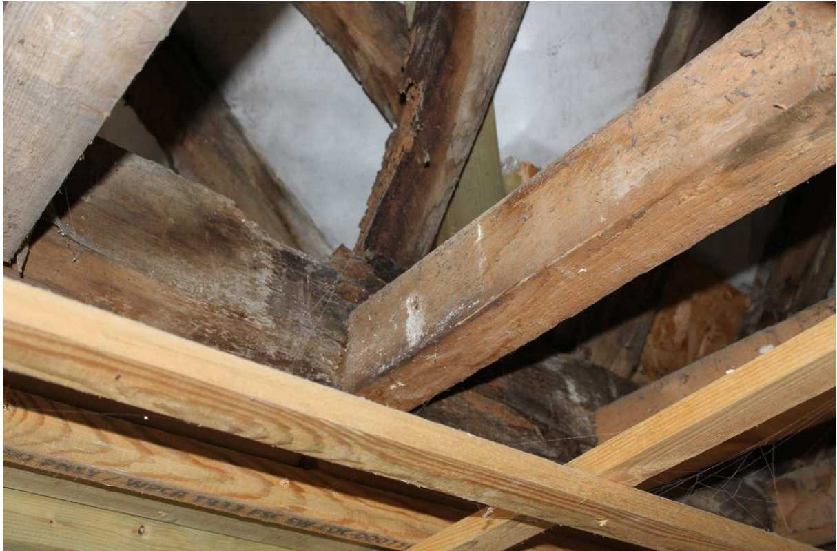
Plate 44 Decay from leaking central well, looking west
