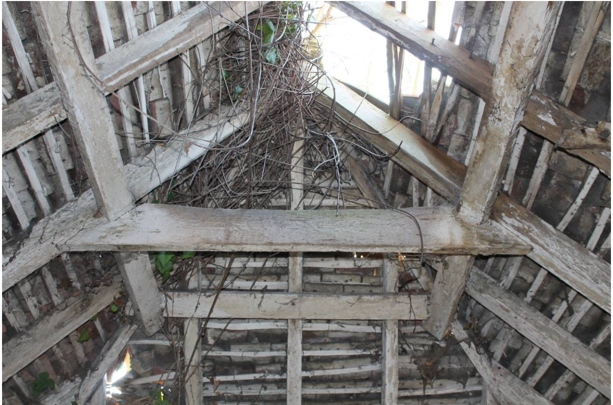
Plate 50 Clapsed side purlin roof in former farm outbuilding, looking south-west
