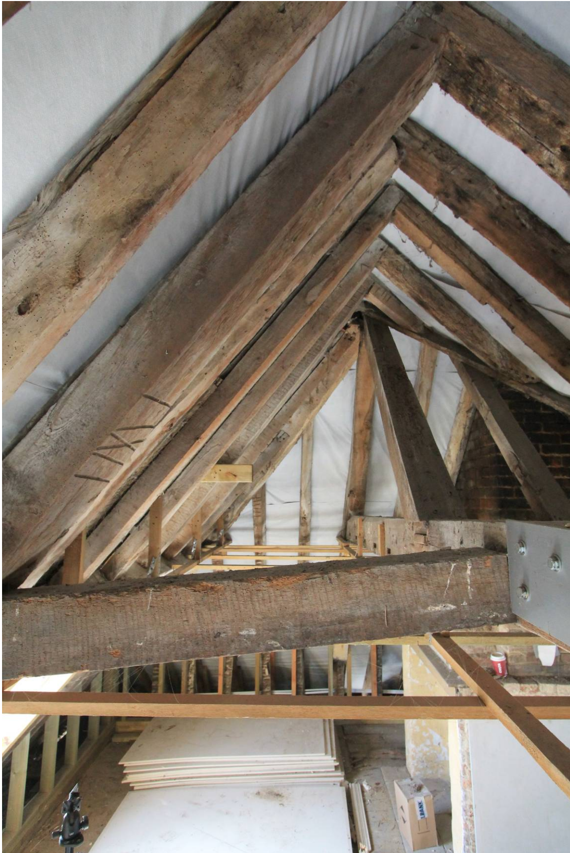
Plate 41 South-eastern roof pitch showing Baltic marks with the central well to the right, looking south-west
