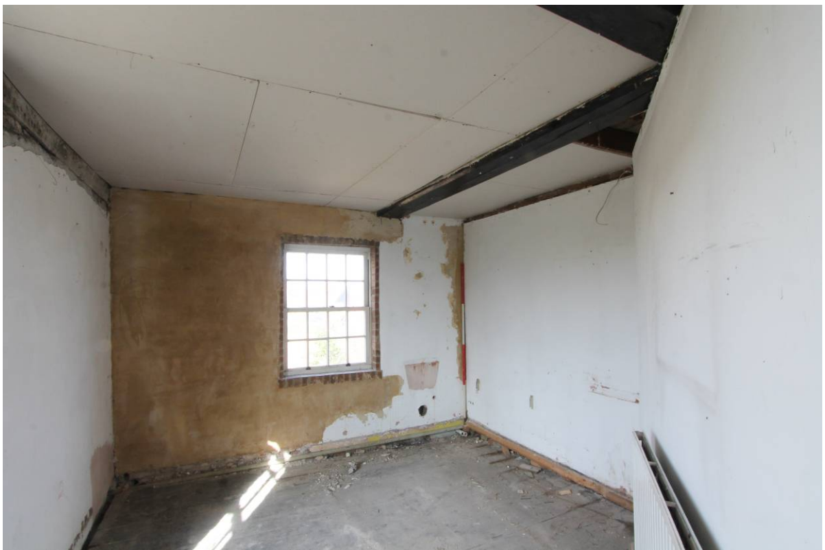
Plate 35 Former Bathroom FF5 before removal of partition (right) between Rooms FF4 and FF5, looking north
