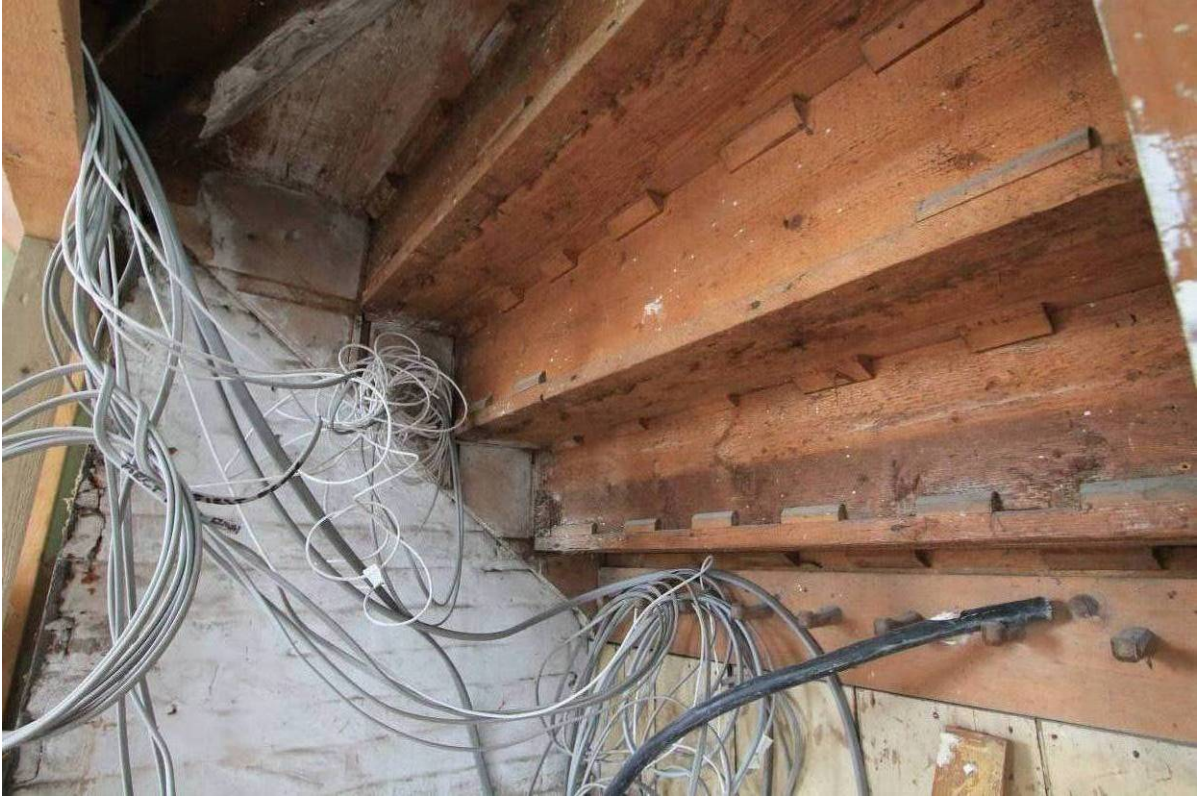
Plate 18 Detail of stair construction seen via ground floor under-stair cupboard in GF2, looking south-west
