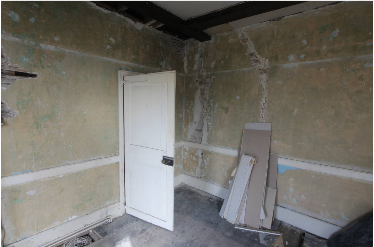
Plate 31 Eighteenth century door, dado rail and skirting boards in Room FF3, looking north
