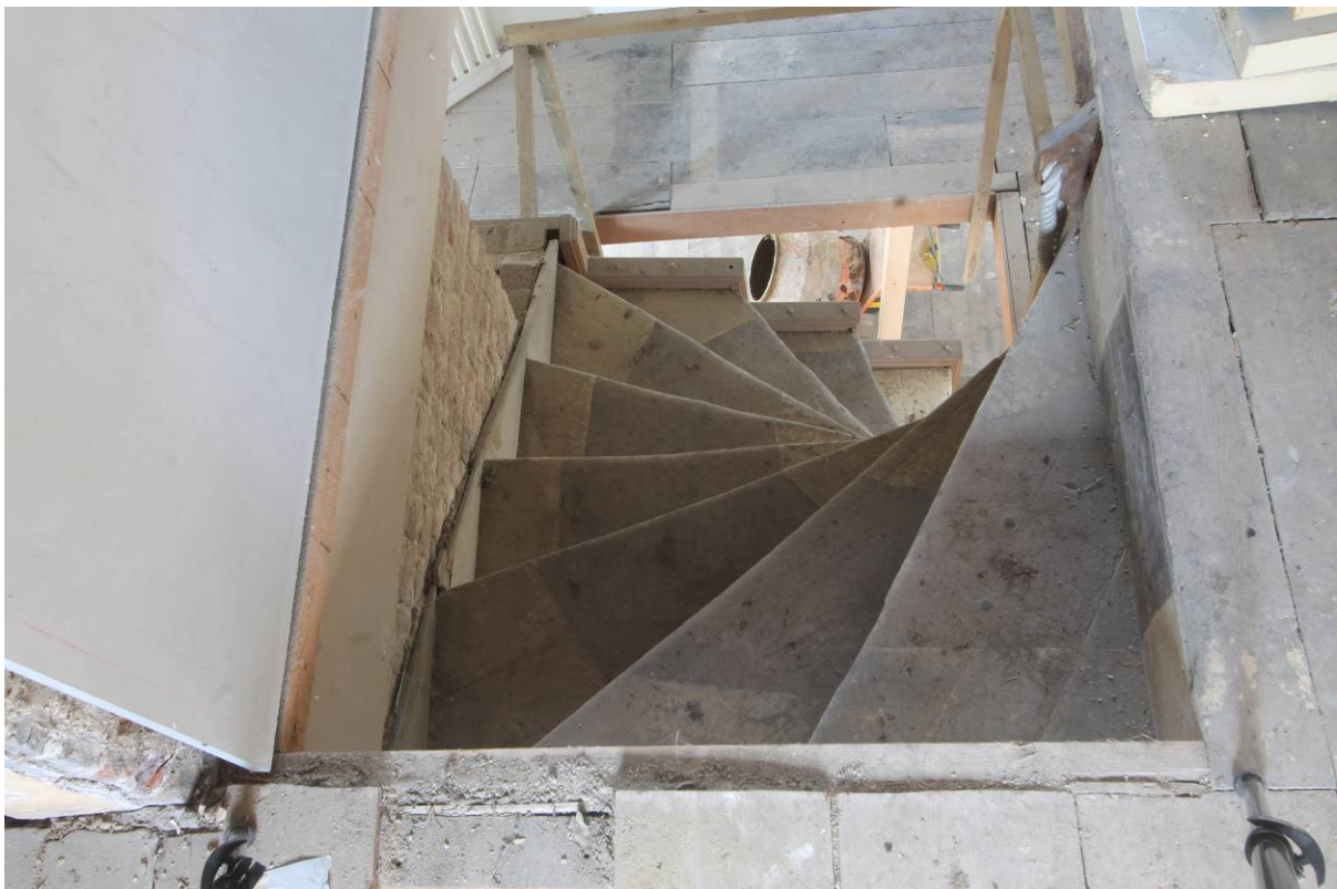
Plate 38 Winder stair, looking north-west from the attic down to the first floor
