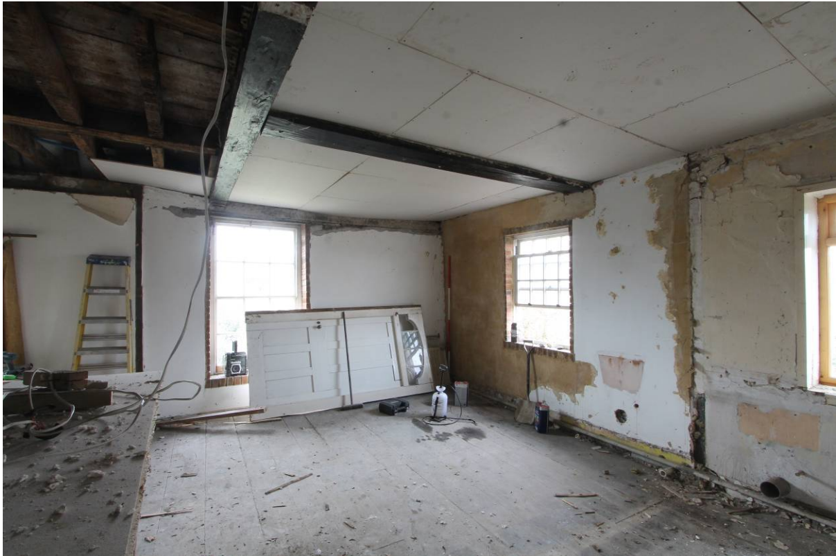
Plate 37 Rooms FF4 and FF5 after the removal of partition wall between the two rooms, looking west
