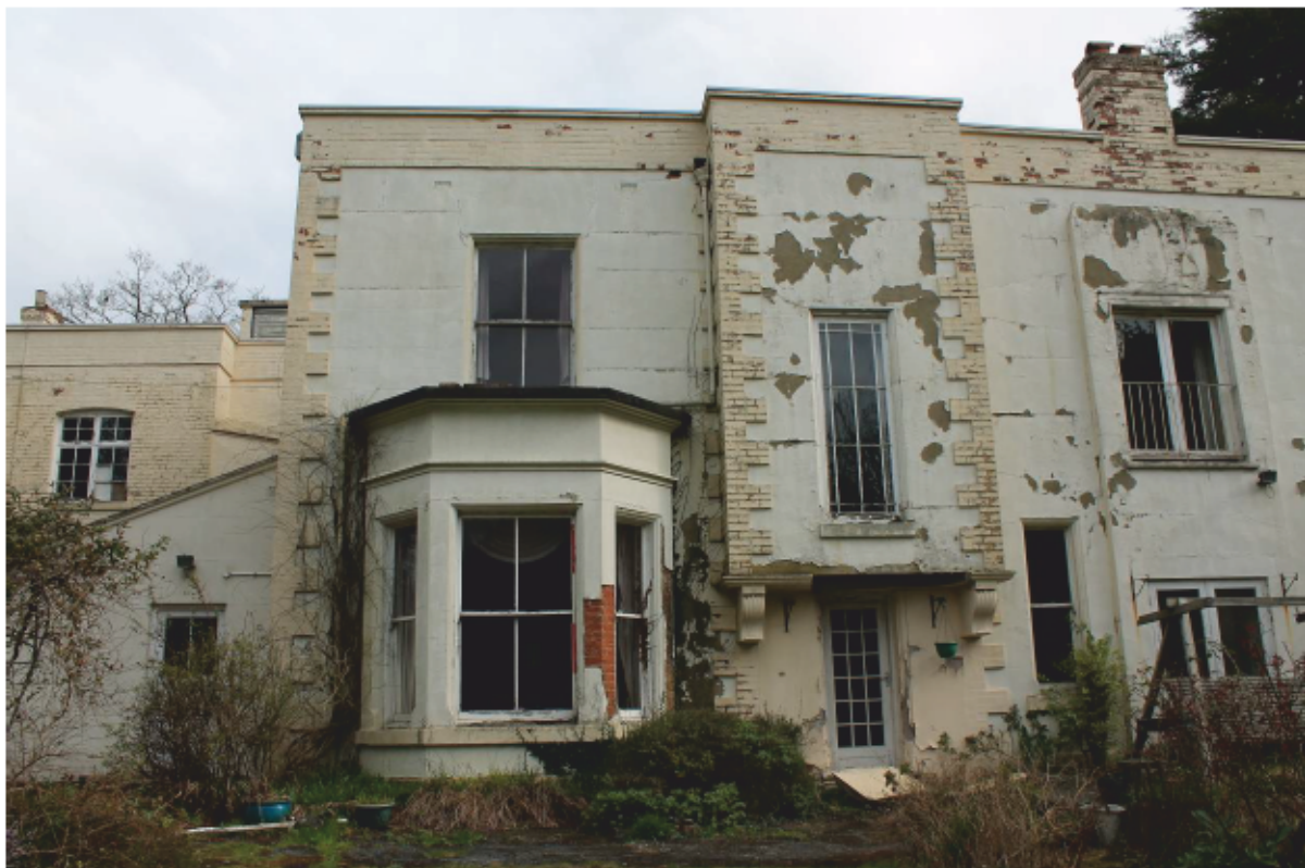
Plate 10 Canted bay window and jettied stairwell bay in southern elevation, looking north
