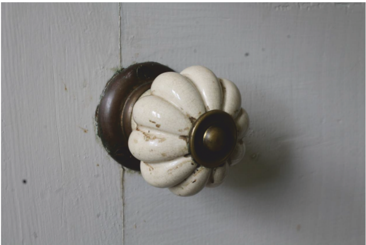
Plate 30 Detail of door handle on door from Study (GF5) to Hall (GF1), looking east
