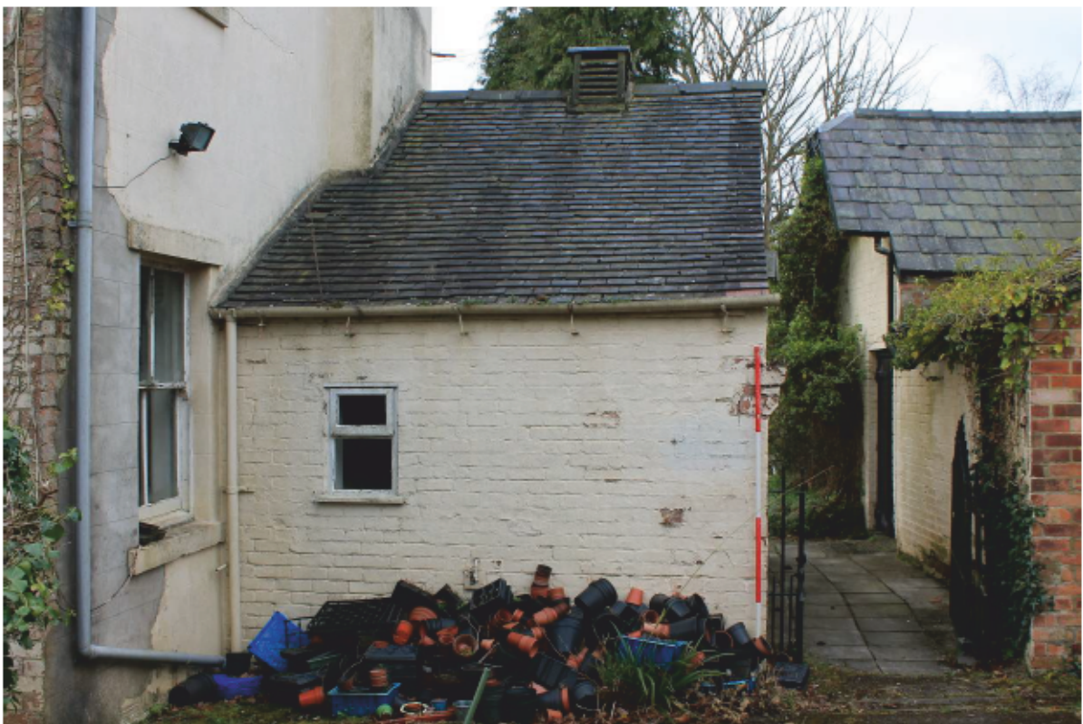
Plate 6 Former laundry (GF12) at the western end of the north elevation, looking south
