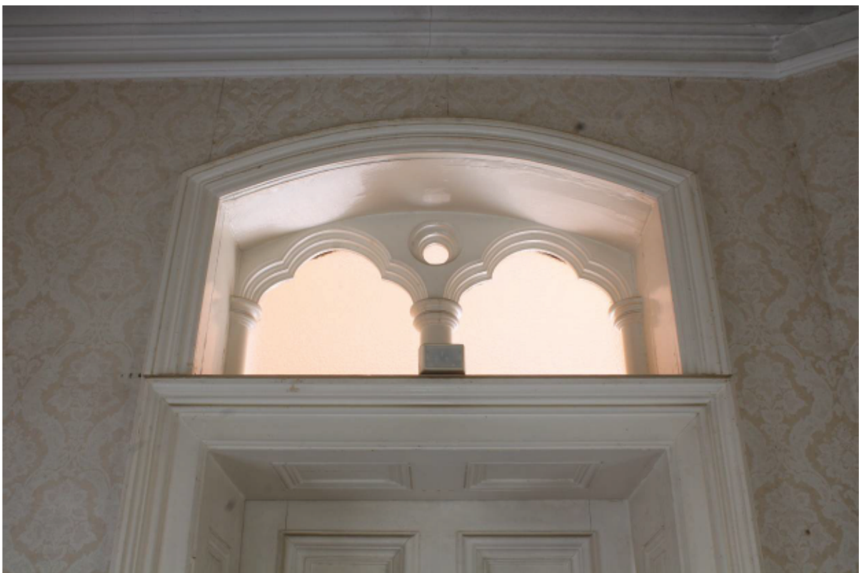
Plate 26 Decorative light above doorway from Hall (GF1) to Cloakroom/WC (GF4), looking north
