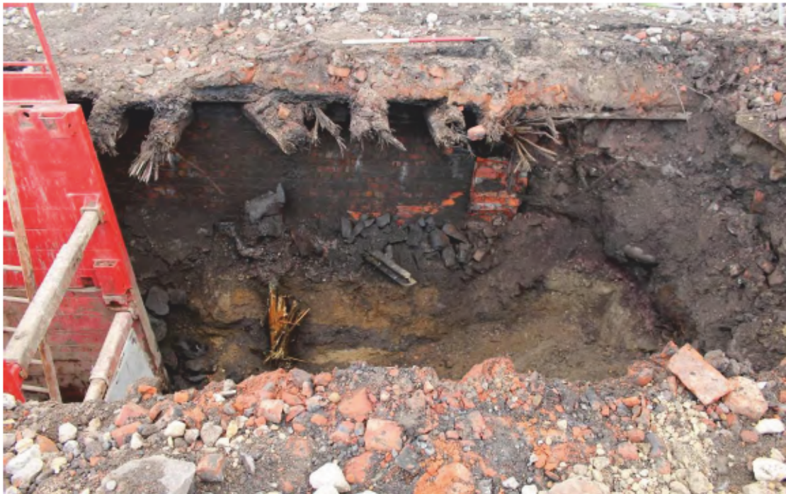
Plate 7: Trench 2, south-west facing section view of concrete floor and rails structure [263] and walls [261] and [264] and rails with timbers [289] and [259] (scale 1m)
