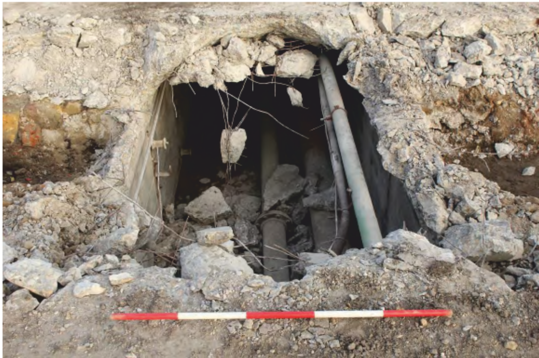
Plate 14: North-east facing view of concrete pipe housing in the northern extent of Trench 3 (scale 1m)
