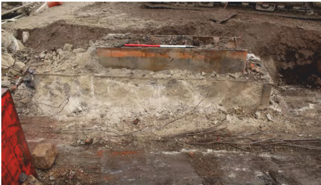
Plate 10: North-west facing view of 20th-century building footing structure [290] in the northern section of Trench 2 (scale 1m)
