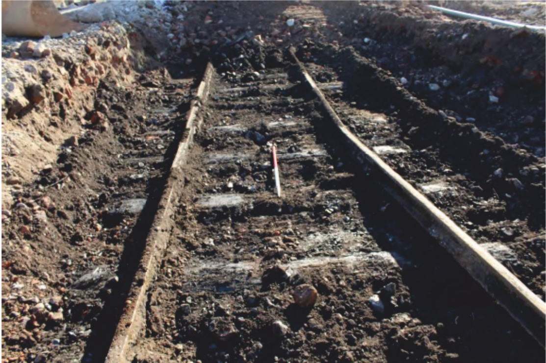
Plate 3: South-east facing view of timber sleepers [124] and vignole rails [125] in central portion of Trench 1 (scale 1m)
