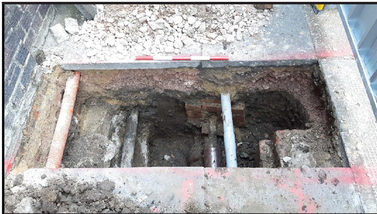
PLATE 8. SOUTH FACING SHOT OF TP8, SECTION 11; THIS SHOWS THE LARGE AMOUNTS OF TRUNCATION WITHIN THIS TRENCH. WHAT CAN BE SEEN IS THE DARK BROWN POST-MEDIEVAL DUMPING OF [29] LEFT AND RIGHT [30] OF THE MANHOLE.
