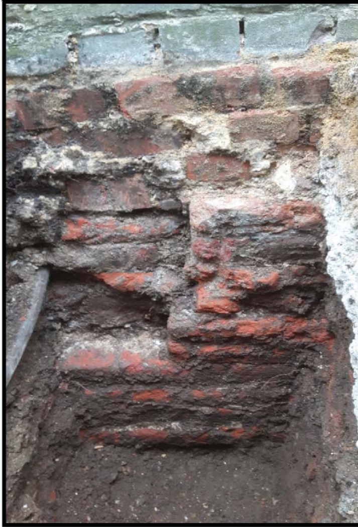
PLATE 12. NORTHEAST FACING SECTION OF WALL [13] WHICH HAS BEEN USED AS A FOUNDATION FOR THE MODERN WALL ABOVE.
