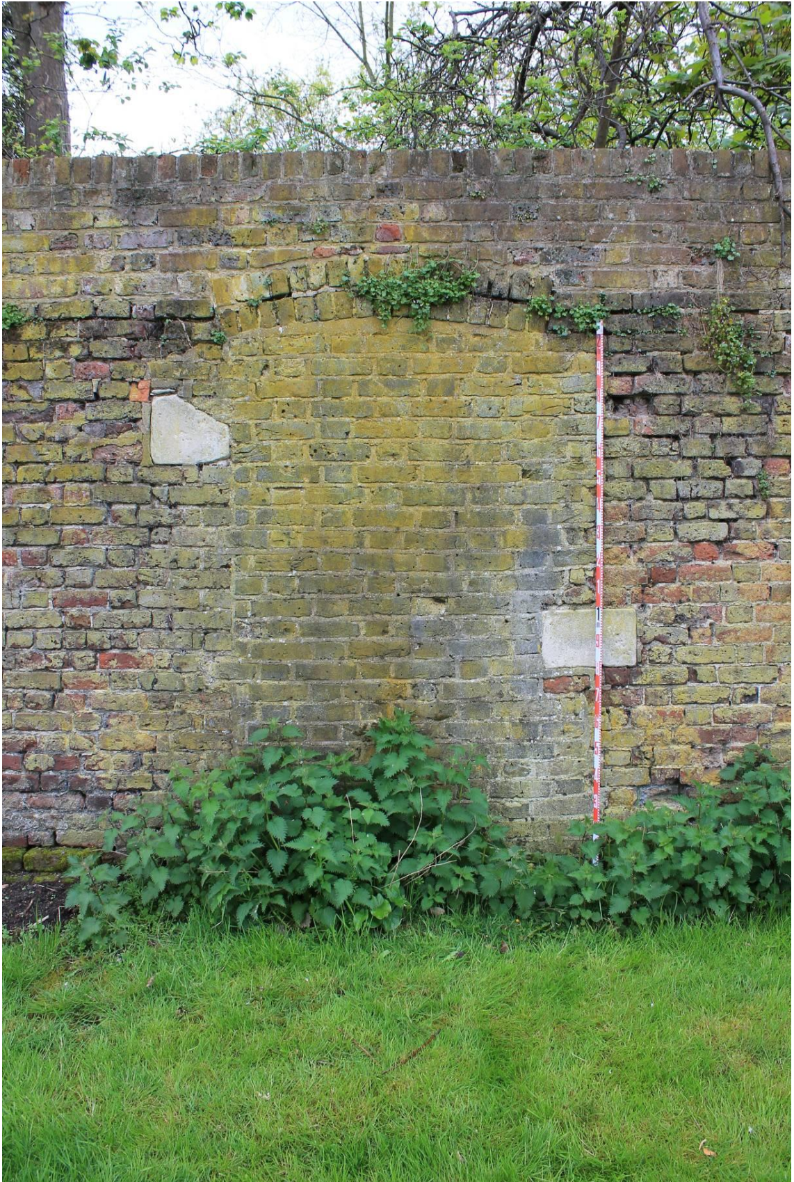
Plate 2 Blocked door opening in Southern Garden Wall (north side)
