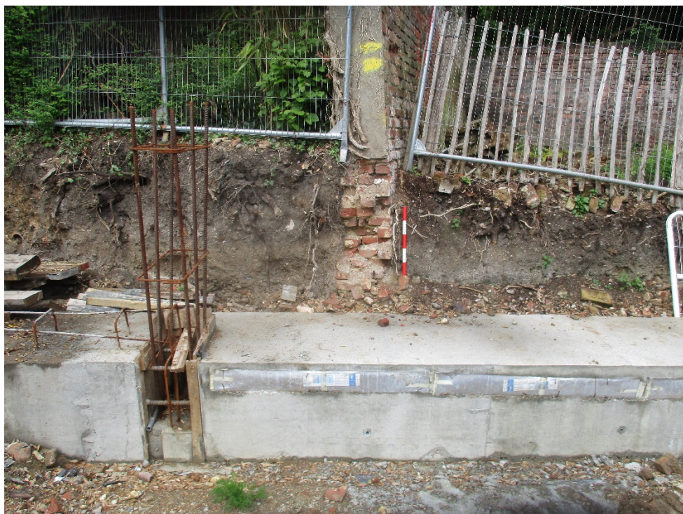
Plate 5. West facing shot of listed structure on neighbouring property, abutting the edge of the development. Scale 0.5m
