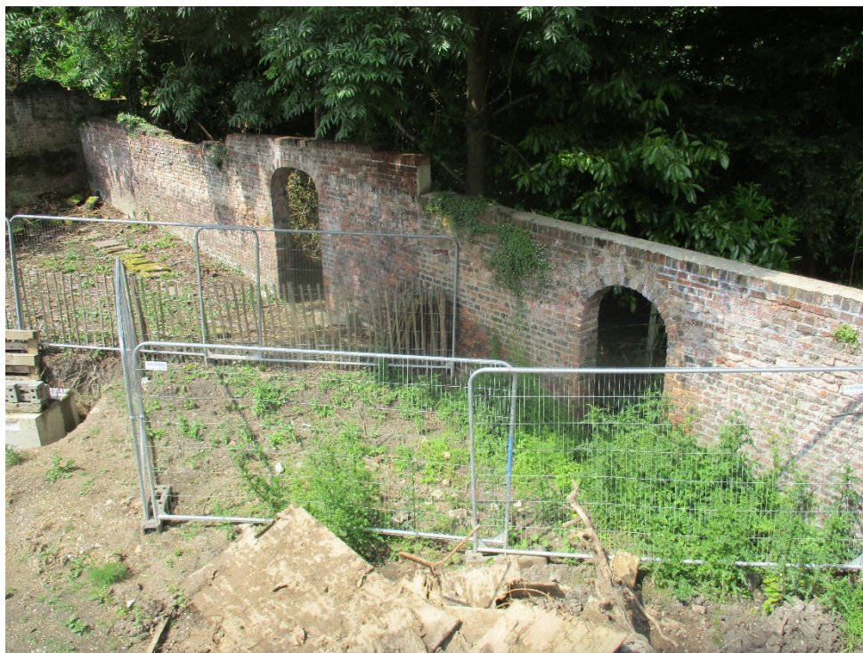
Plate 4. North West facing shot of listed structure bisecting both the site and the neighbouring property.
