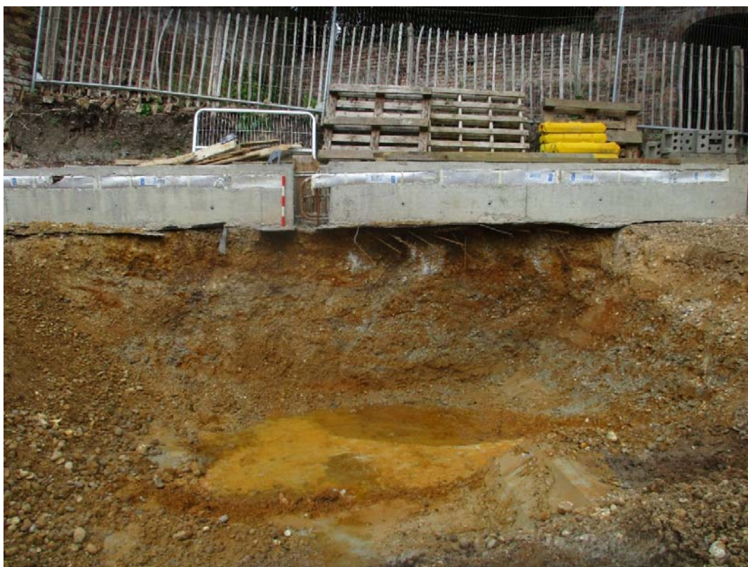
Plate 2. West facing shot of excavations, showing basement pile wall, sands & gravels and underlying clays. Scale 0.5m in length.
