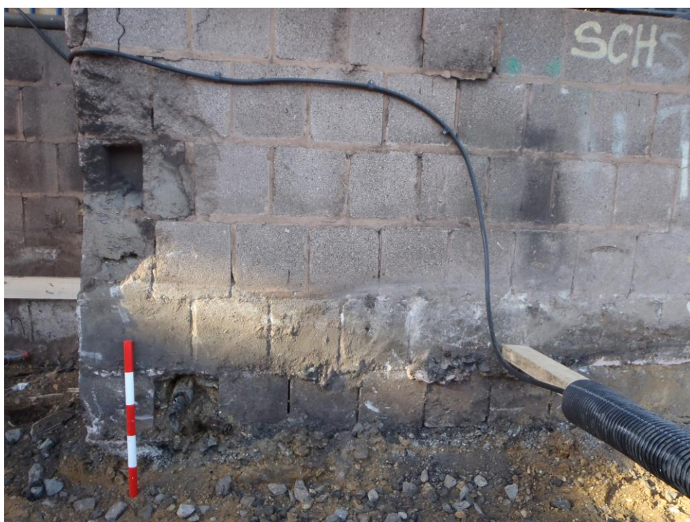
Plate 3: South-west view of north-west to south-east running wall which supports Platform 5's walkway [3]
