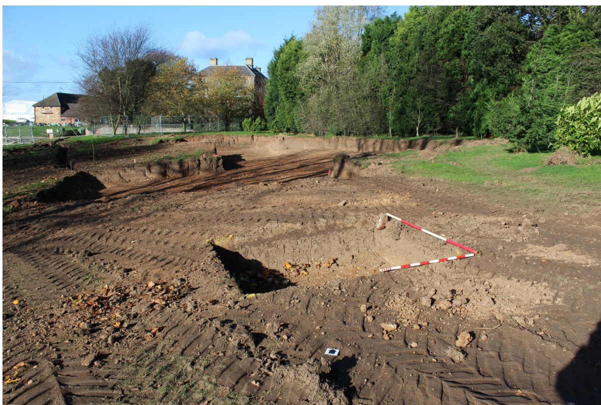
Plate 2: North-northwest facing shot of building footprint and excavated trench for water tank.
