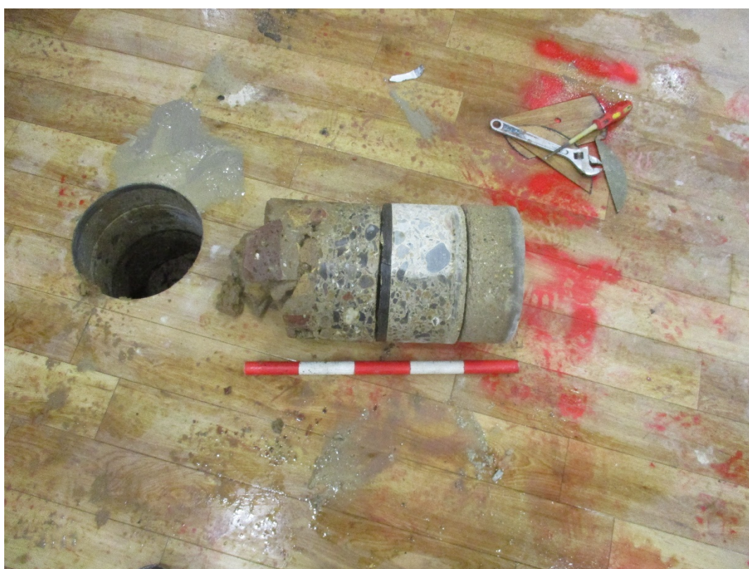
Plate 2. East facing shot of WS01, showing concrete core. Scale 0.5m in length.
