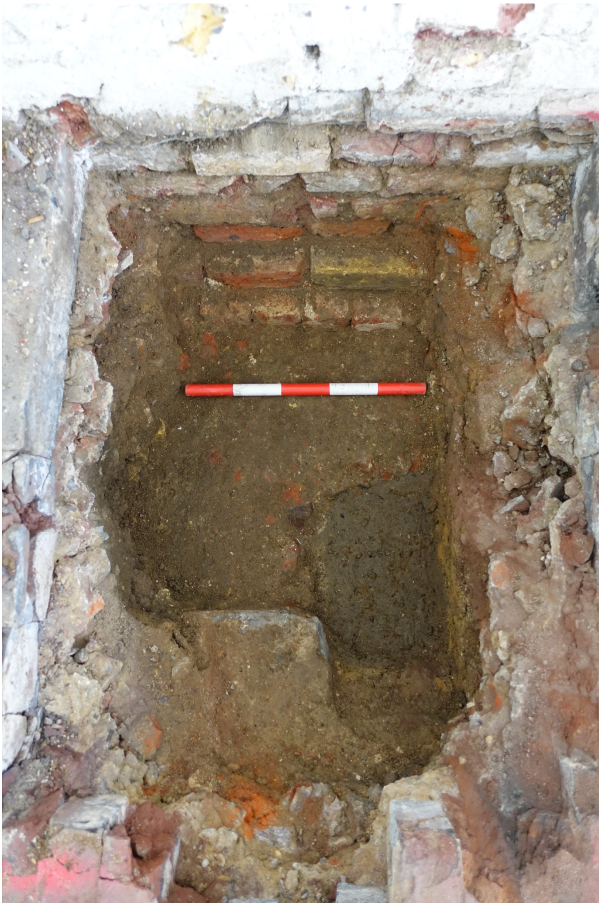
Plate 8: Base of Test Pit 3, showing [3] and current wall foundation (0.5m scale, looking east)
