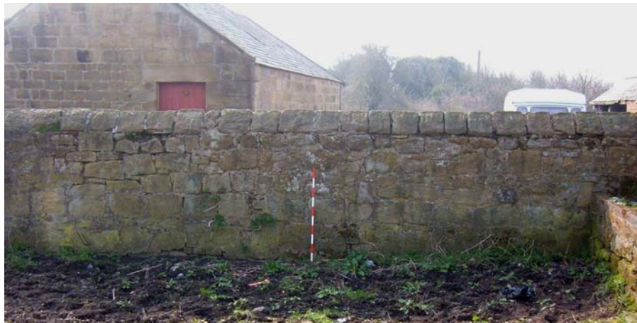
Plate 18. Fold yard, south wall – west part, interior, from the north ( 1m scale ).
