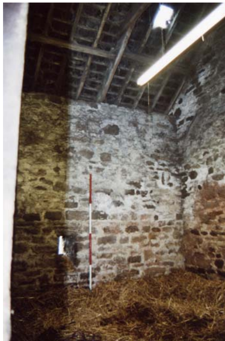
Plate 64. Threshing barn (ground floor – west part), interior, south wall, from the north-east (2m scale).
