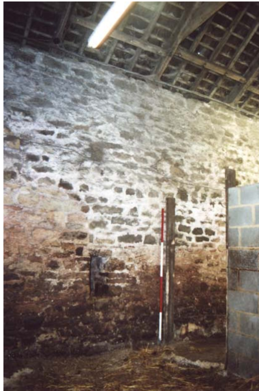
Plate 65. Threshing barn (ground floor – west part), interior, north wall, from the south-west (2m scale).
