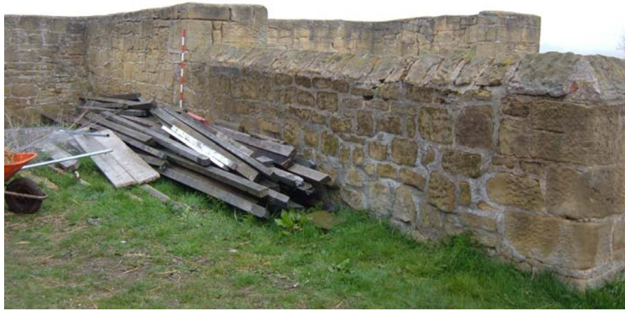
Plate 8. Former building, central and east bays, south elevation and fold yard, west wall, exterior, from the south-west ( 2m scale ).
