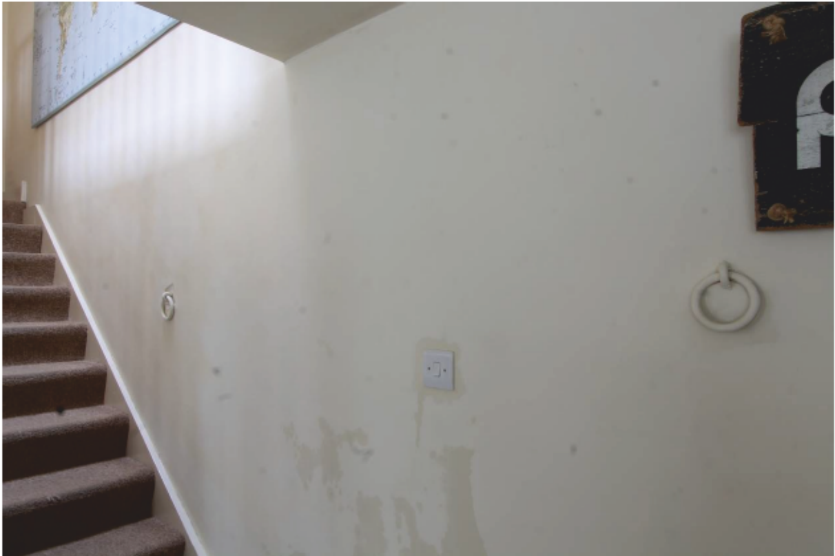
Plate 27 Extant Tethering Rings on North Wall of Ground Floor Room 3.1 in Unit 3 looking north-west
