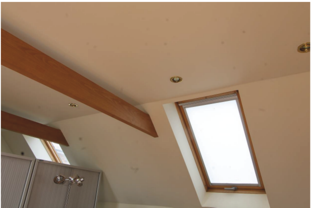
Plate 24 Inserted Velux windows and oak collars in first floor room 2.4 in Unit 2 looking south-west
