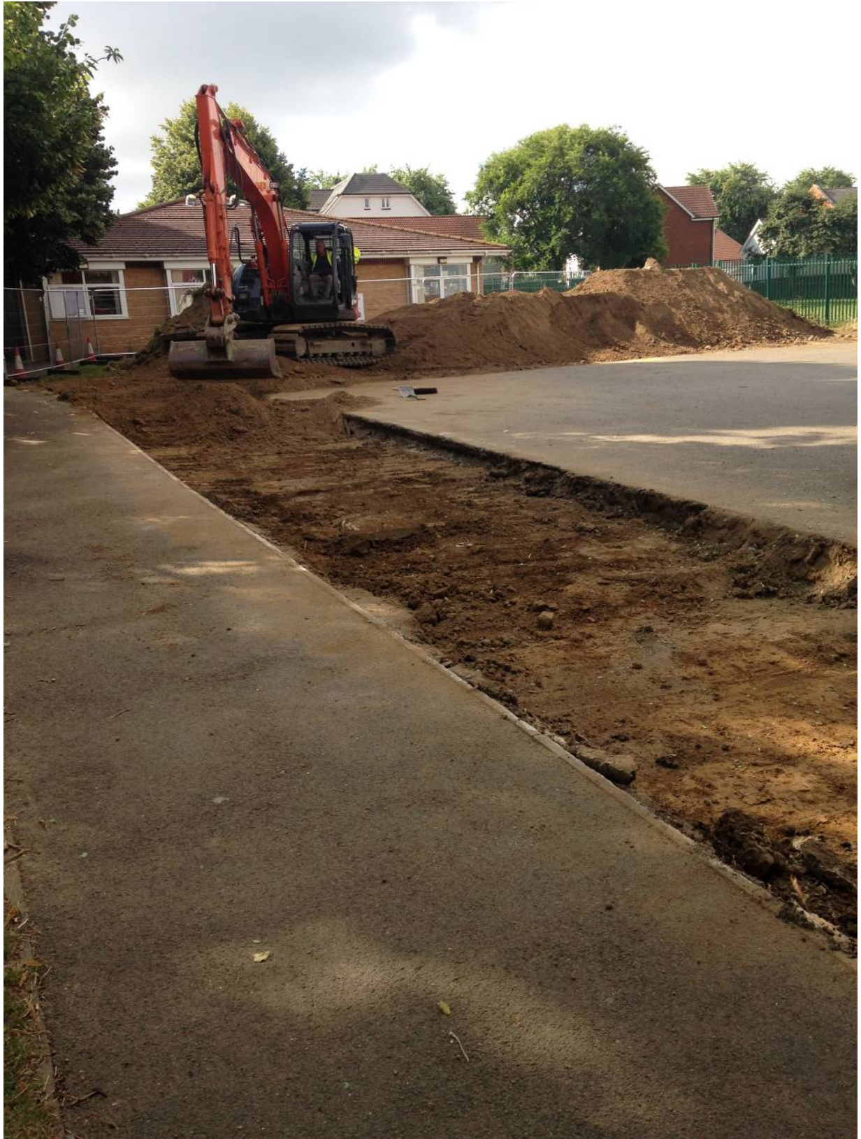
Plate 3 East side of Watching Brief area looking south towards South Borough Primary School
