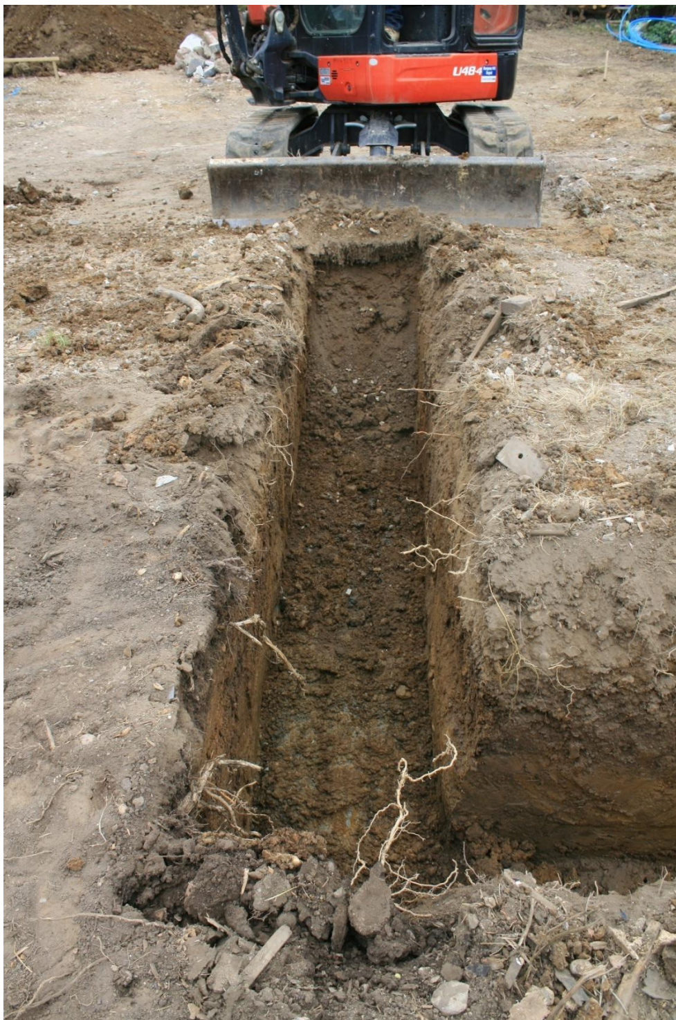
Plate 3: Excavation shot showing one trench run in House 1 (trench 1), looking southwest, (KBCE16 (13))
