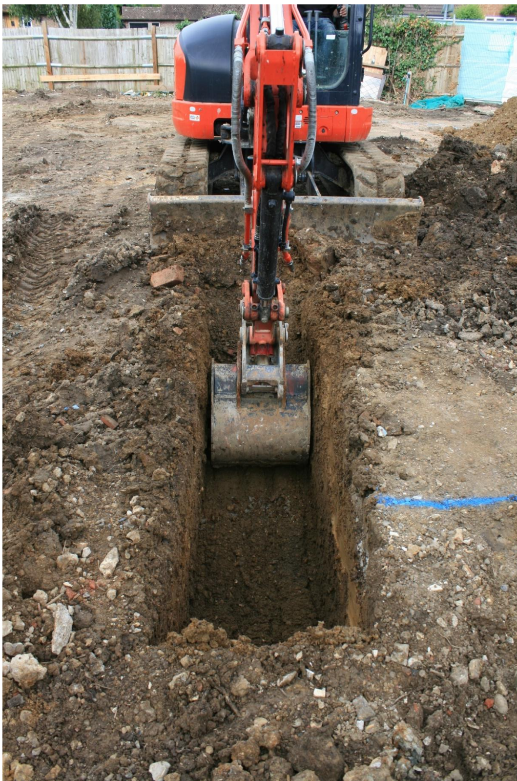
Plate 4: Mid excavation shot of one trench run in House 2 (trench 2), looking west, (KBCE16 (24))
