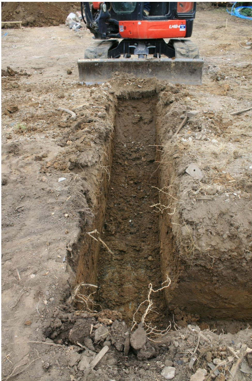
Plate 3: Excavation shot showing one trench run in House 1 (trench 1), looking southwest, (KBCE16 (13))
