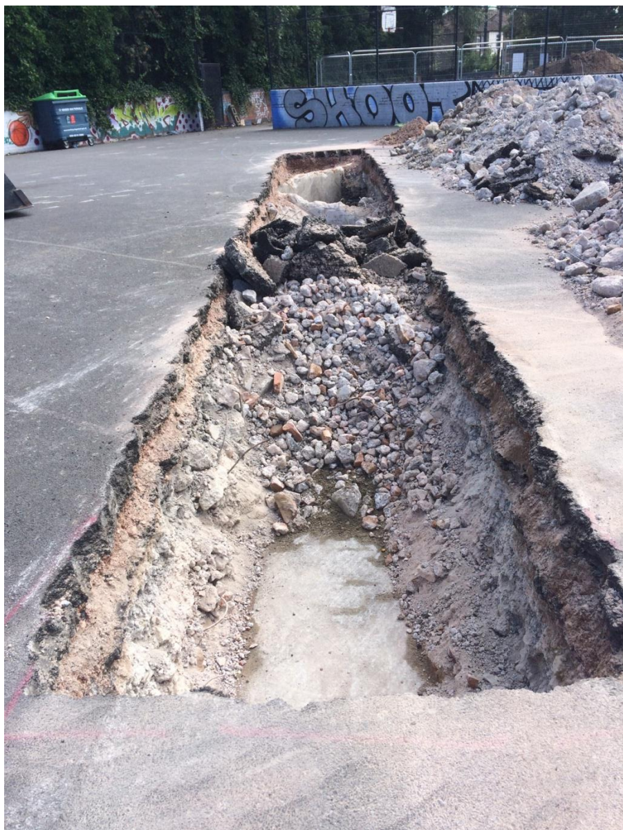
Plate 2: Trench 2, looking south east showing modern reinforced concrete floor slab and walls.
