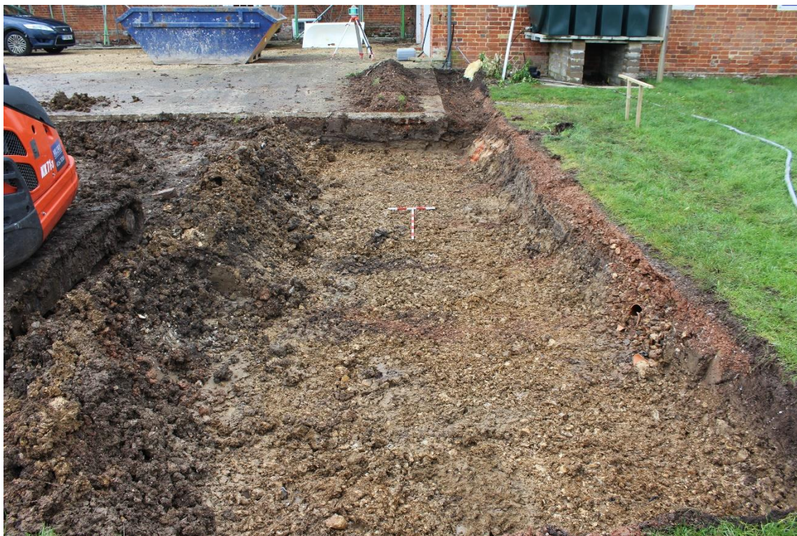
Plate 1 View to the west of Area A, showing concrete slab and modern overburden
