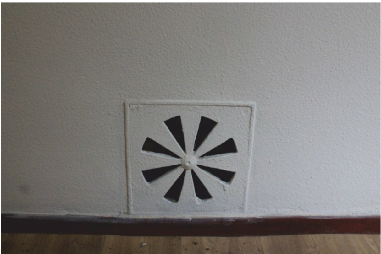
Plate 35 Cast-iron ventilator within Cell Block Area
