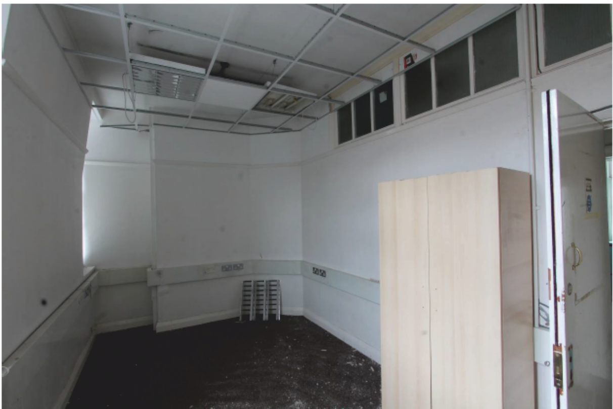
Plate 45 Office SF5 showing corbelling of wall
