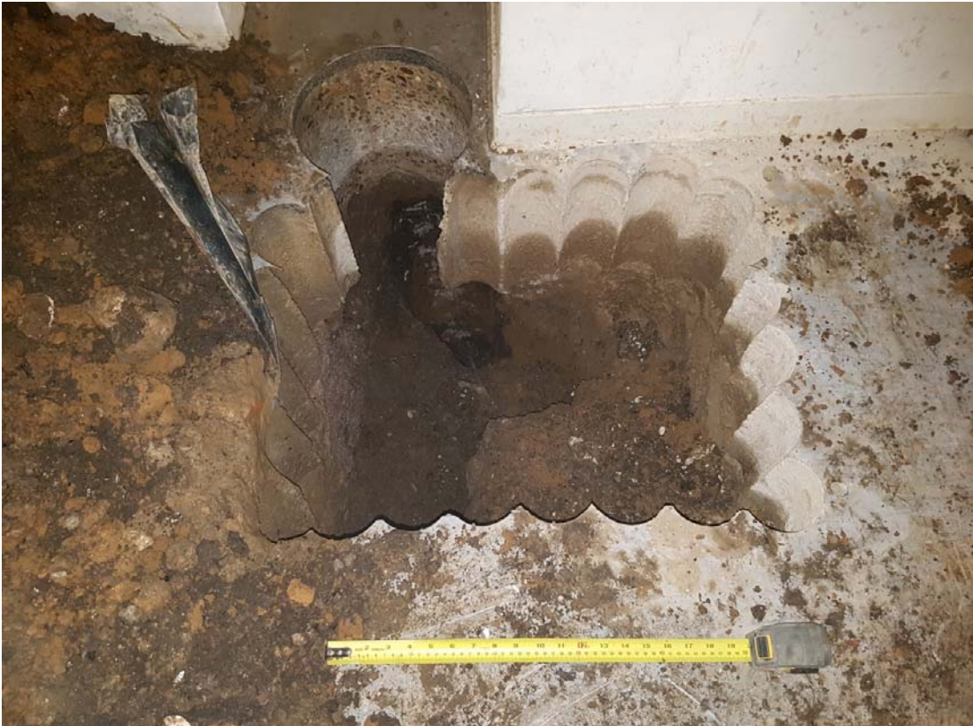
Test Pit 2 facing east. Thin strip of wall exposed below party wall (Top of photograph below large circular core through basement slab)
