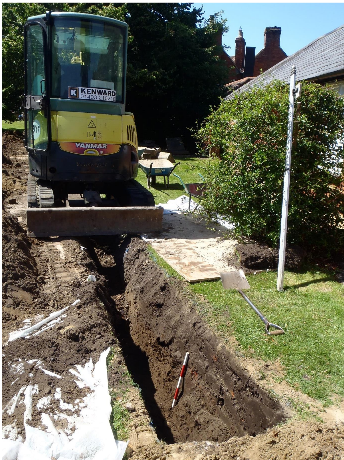
Plate 3 West view of north-eastern end of monitored area, showing general excavation area (Figure 2)
