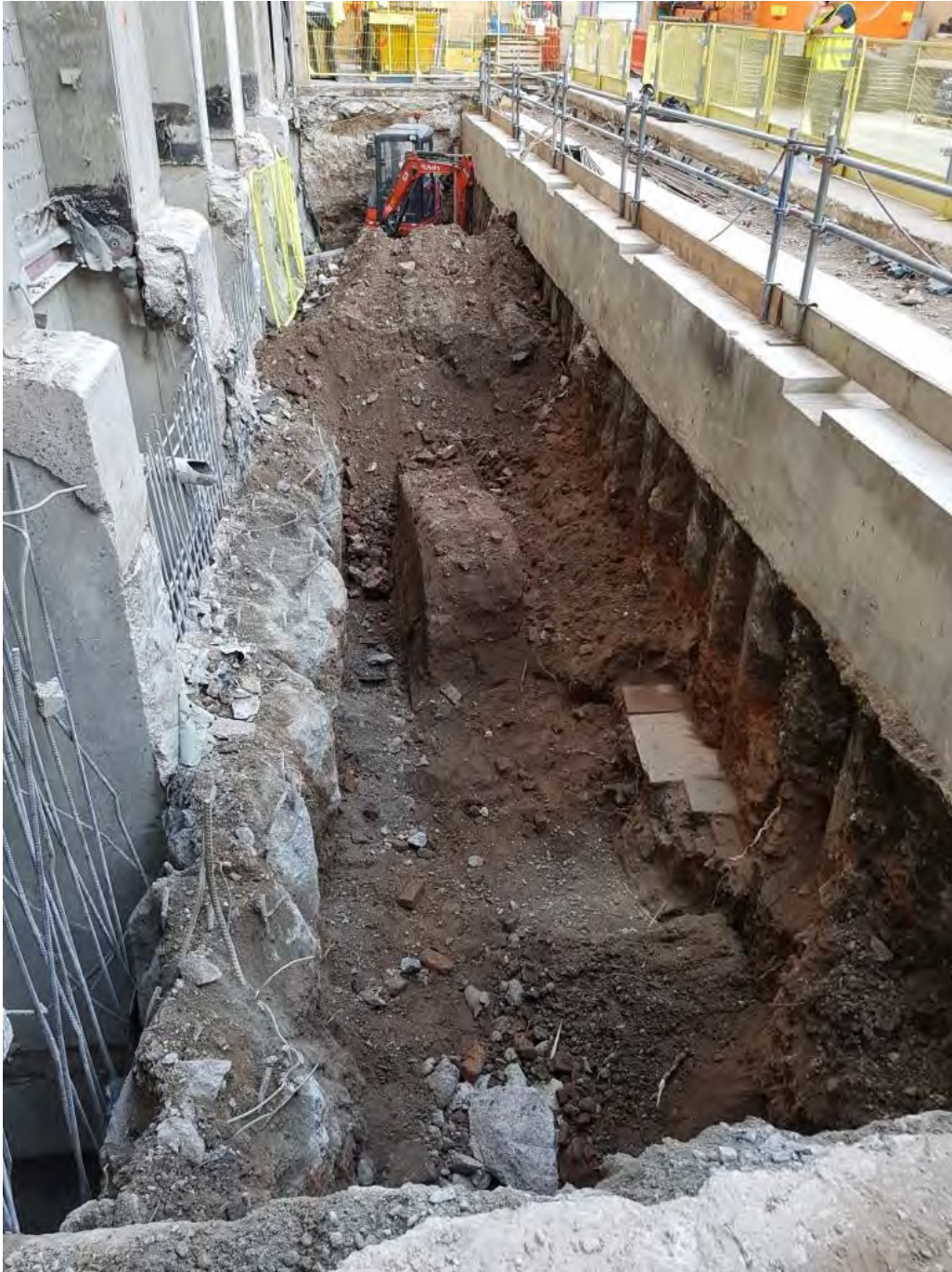
Overall view of the trench facing north. The 1990's secant pile wall is evident to the left; the remains of the large early 19th century brick wall can be seen in centre of the photograph
