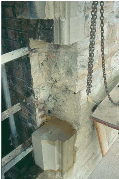
FIGURE 11: View of conservation works to the east opening on the second floor, showing the construction of the 1901 – 1903 walls.
