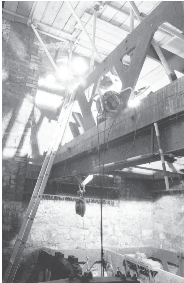
Figure 10a: The Independent Two Tier Cast Iron Bell Frame Second Floor
