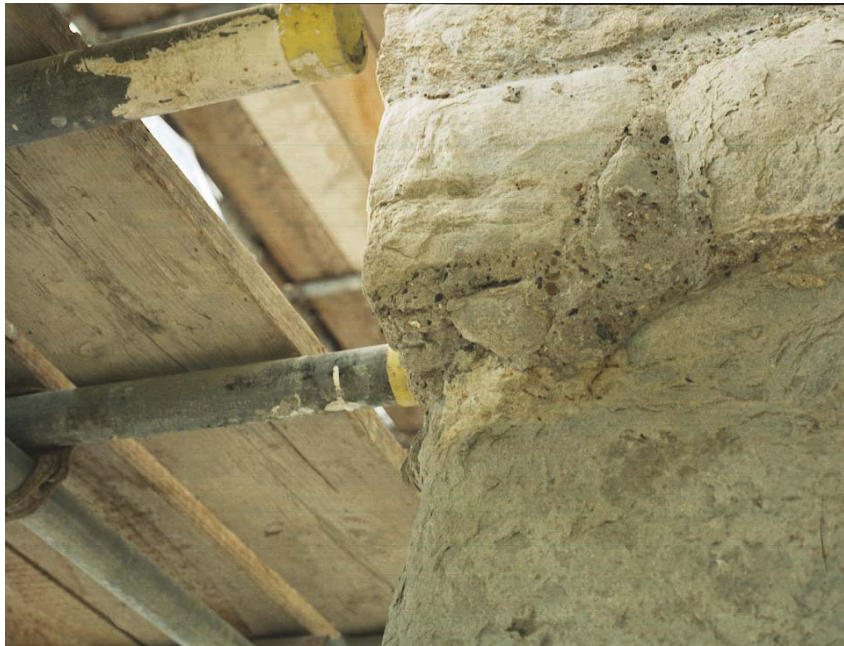
FIGURE 15: View of the southeast buttress showing the Kentish ragstone set in Portland cement-based mortar
