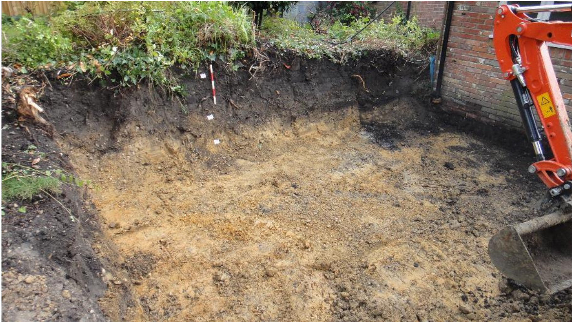
Plate 3. General shot of trench excavated to finished depth, looking northeast. Scale: 1 x 0.5m.
