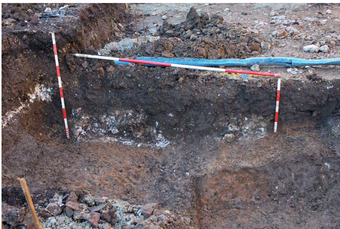
Plate 2 North facing section, showing walls [008] and [009], truncated by [011] (same as depicted in Figure 4)
