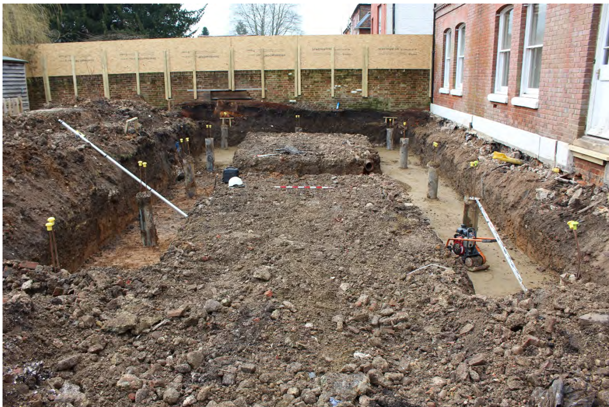
Plate 5 View to the south of the area monitored during the watching brief
