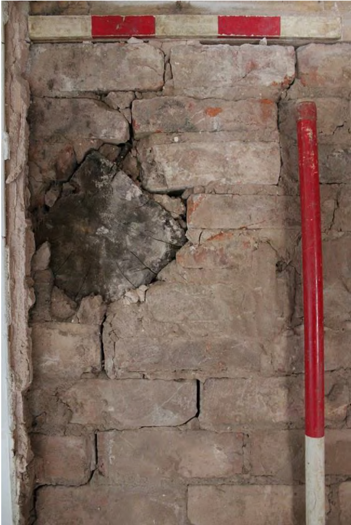
Plate 90: Detail of timber in north-west wall of Staff Room following removal of the south-west wall, looking north-west (LMSC16 D103 (35))
