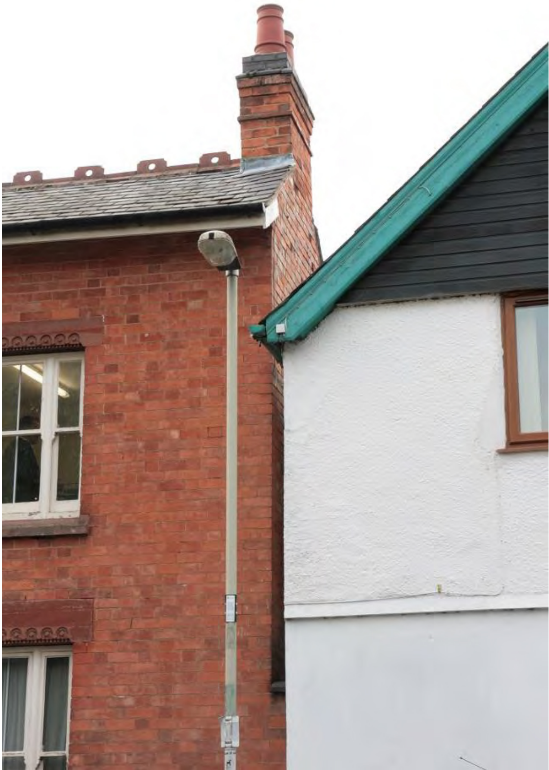
Plate 8: Chimneystack at north-east end of Cosby Pharmacy, looking up and north-west (LMSC16 D100 (17))
