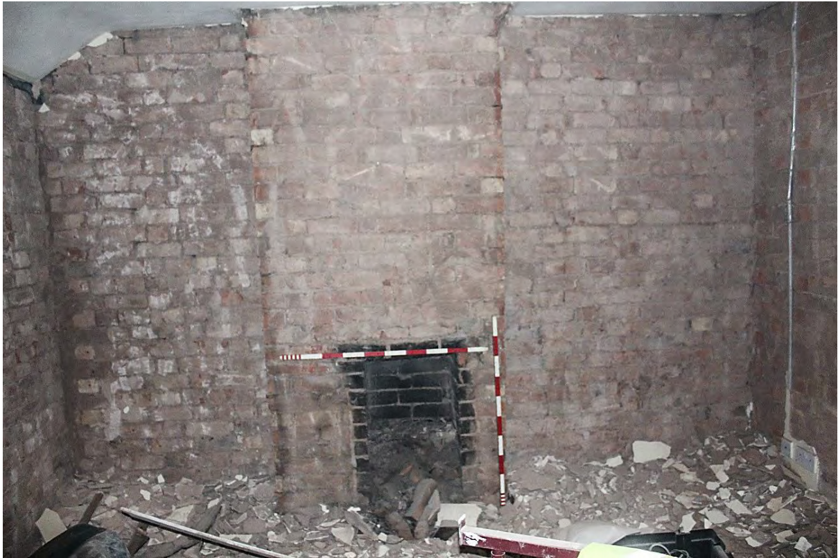
Plate 85: North-east wall of Staff Room following soft strip, looking north (LMSC16 D102 (4))
