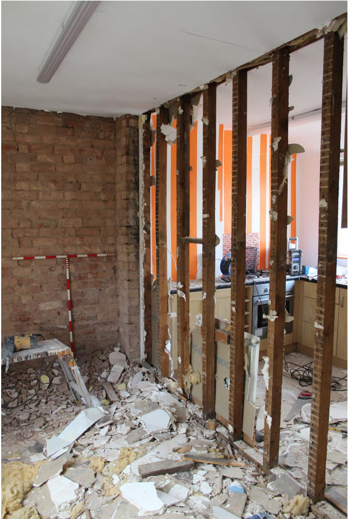
Plate 70: Chimney breast in the west corner of the First Floor Store Room, looking west (LMSC16 D101 (6))
