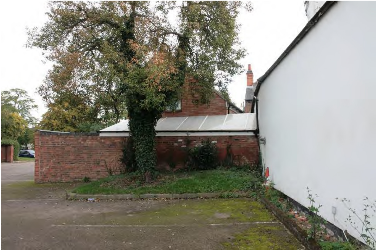
Plate 20: North-east end of the north-west (rear) elevation in relation to nearby properties, looking south-east (LMSC16 D100 (117))
