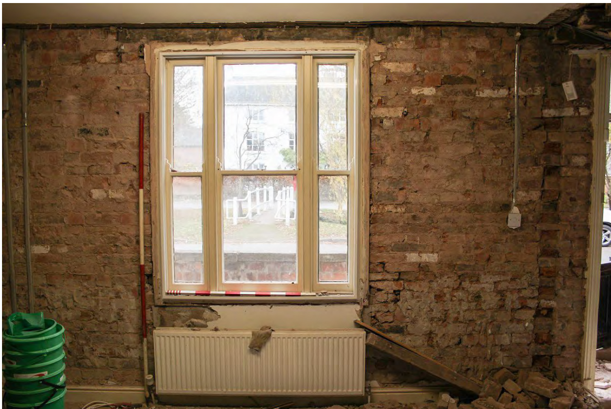
Plate 58: South-east wall of Staff/Store Area following soft strip, looking south-east (LMSC16 D103 (4))
