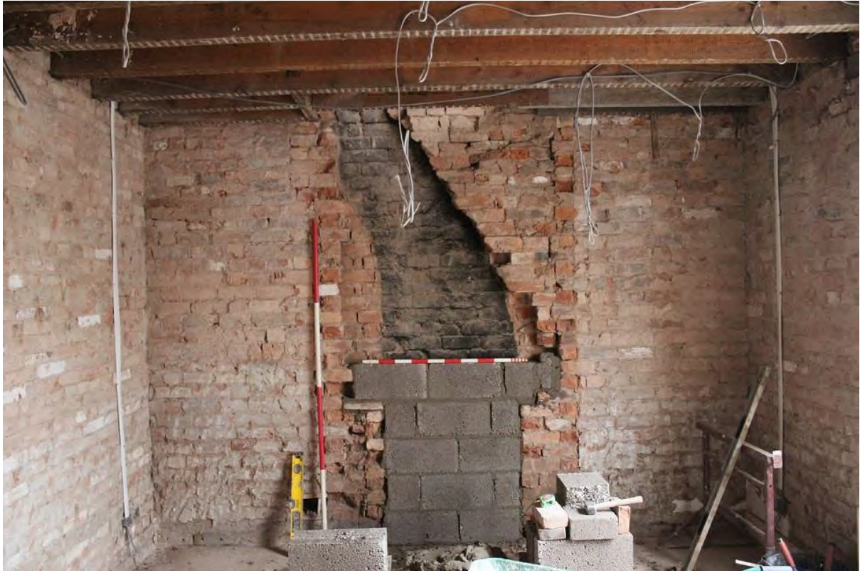
Plate 56: North-east wall of Staff/Store Area following removal of the chimney breast, looking north-east (LMSC16 D104 (4))
