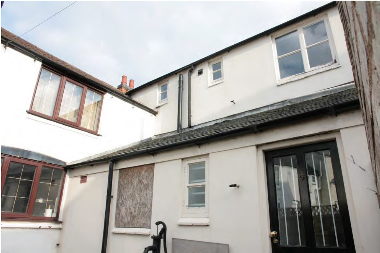
Plate 15: North-west (rear) elevation in relation to no. 69 Main Street (left), looking up and east (LMSC16 D100 (124))
