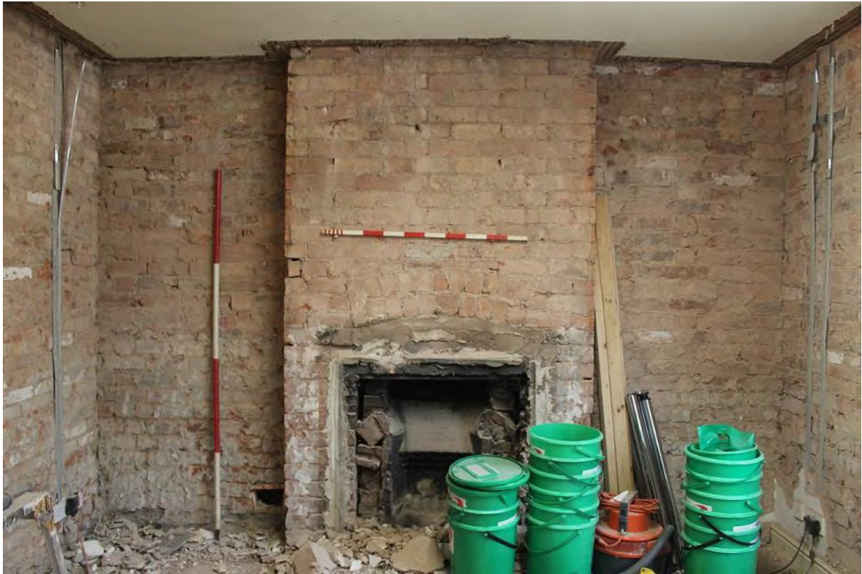
Plate 55: North-east wall of Staff/Store Area following soft strip, looking north-east (LMSC16 D103 (2))
