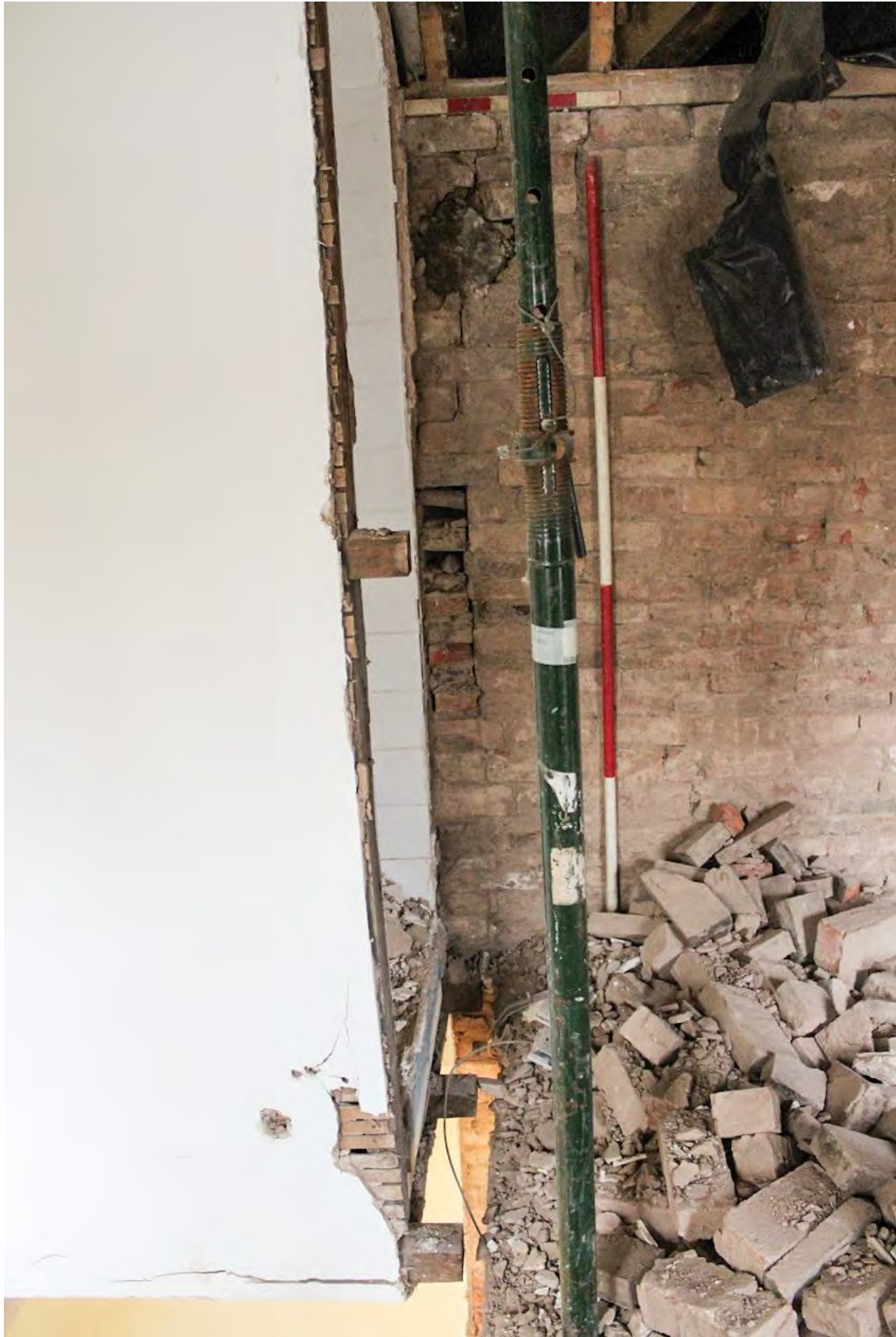
Plate 89: North-west wall of Staff Room following removal of the south-west wall, looking north-west (LMSC16 D103 (32))
