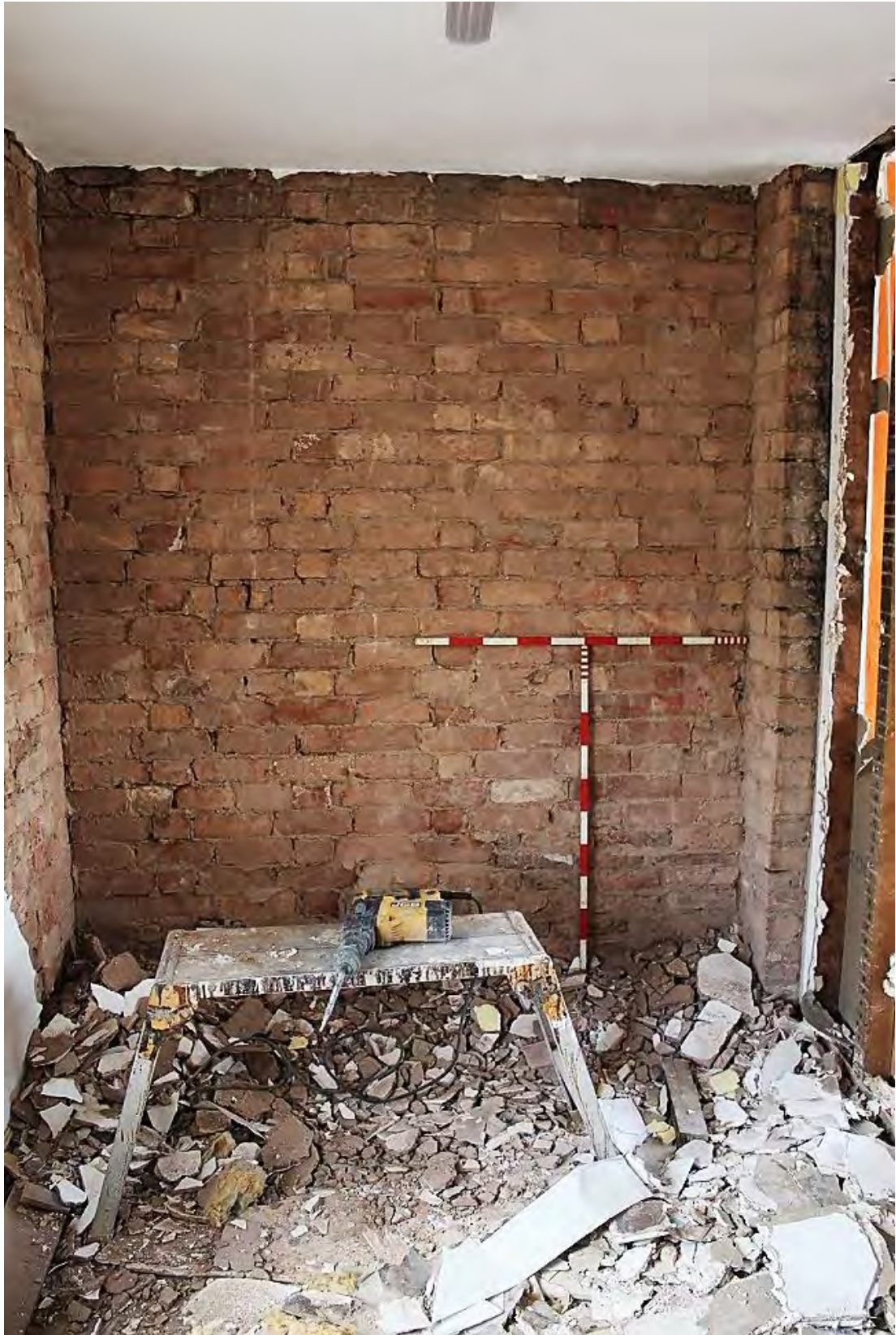
Plate 69: Chimney breast in the west corner of the First Floor Store Room, looking west (LMSC16 D101 (4))
