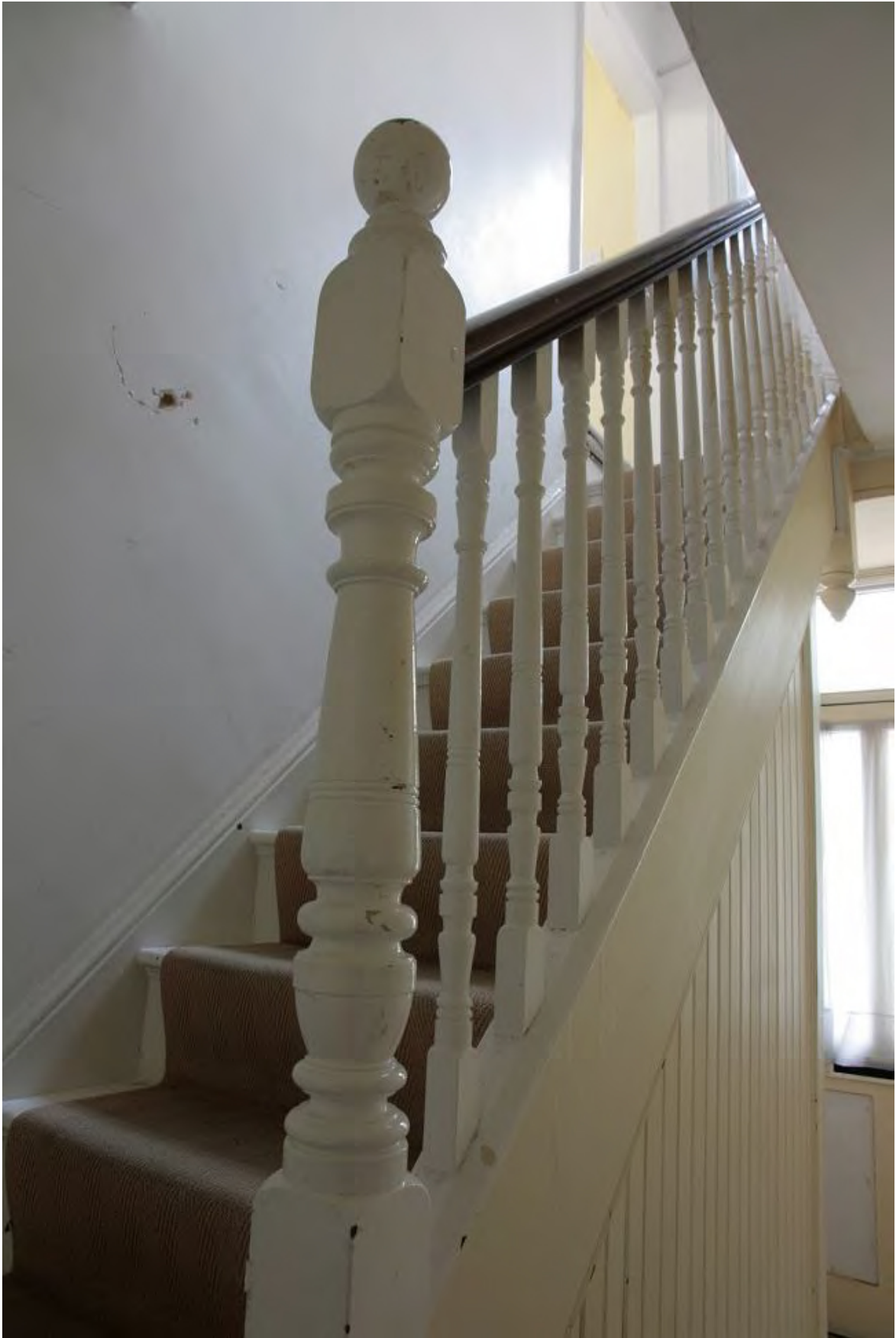
Plate 61: Newel post and balustrade of stairs to first floor, looking east-southeast (LMSC16 D100 (70))
