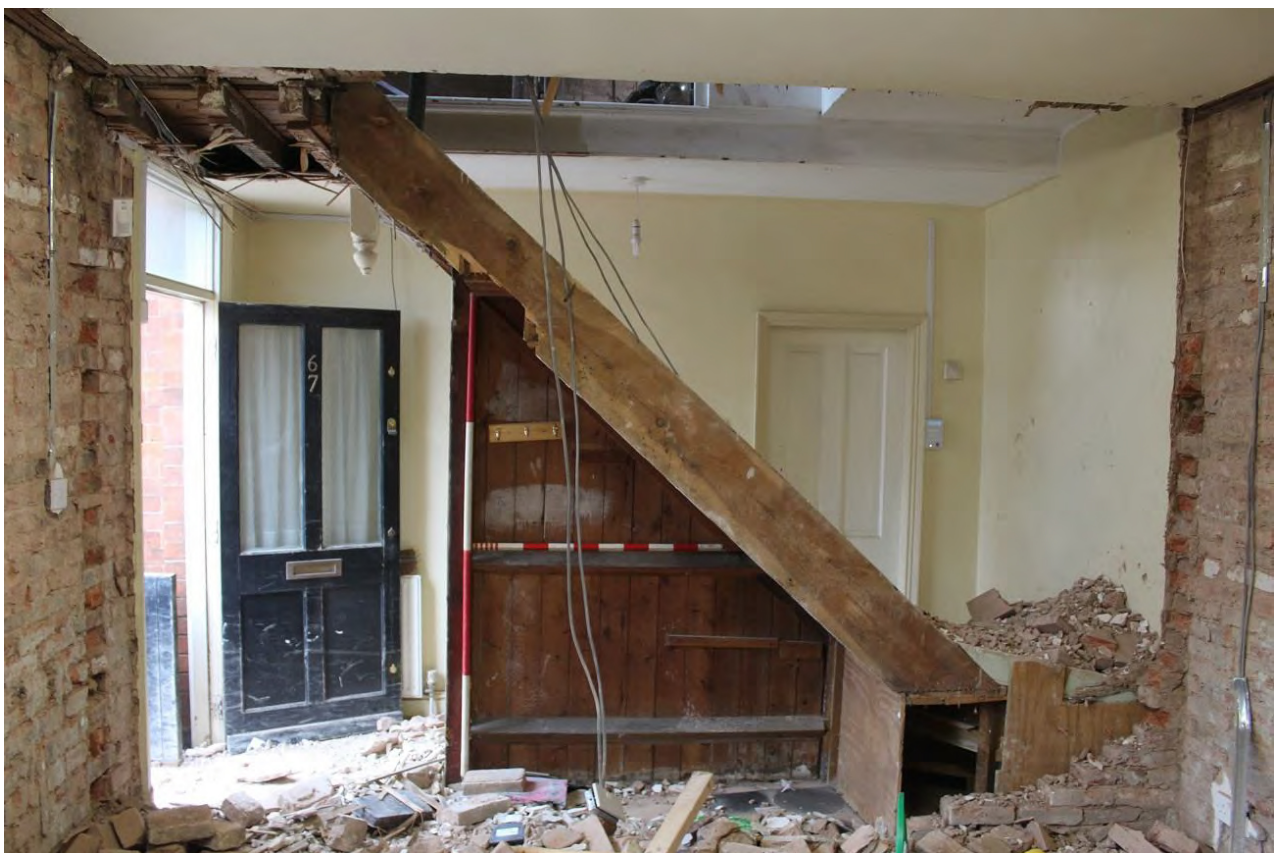
Plate 60: South-west wall of Staff/Store Area following soft strip, looking south (LMSC16 D103 (7))
