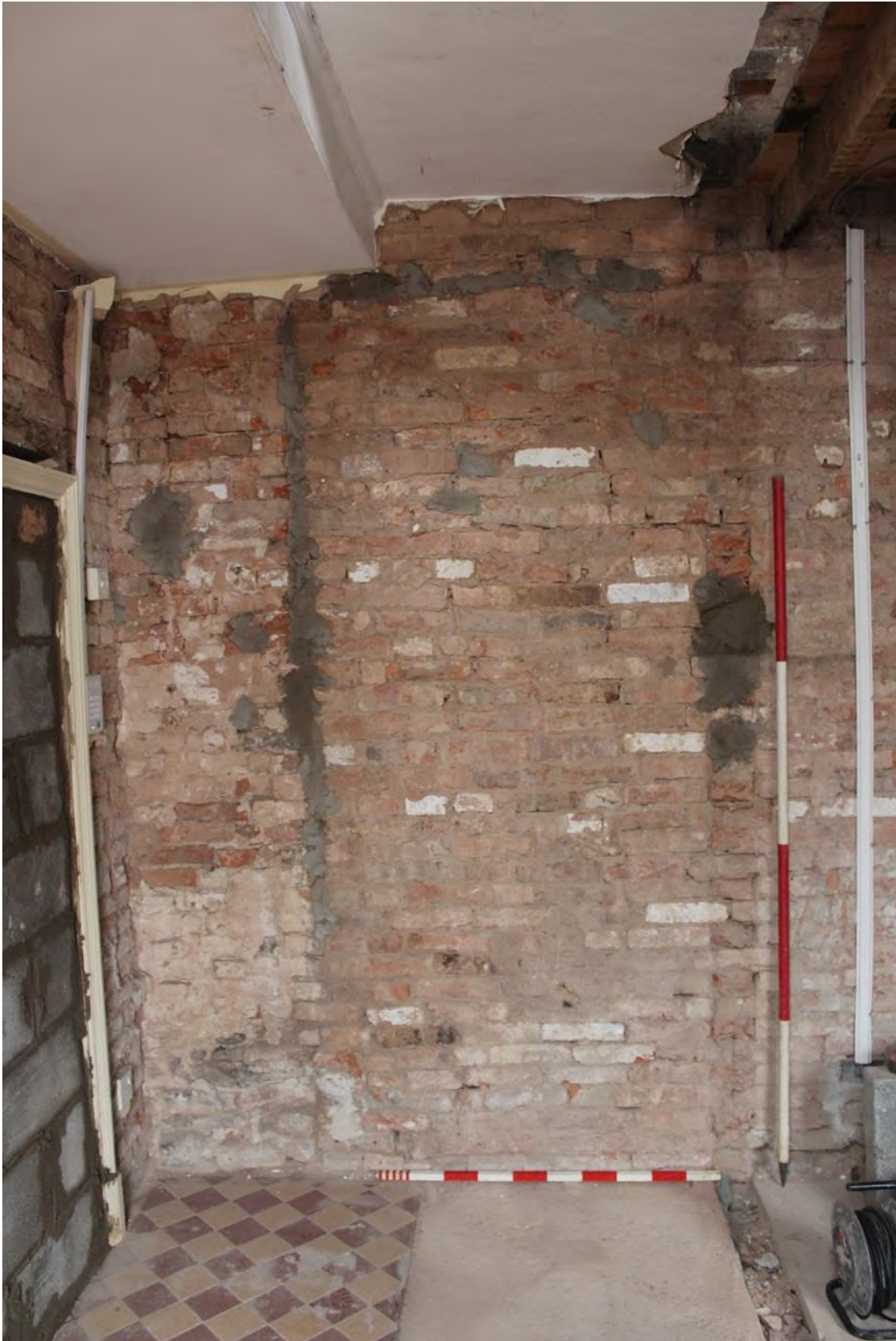
Plate 48: Entrance Lobby following soft strip, removal of the staircase (faint scar) and removal of the south-west wall of the Staff/Store Area (scar on right hand side), looking north-west (LMSC16 D104 (7))
